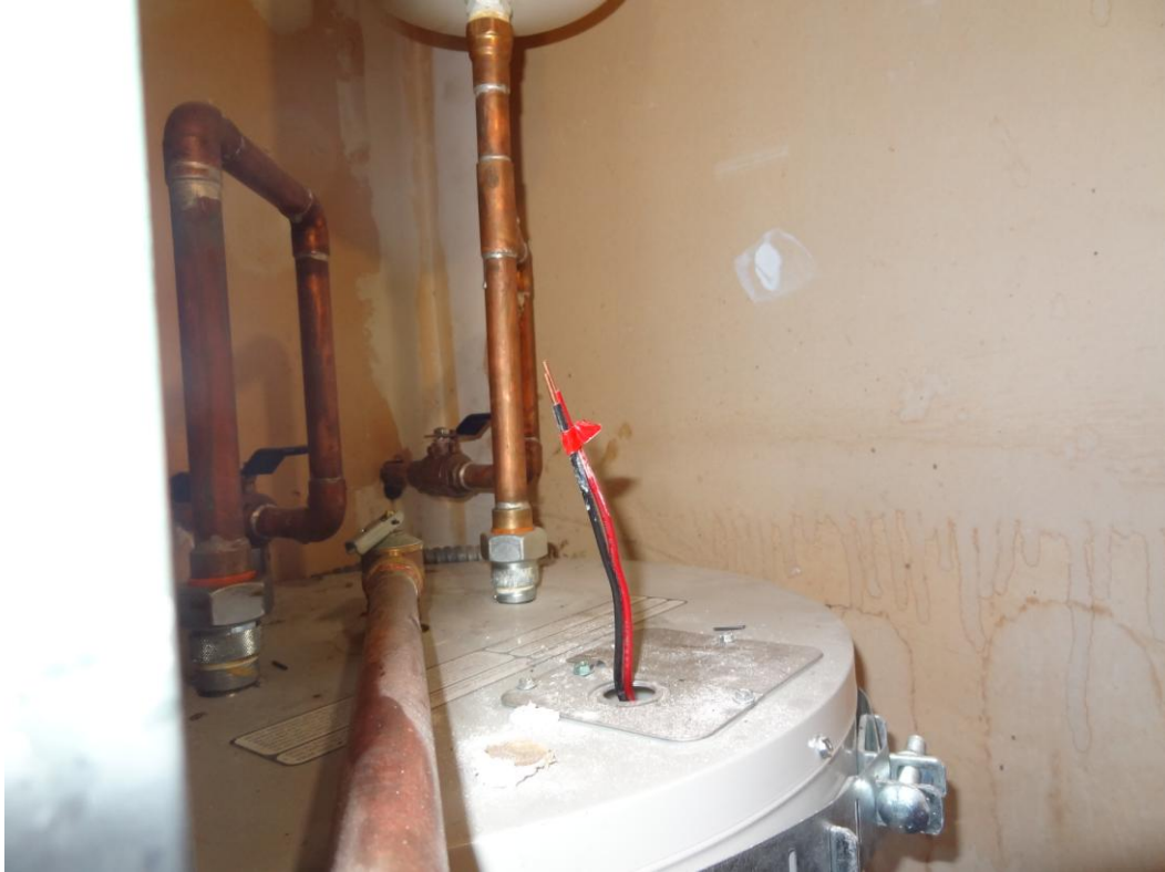
Winnemucca Office Building – Winnemucca Site – FCA Building #2433 Description: Water Heater electrical not connected.
