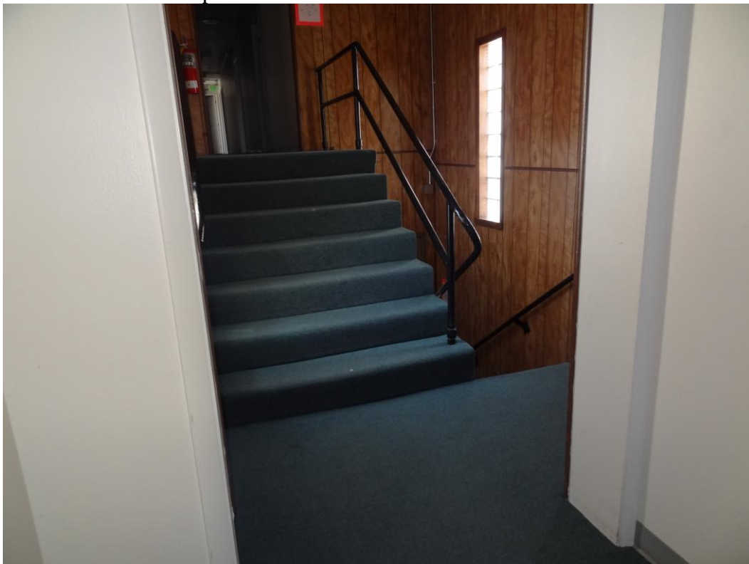
Winnemucca Office Building – Winnemucca Site – FCA Building #2433 Description: Non-compliant interior handrails.
