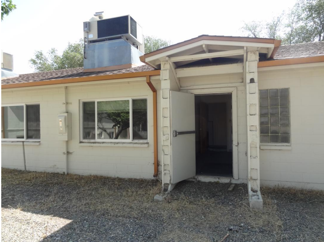
Winnemucca Office Building – Winnemucca Site – FCA Building #2433 Description: Missing exterior landing.
