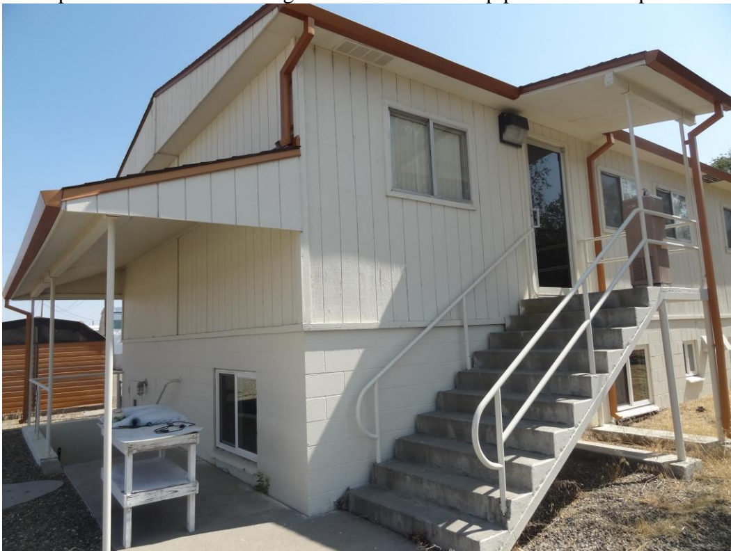
Winnemucca Office Building – Winnemucca Site – FCA Building #2433 Description: Non-compliant exterior handrails.
