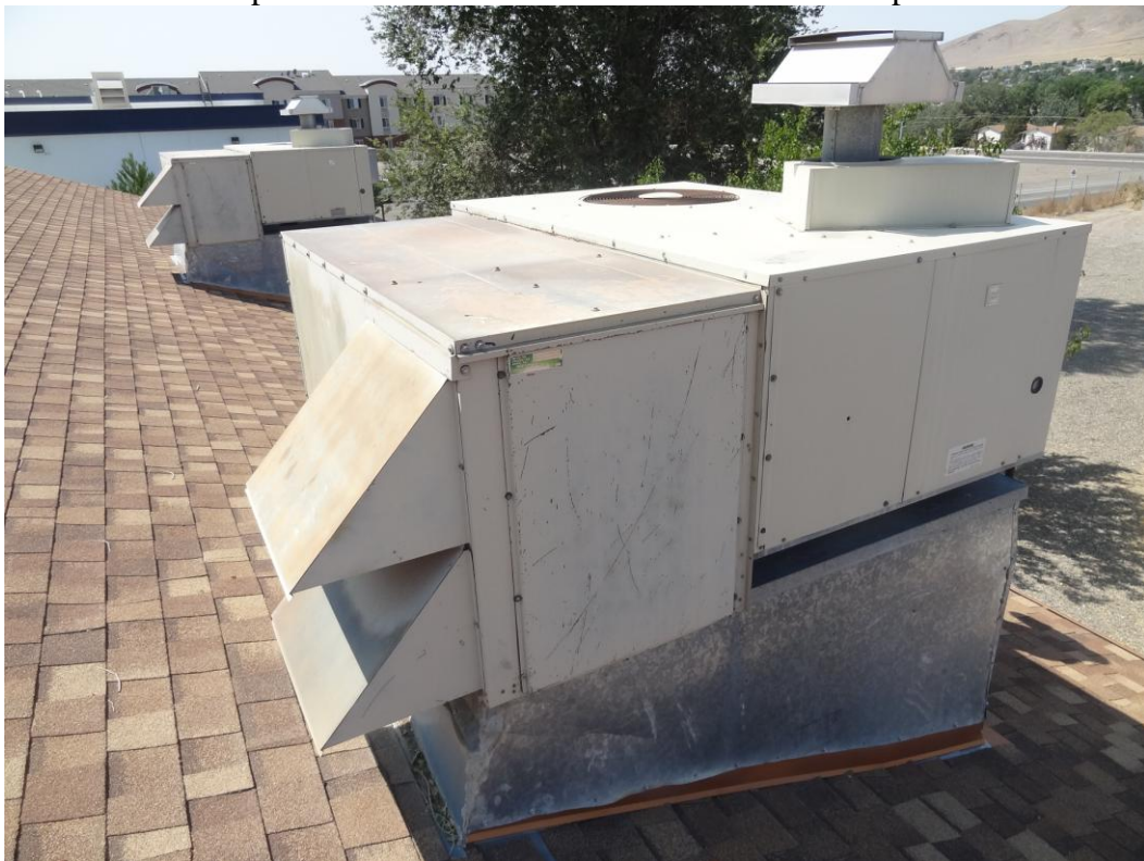
Winnemucca Office Building – Winnemucca Site – FCA Building #2433 Description: HVAC rooftop units over 30 years old.
