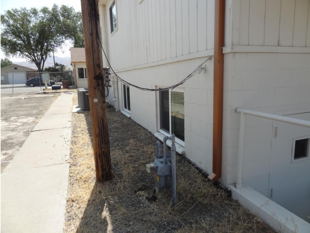
Winnemucca Office Building – Winnemucca Site – FCA Building #2433 Description: Gas service missing seismic shut-off and pipe bollards for protection.
