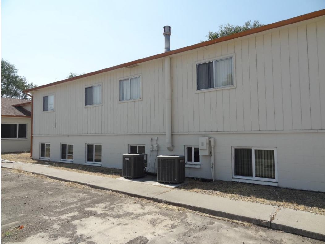
Winnemucca Office Building – Winnemucca Site – FCA Building #2433 Description: Second level windows have not been replaced.
