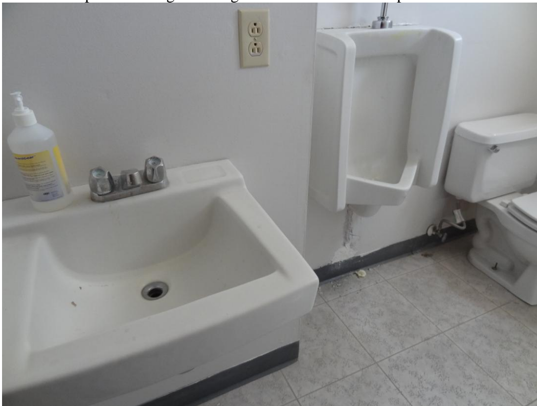
Winnemucca Office Building – Winnemucca Site – FCA Building #2433 Description: Restrooms due for a complete remodel.
