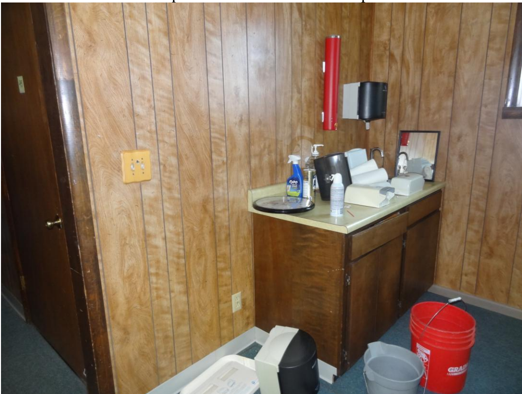
Winnemucca Office Building – Winnemucca Site – FCA Building #2433 Description: Kitchenette due for replacement.
