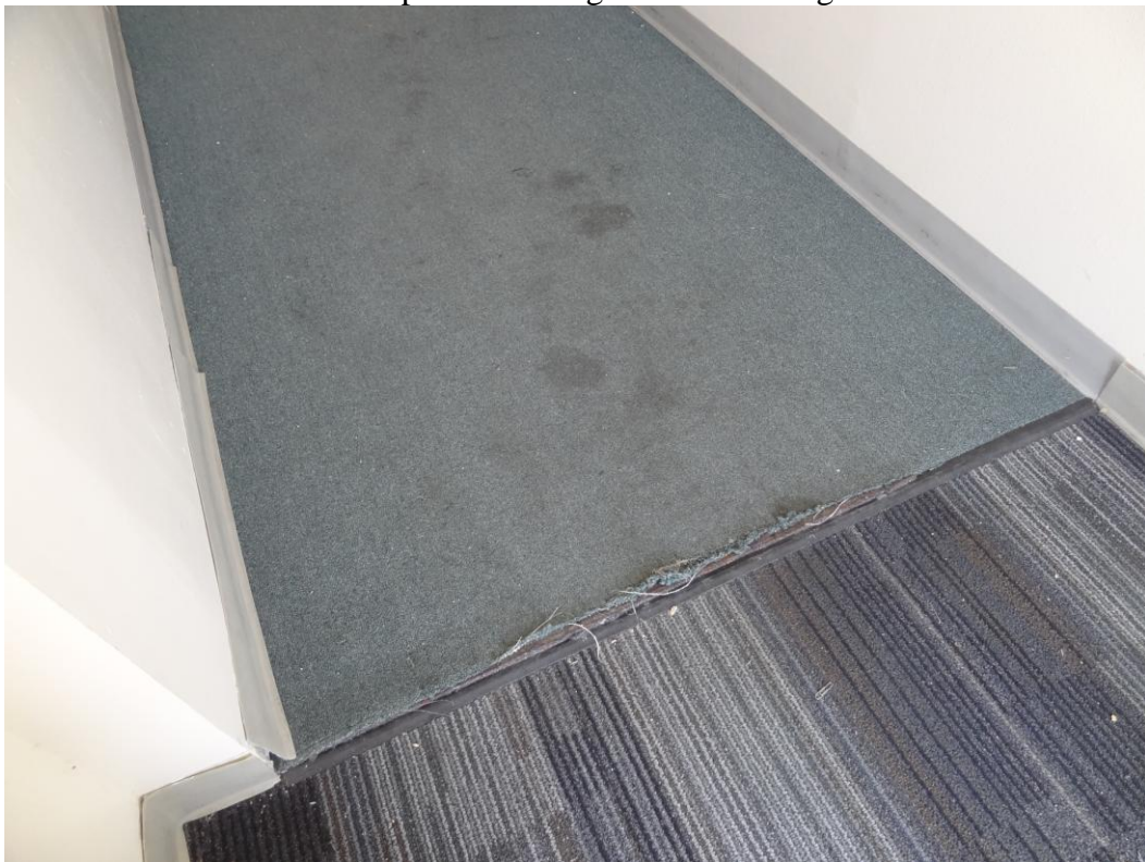
Winnemucca Office Building – Winnemucca Site – FCA Building #2433 Description: Stained and worn carpet.
