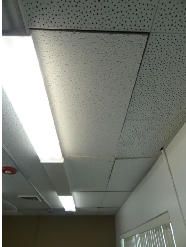
Winnemucca Office Building – Winnemucca Site – FCA Building #2433 Description: Damaged ceiling tile with mismatched replacement tiles.
