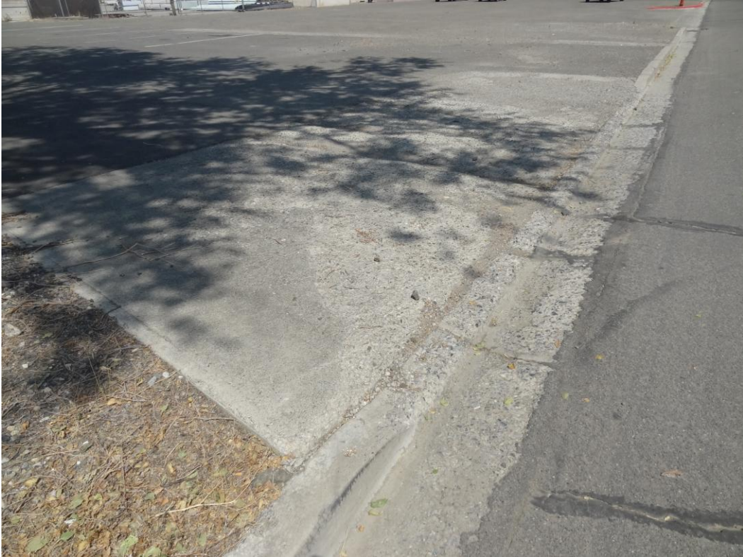
Winnemucca Office Building – Winnemucca Site – FCA Building #2433 Description: Deteriorated concrete apron.
