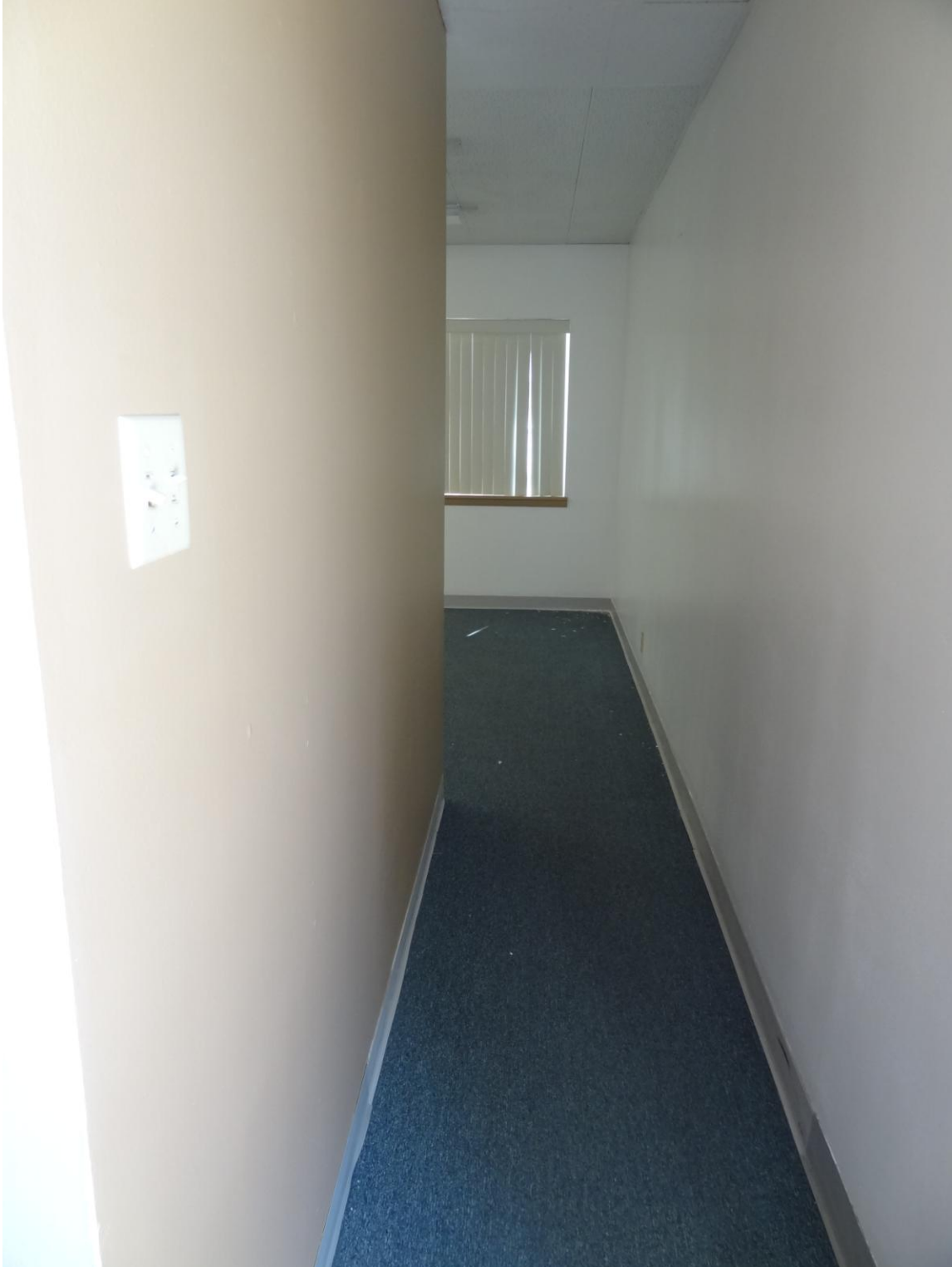
Winnemucca Office Building – Winnemucca Site – FCA Building #2433 Description: Non-compliant exit corridor from conference room.
