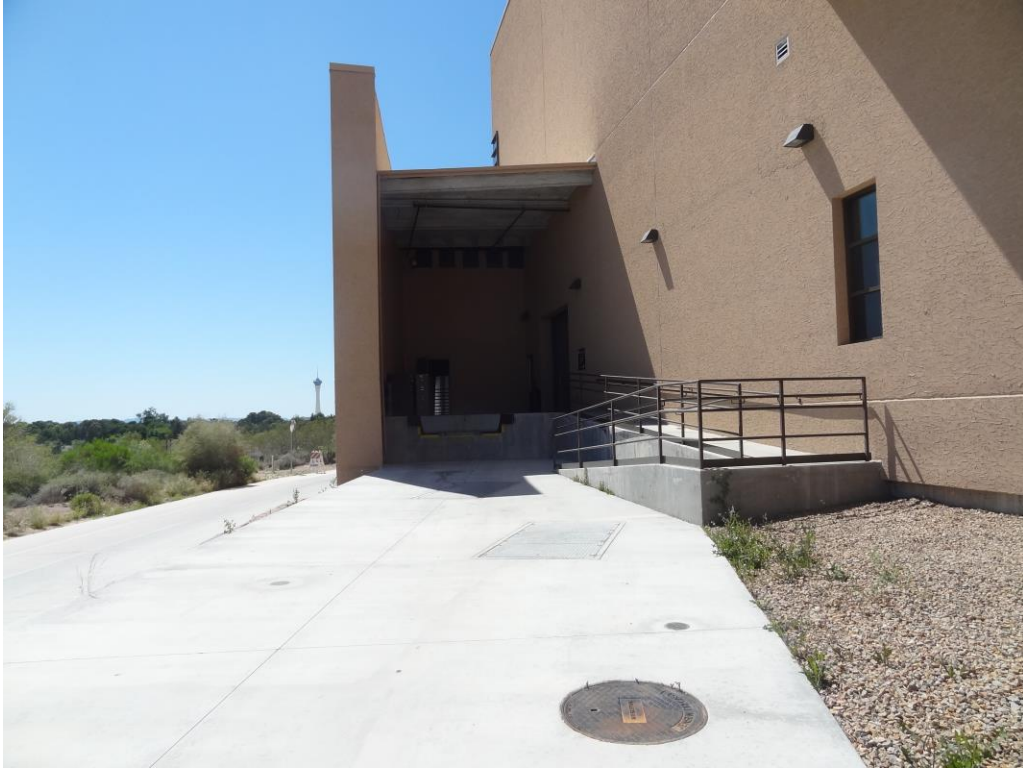
Nevada State Museum, LV - Building #2811 Description: Loading dock upgrades needed.
