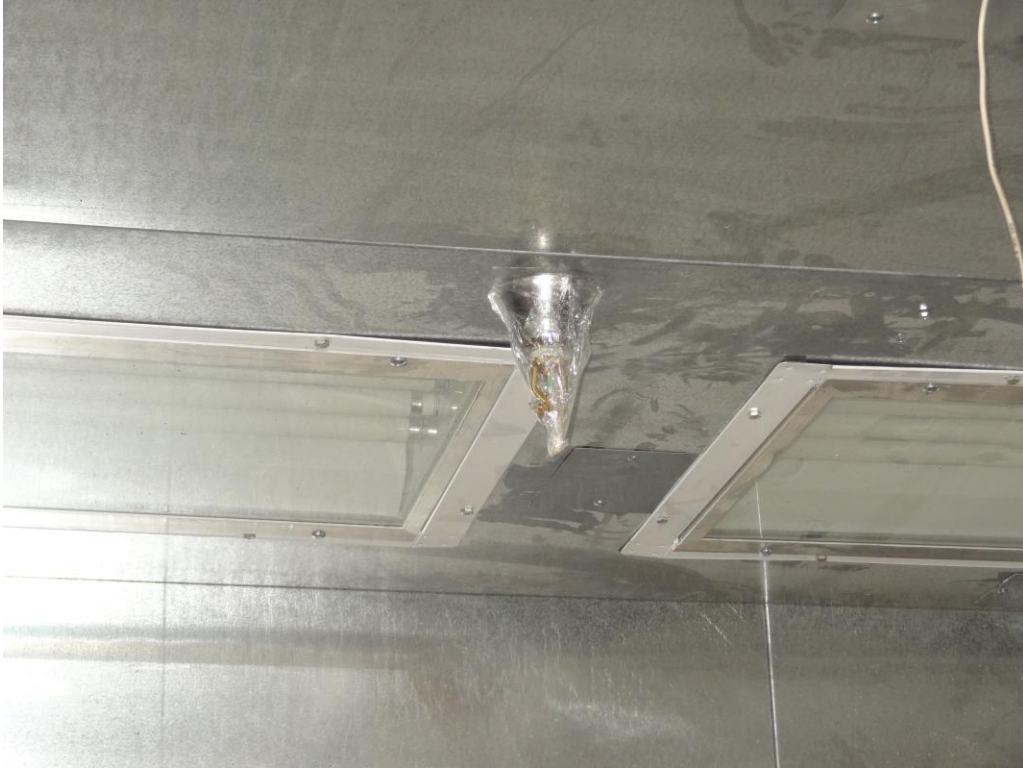
Nevada State Museum, LV - Building #2811 Description: Fire suppression/ mechanical upgrade needed.
