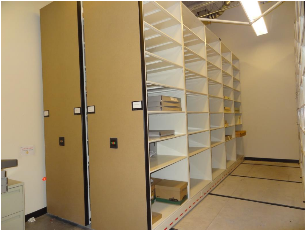
Nevada State Museum, LV - Building #2811 Description: High density storage repairs needed.
