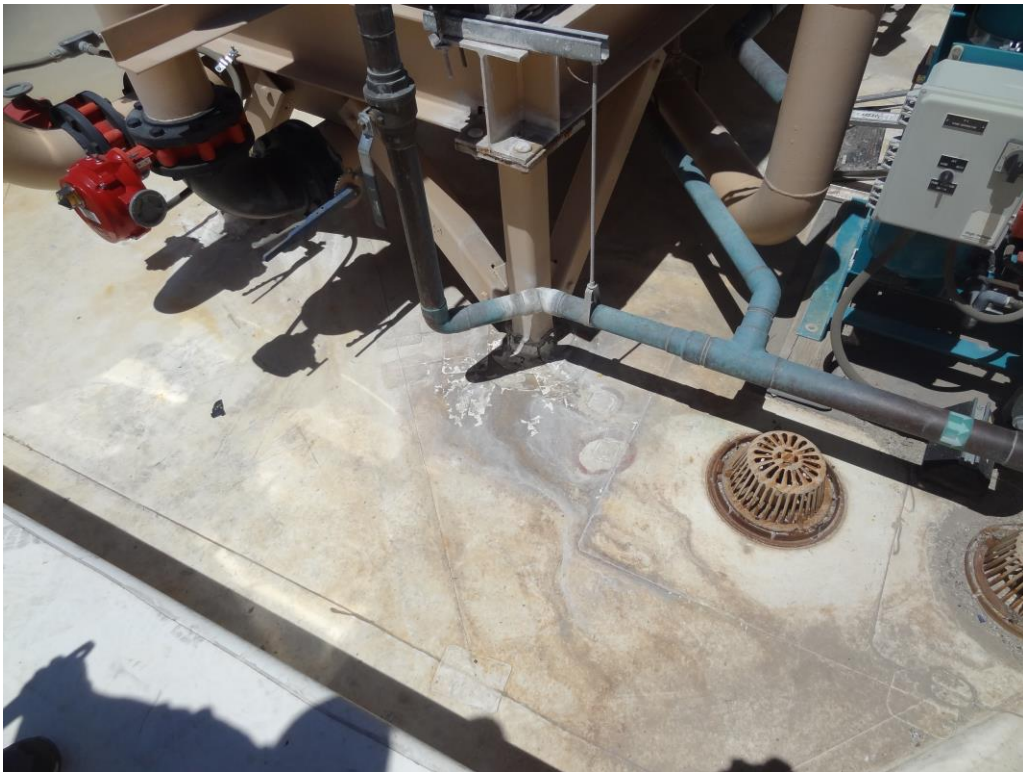
Nevada State Museum, LV - Building #2811 Description: Roof repairs needed.
