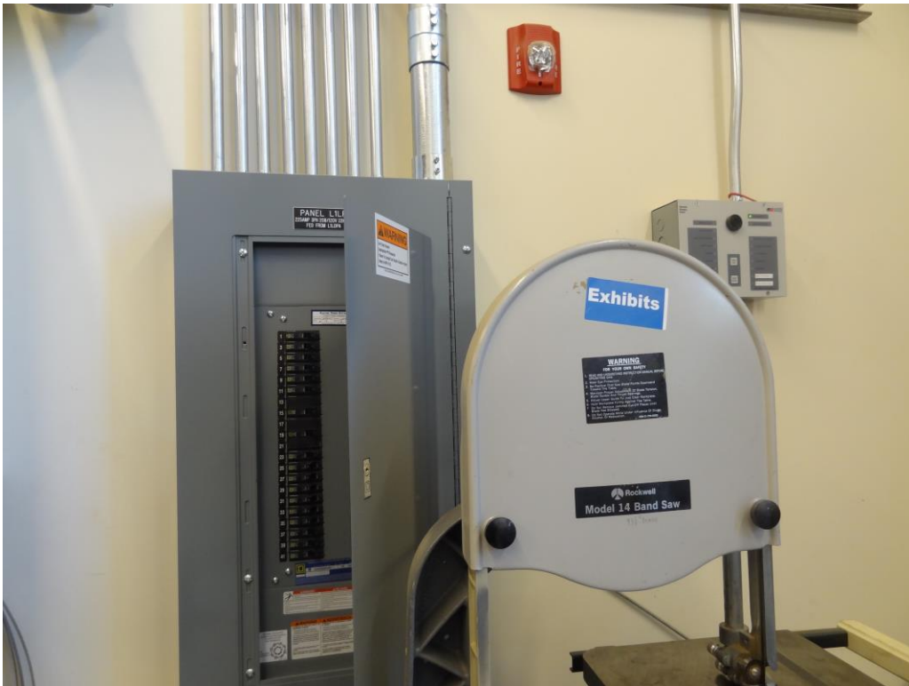
Nevada State Museum, LV - Building #2811 Description: Provide clearance at electrical panels.
