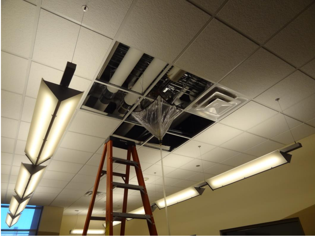
Nevada State Museum, LV - Building #2811 Description: Isolation valve installation needed.
