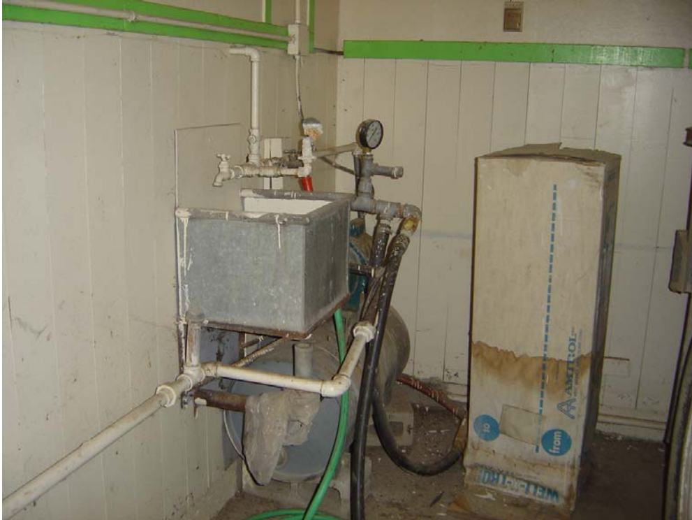
NDF Volunteer Fire Station - Building #0600 Description: Sink/Water service area.
