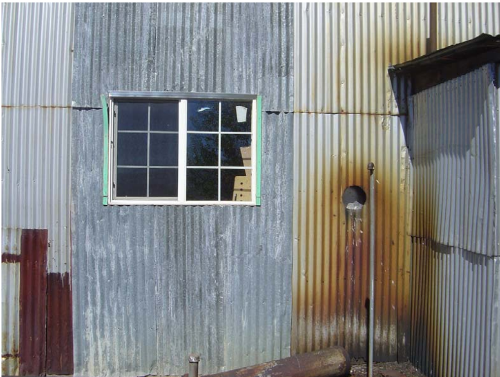
NDF Volunteer Fire Station - Building #0600 Description: Exterior view of damaged siding.
