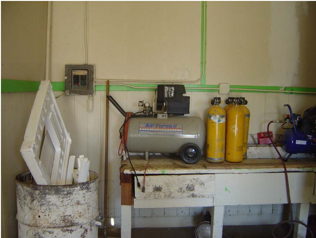
Division of Forestry, Deeth, Garage/Fire Station - Building #0600 Description: Workbench area, interior of building.
