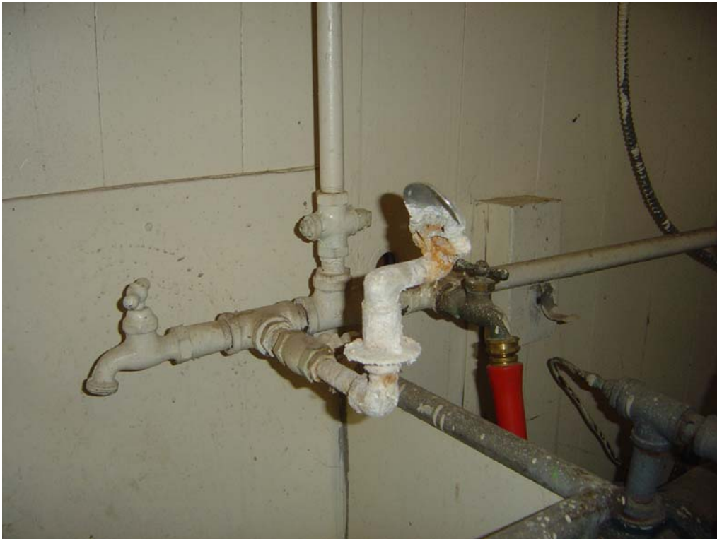
NDF Volunteer Fire Station - Building #0600 Description: Corroded drinking fountain.
