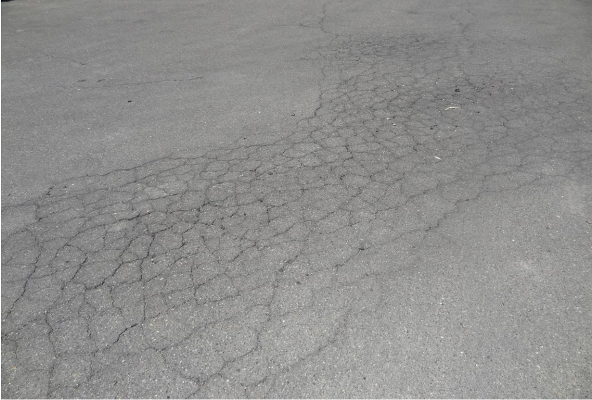
Elko Agriculture Office Site – FCA Site #9822 Description: AC paving in need of maintenance.
