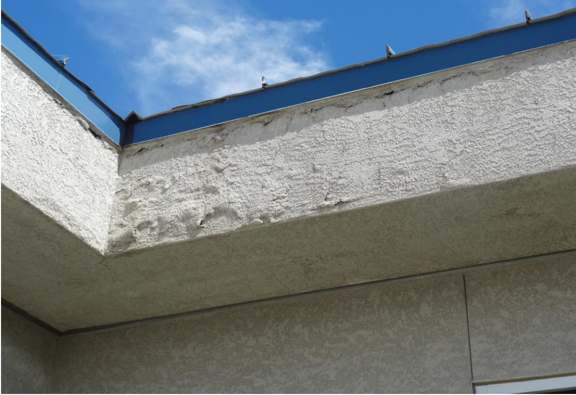
Elko Agriculture Regional Office – FCA Building #2558 Description: Stucco damage to the north side of the fascia.
