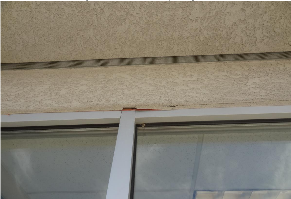
Elko Agriculture Regional Office – FCA Building #2558 Description: Window in need of caulking.
