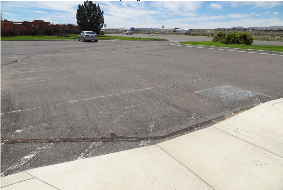
Elko Agriculture Office Site – FCA Site #9822 Description: ADA accessible parking area in need of striping.
