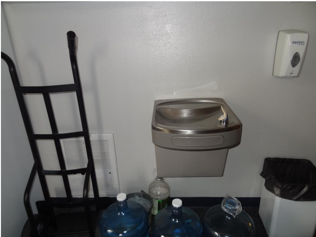
Elko DETR - Building #1476 Description: Dual level drinking fountain installation needed.
