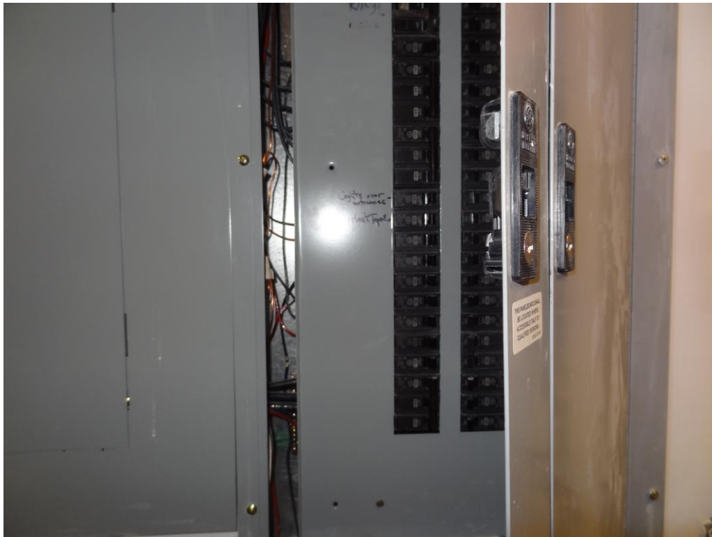
Elko DETR - Building #1476 Description: Electrical panel upgrades needed.
