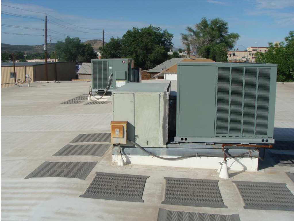
DETR Elko Office – Building #1476 Description: Roof top HVAC equipment.
