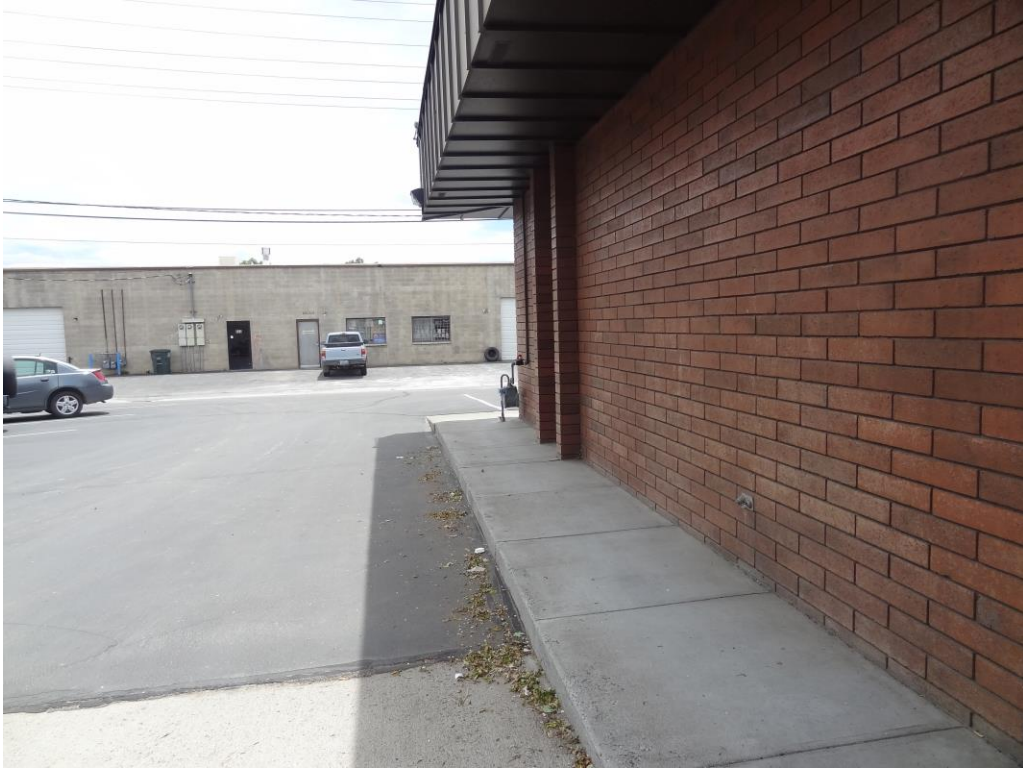
Elko DETR - Building #1476 Description: Exterior finishes needed.
