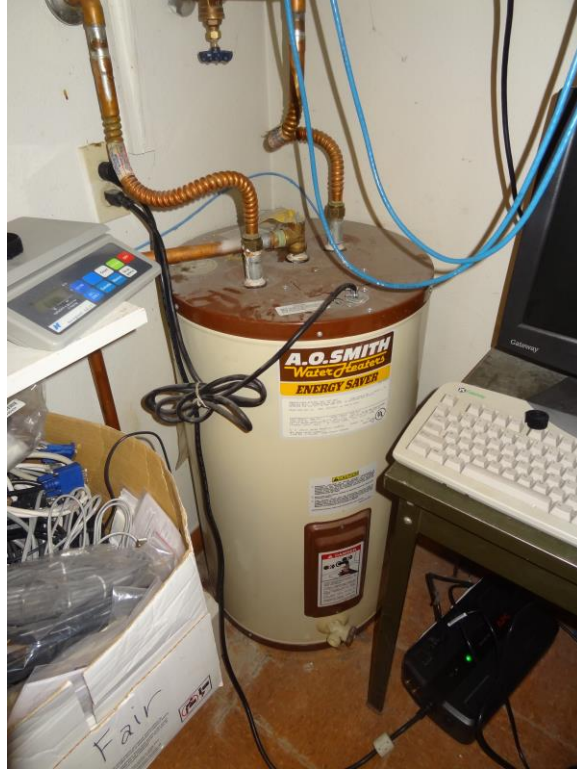
Elko DETR - Building #1476 Description: Water heater replacement needed.
