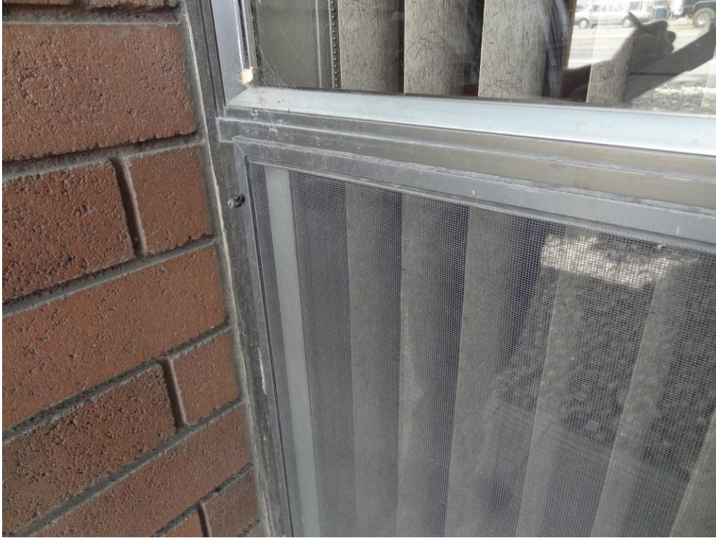
Elko DETR - Building #1476 Description: Window replacement needed.
