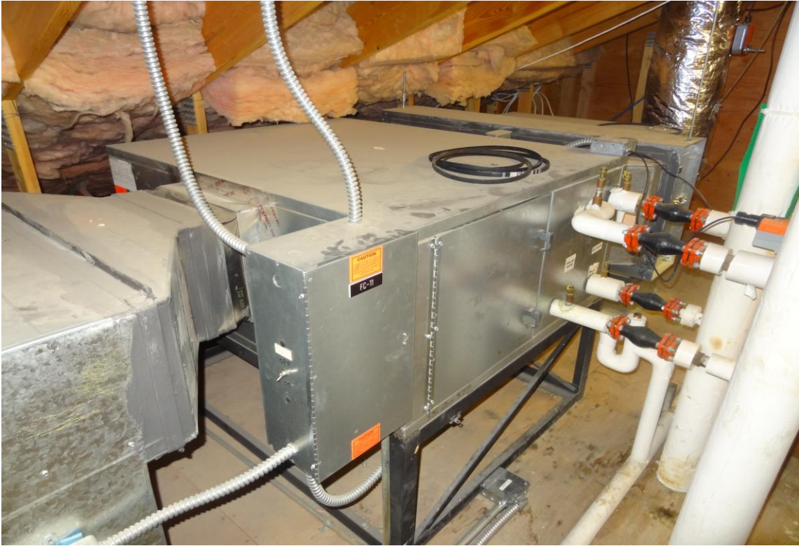
Elko Interagency Dispatch Center – FCA Building #2107 Description: Typical fan coil unit in attic.
