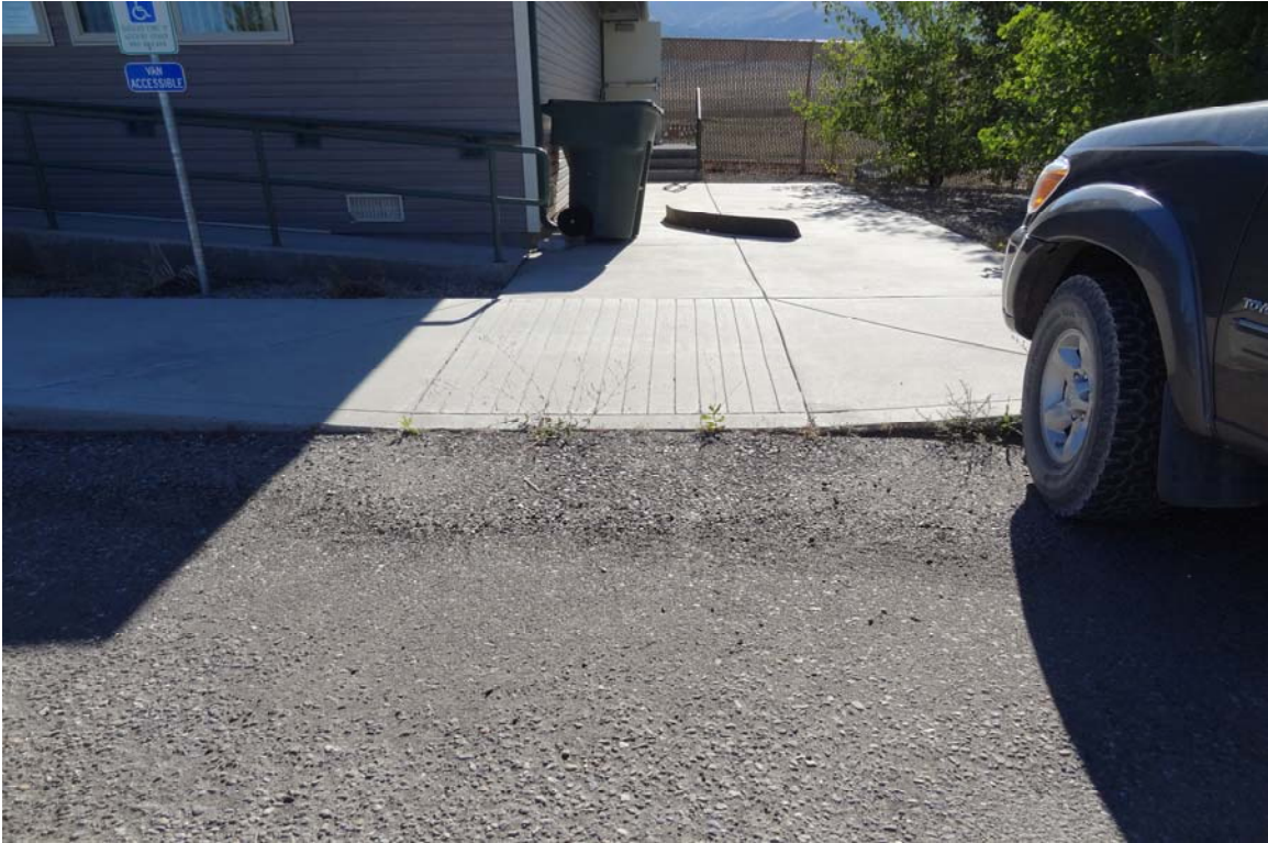
Ely Wildlife Field Office Site - Site #9825 Description: ADA parking area in need of striping.
