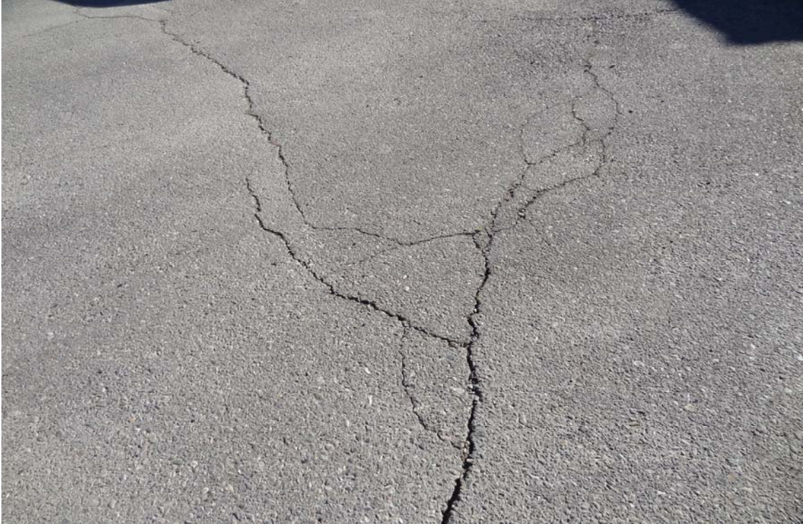
Ely Wildlife Field Office Site - Site #9825 Description: AC Paving in need of crack filling and seal coat.
