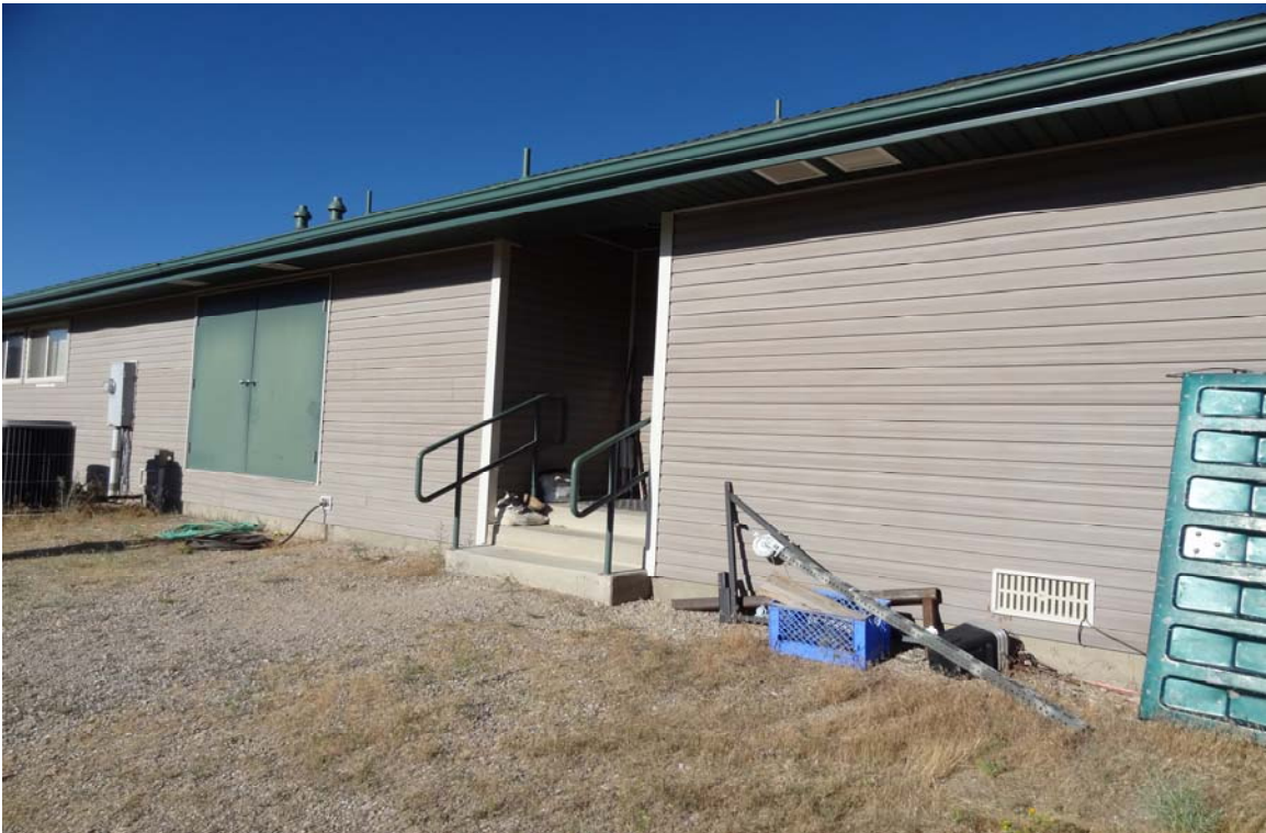
Ely Wildlife Field Office - Building #2127 Description: East elevation, note landing missing at stairs.
