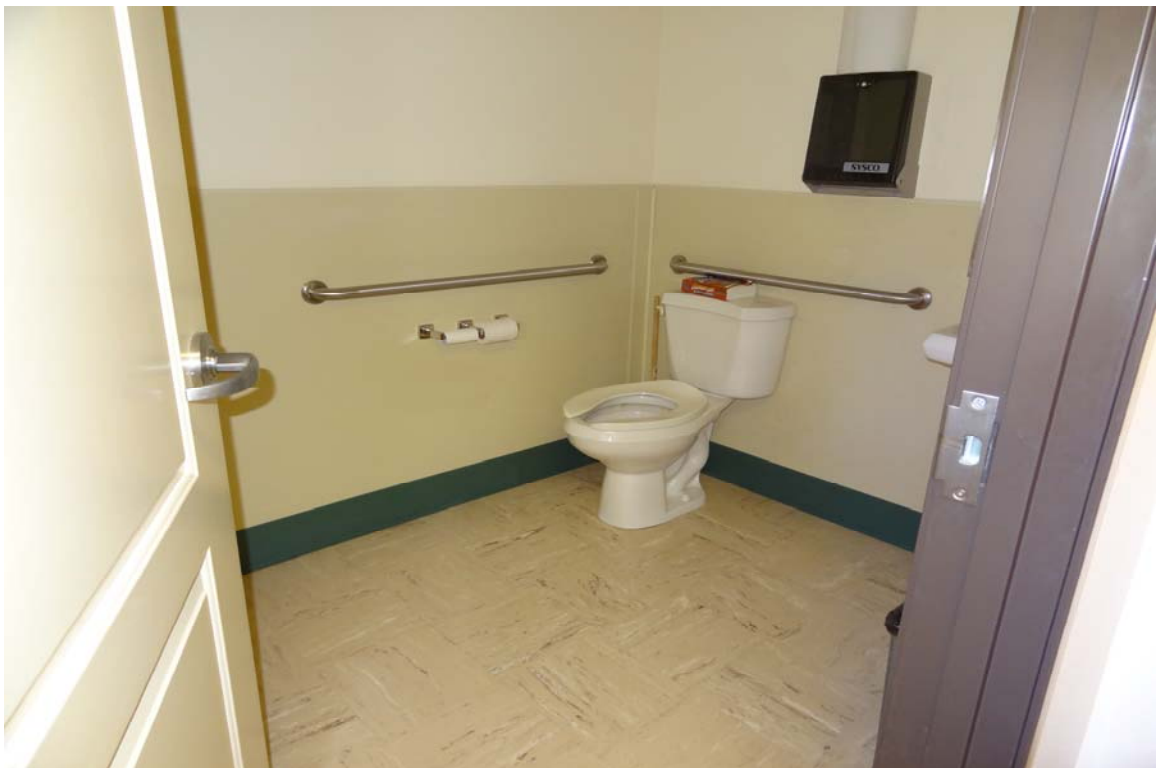
Ely Wildlife Field Office - Building #2127 Description: ADA restroom, note flush handle on wrong side.
