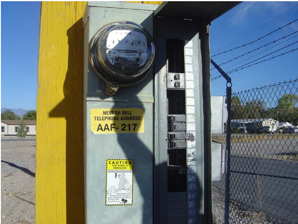
Indian Springs NHP Substation - Building #2462 Description: Electrical safety covers missing in main panel.
