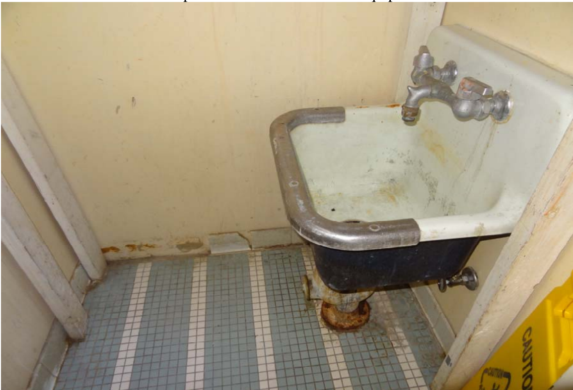
Belrose Office Building - Building #0286 Description: Janitor's closet in need of repairs.
