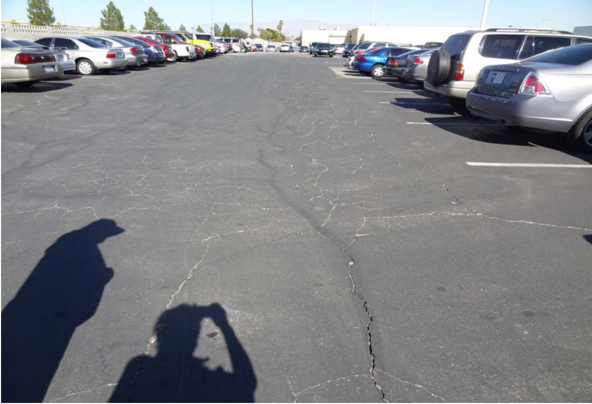
Belrose Office Building Site - Site #9831 Description: Damaged paving in parking area.
