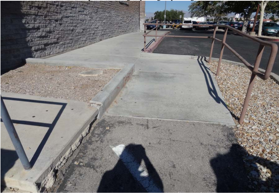
Belrose Office Building Site - Site #9831 Description: Non-ADA compliant route from bus stop to building.
