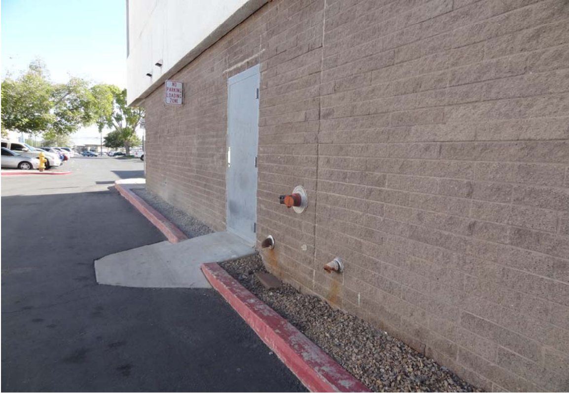
Belrose Office Building Site - Site #9831 Description: Non-code compliant landing at door.
