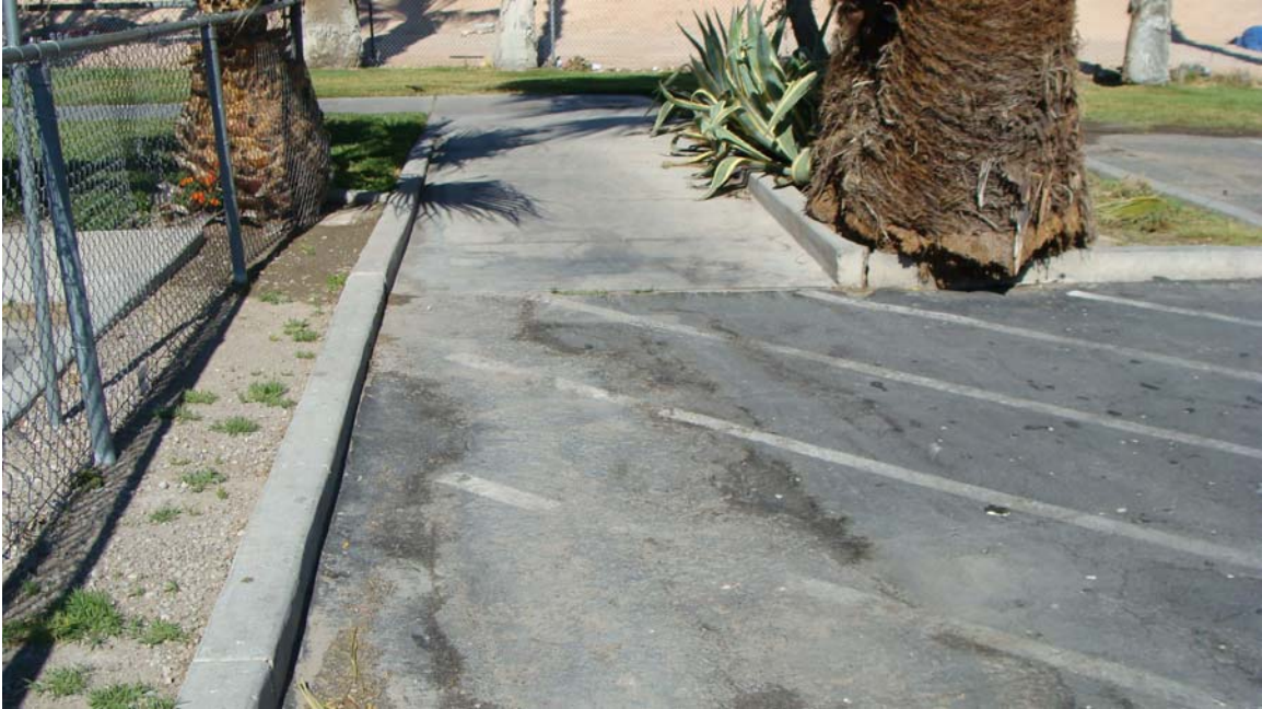
Las Vegas Casual Labor Office Site - Site #9833 Description: Tree causing damage to curb.
