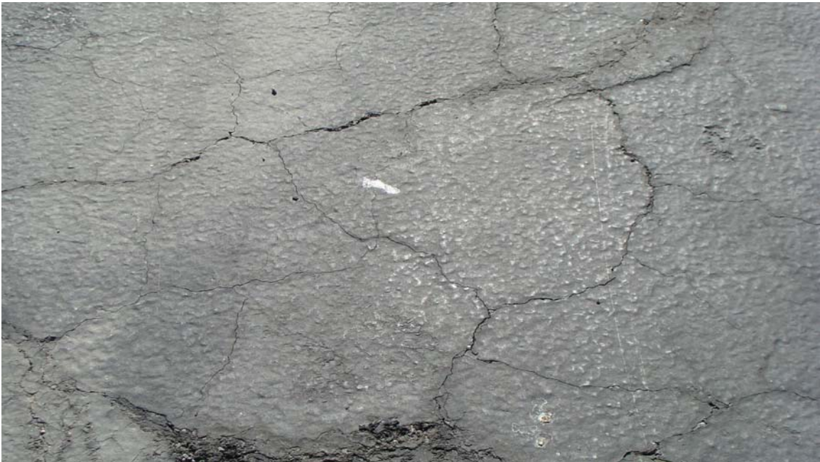
Las Vegas Casual Labor Office Site - Site #9833 Description: Asphalt paving in need of crack fill and slurry.
