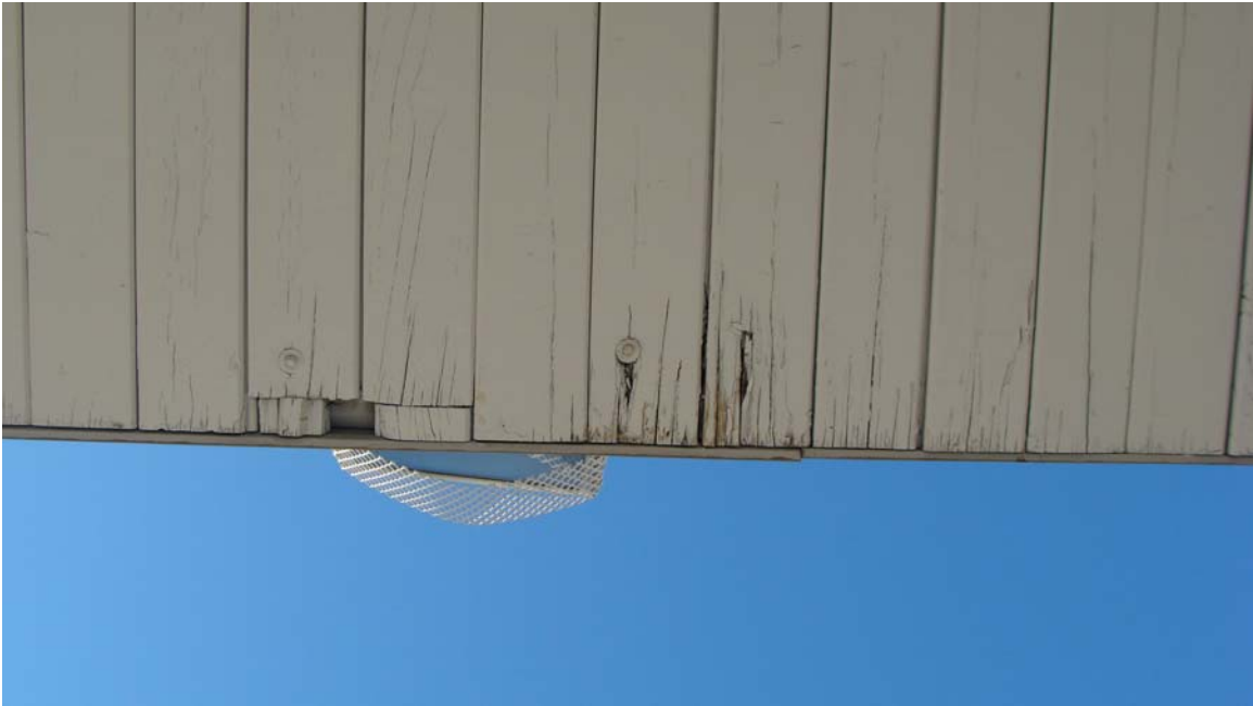
Las Vegas Casual Labor Office Site - Site #9833 Description: Soffit damage.
