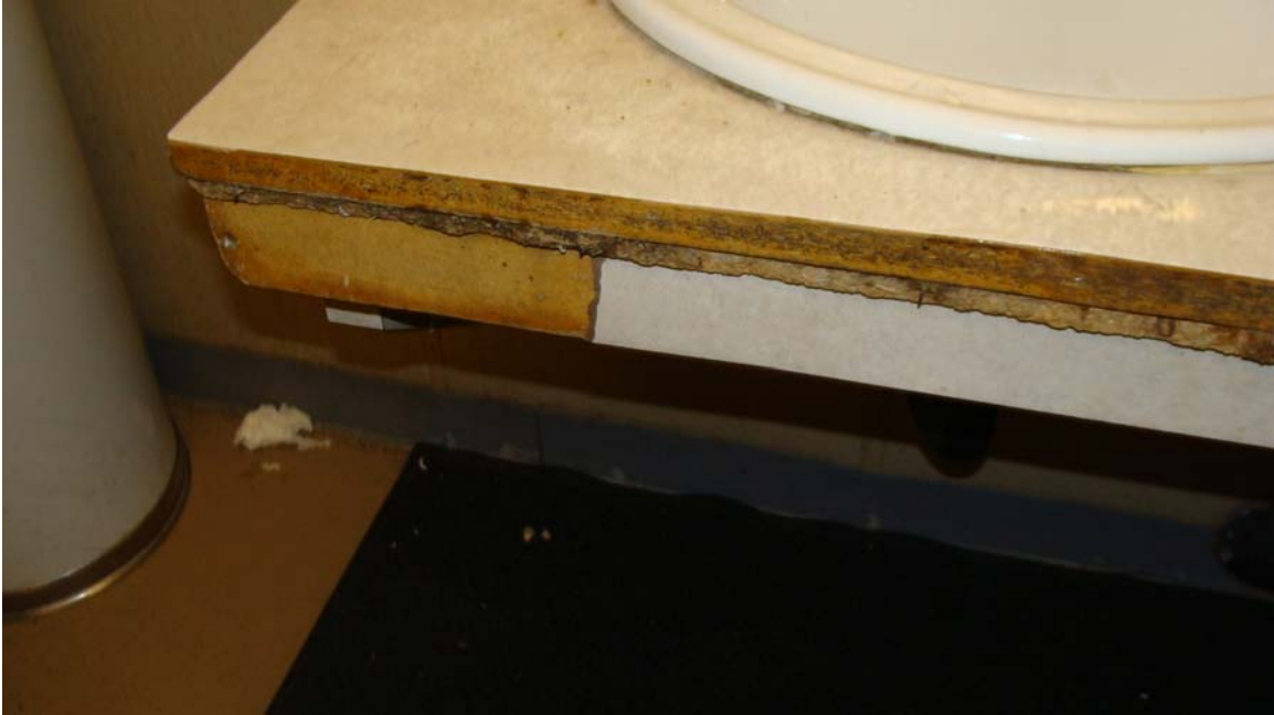
Las Vegas Casual Labor Office Site - Site #9833 Description: Damaged countertop in day room restroom.
