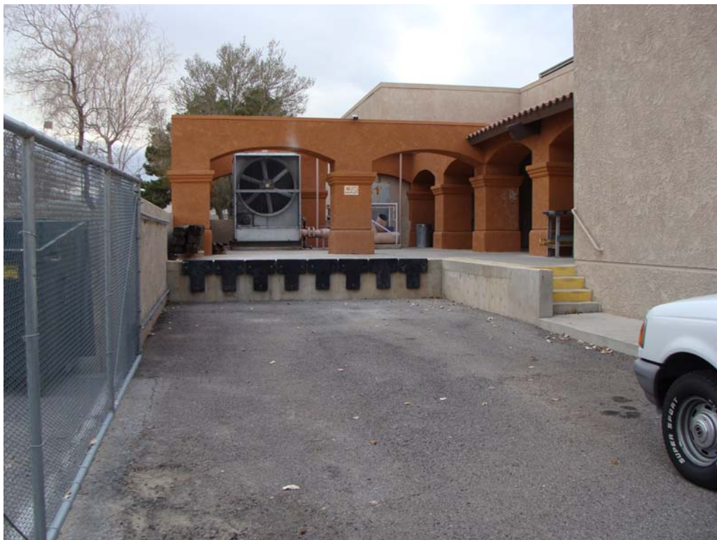
Las Vegas Museum & Historical Society - Site #9834 Description: Loading dock with cooling tower beyond.
