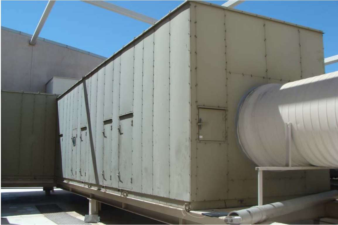
Grant Sawyer Office - Building #1680 Description: View of roof top mechanical equipment.
