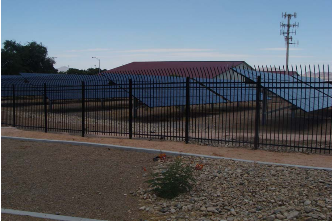
Grant Sawyer Office Site - Site #9835 Description: View of the solar array.
