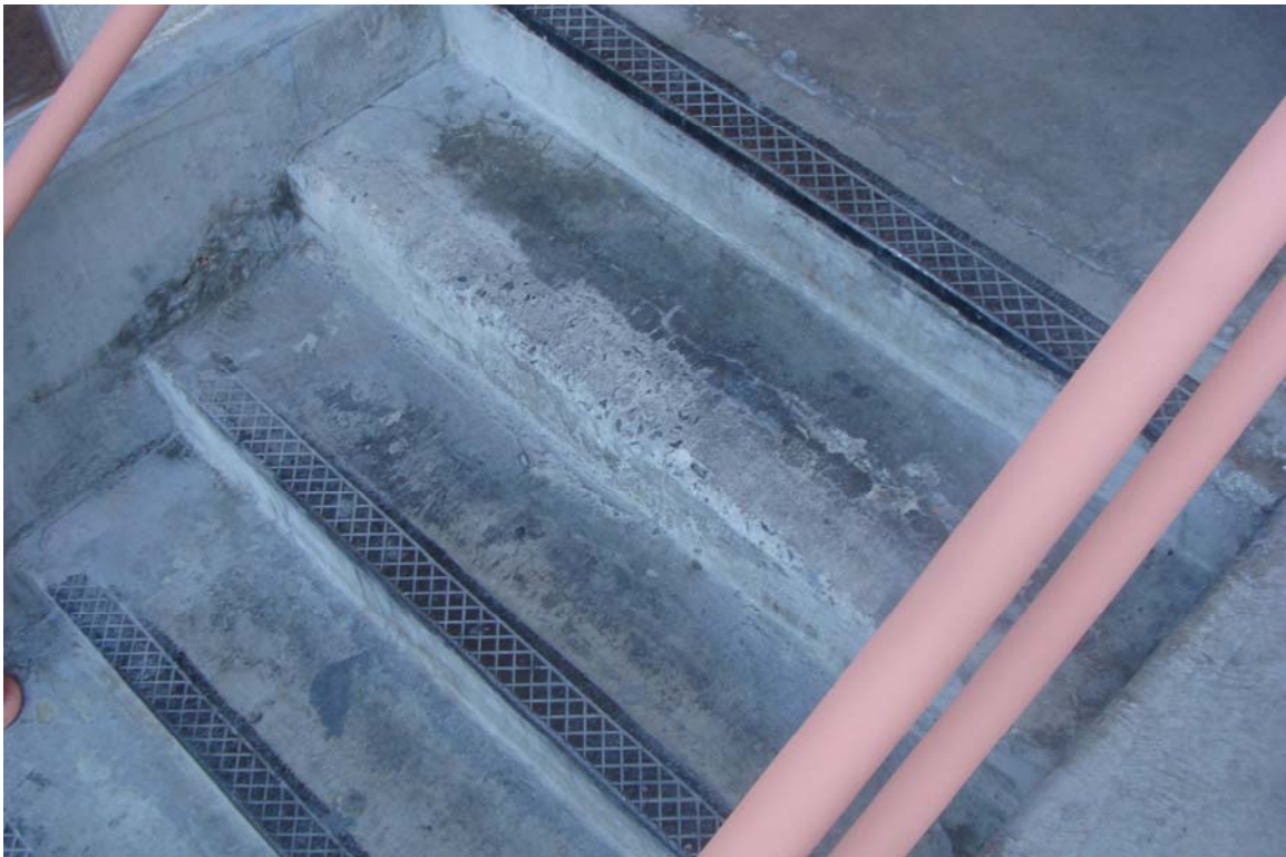
Grant Sawyer Office - Building #1680 Description: Damaged concrete stairs at loading dock.
