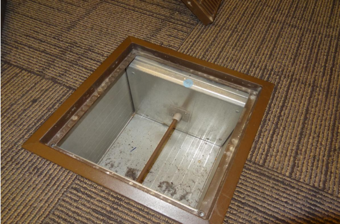
DETR Las Vegas Office - FCA Building #2565 Description: Access floor vent.
