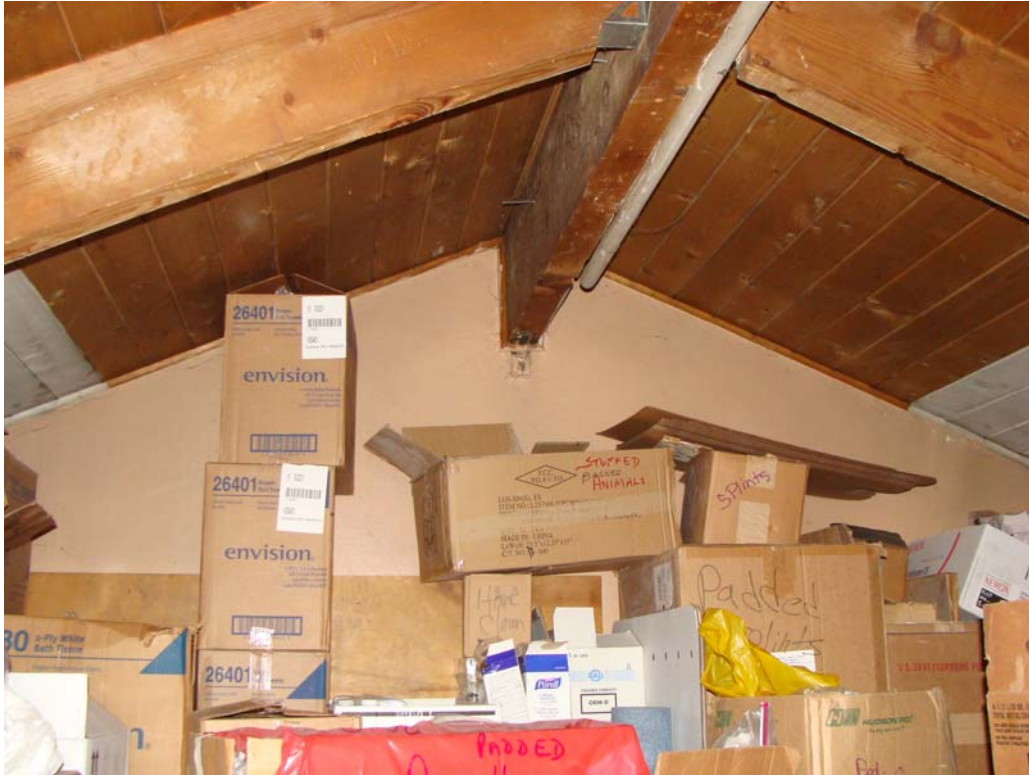
Kyle Canyon Fire Station No. 1 - Building #0285 Description: View of the unisulated attic space.
