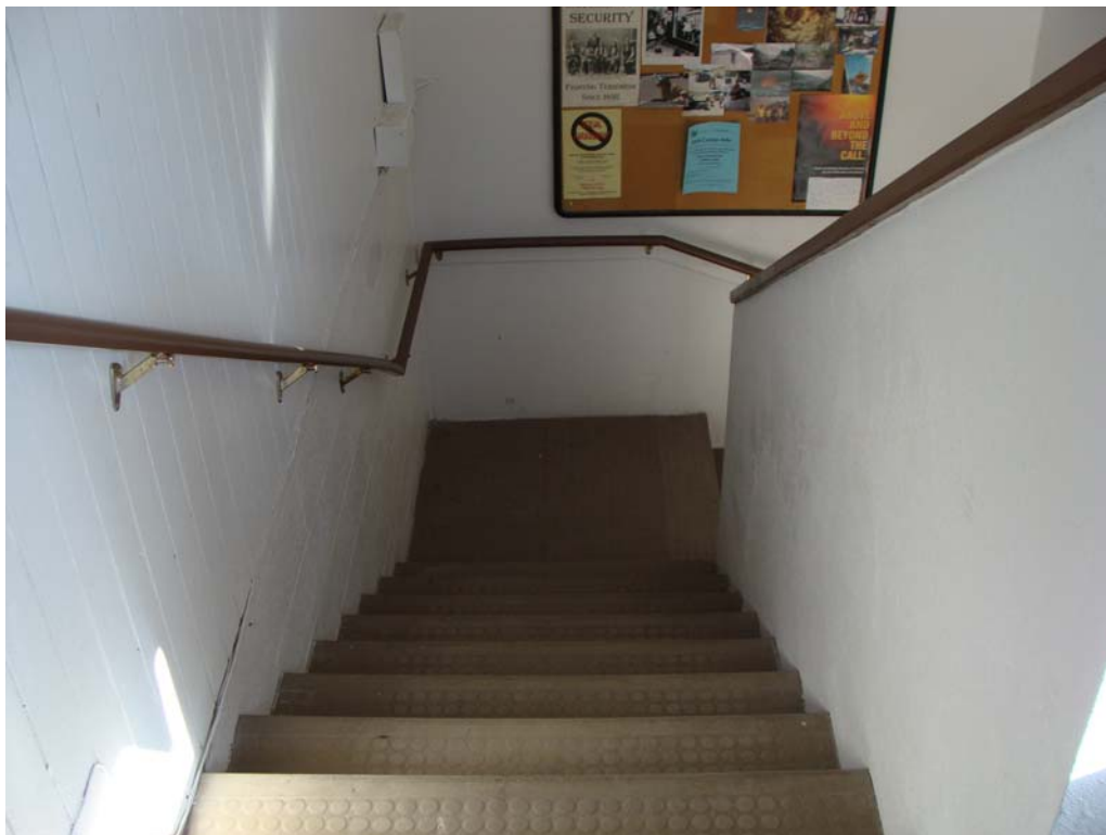
Kyle Canyon Fire Station No. 1 - Building #0285 Description: Entry stairs to living quarters.
