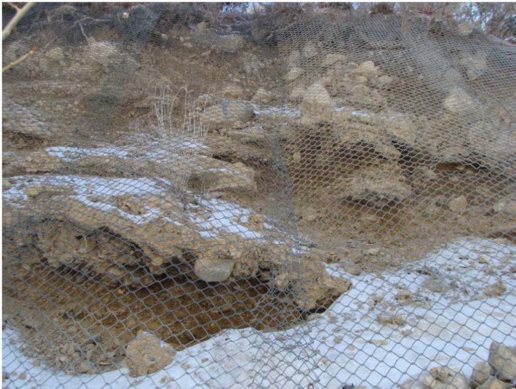
Kyle Canyon Fire Station No. 1 Site - Site #9843 Description: Unstable slope directly behind station.
