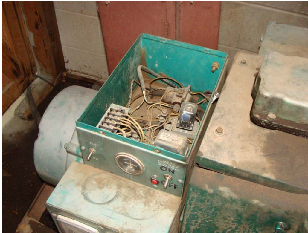
Kyle Canyon Fire Station No. 1 - Building #0285 Description: Emergency generator.
