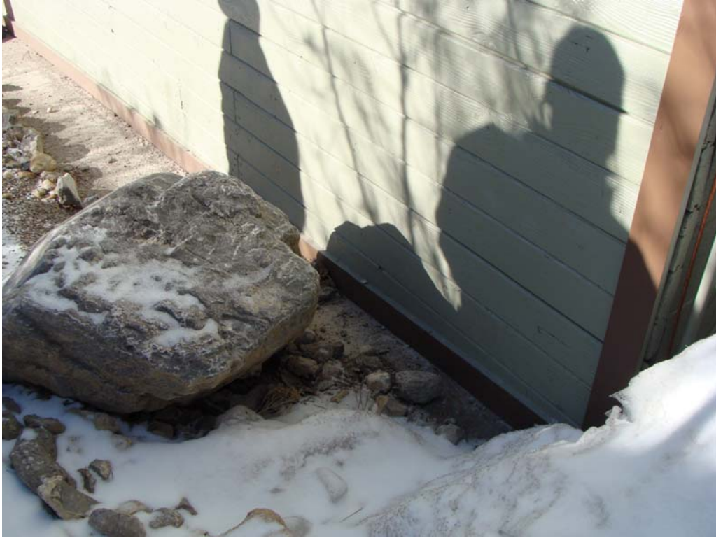
Kyle Canyon Fire Station No. 1 Site - Site #9843 Description: Fallen debris from slope above.
