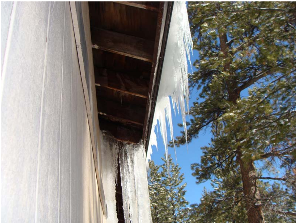
Lee Canyon Fire Station No. 2 - Building #0284 Description: Ice damming on the roof.
