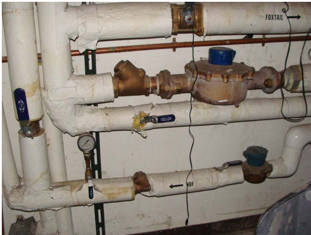
Lee Canyon Fire Station No. 2 - Building #0284 Description: Domestic water distribution piping.
