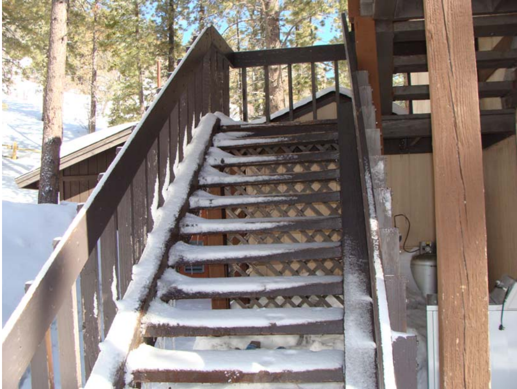
Lee Canyon Fire Station No. 2 - Building #0284 Description: Entry stairs, only entrance to facility.
