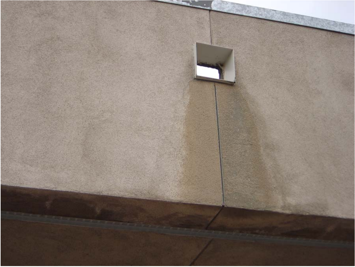
Reno Motor Pool Index No. 2483 Description: Fueling canopy roof drain.
