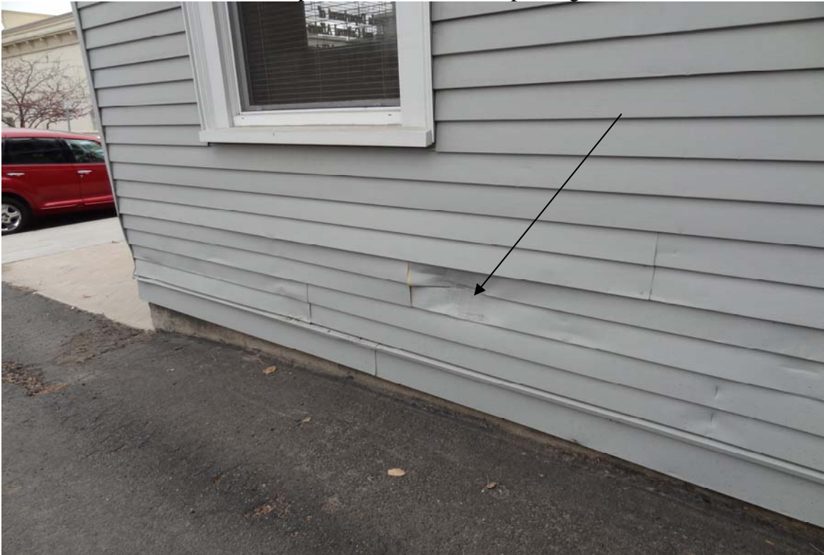
Museum Administration Office - Building #2028 Description: Exterior of the building, note damaged siding.
