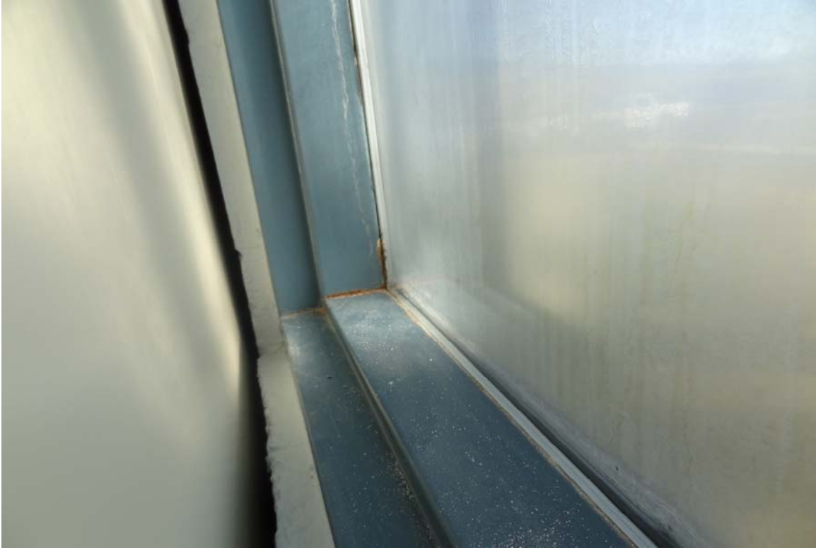
DPS Training Facility - Building #0898 Description: Interior of window / frame in need of upgrade.
