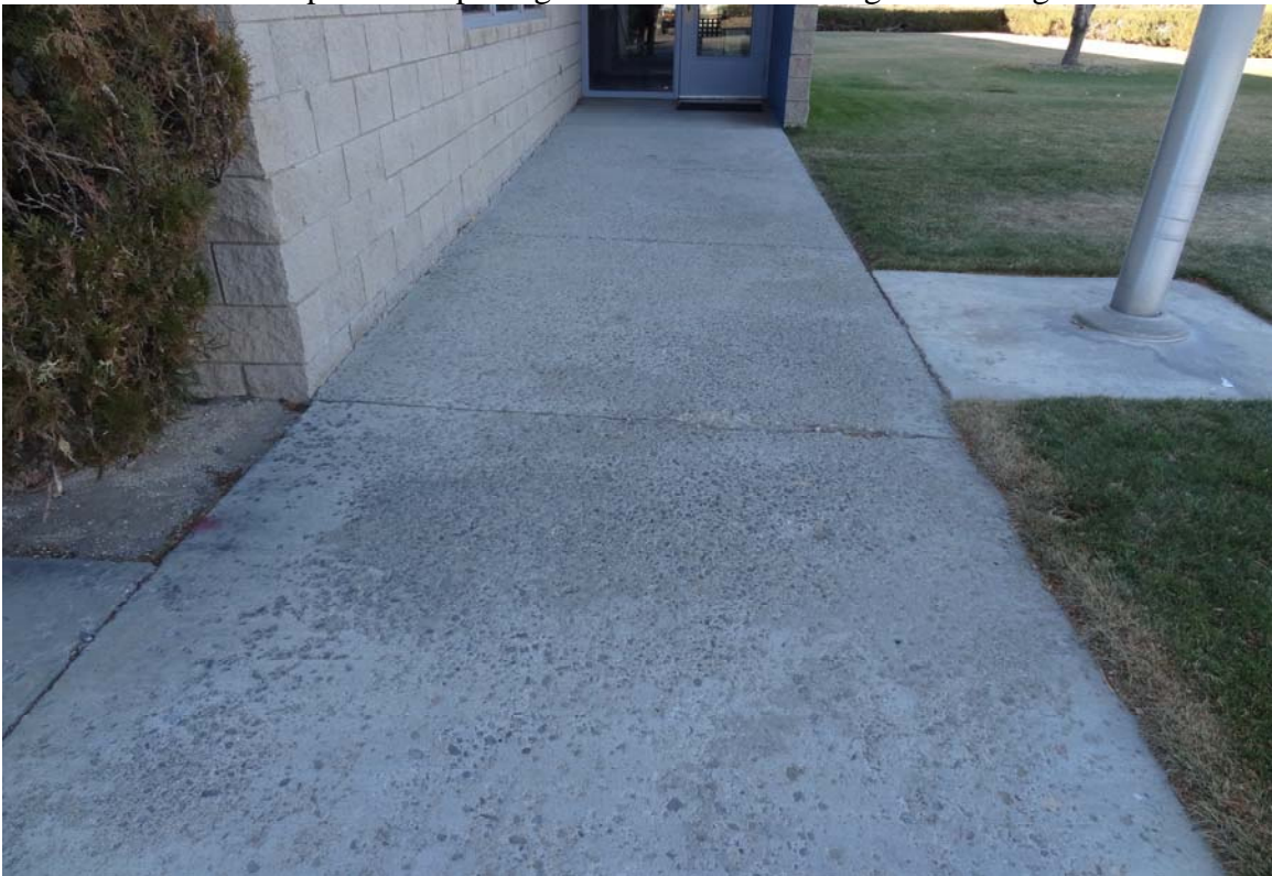
DPS Training Facility Site - Site #9851 Description: Damaged concrete walkway at entrance to building.
