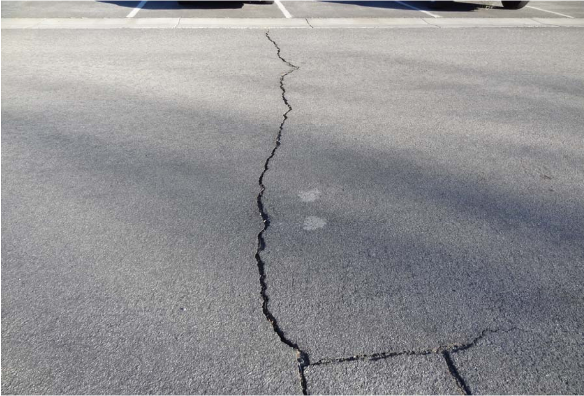
DPS Training Facility Site - Site #9851 Description: AC paving in need of crack filling and sealing.
