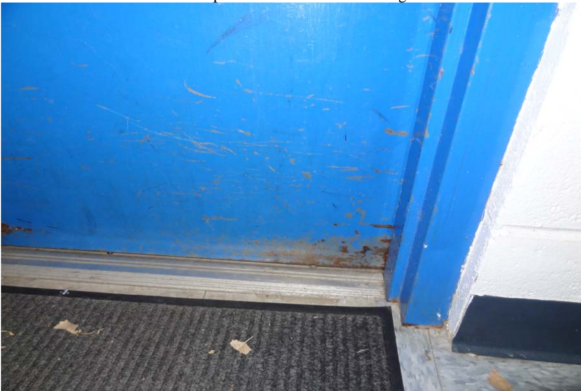
DPS Training Facility - Building #0898 Description: Exterior door due for replacement.
