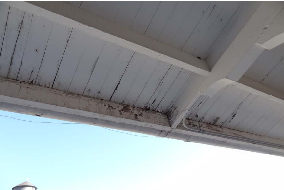
East Ely Railroad Depot - Building #2227 Description: Water damage on north shed roof.
