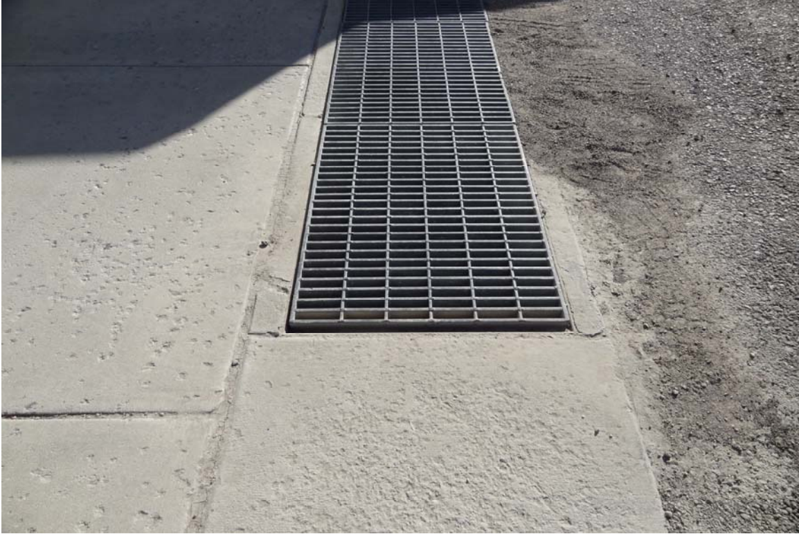
East Ely Railroad Depot Museum Site - Site #9857 Description: Grate on south side in need of modifications.
