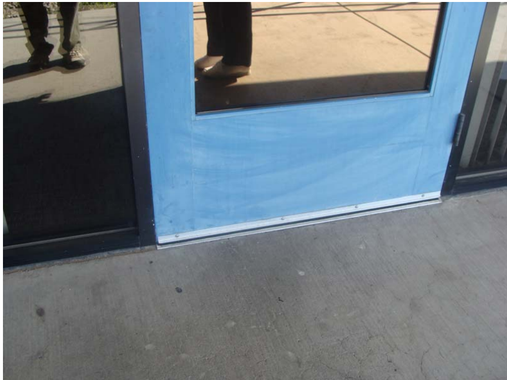
DMV Reno Office - Building #0272 Description: Exterior door in need of replacement.
