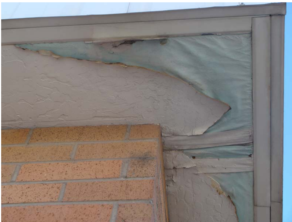
Reno DMV Inspection Station - Building #2169 Description: Damaged exterior gypsum board soffit.
