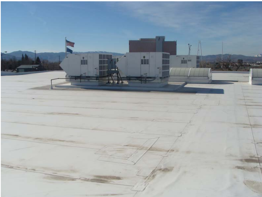
DMV Reno Office - Building #0272 Description: Roof and roof top HVAC equipment.
