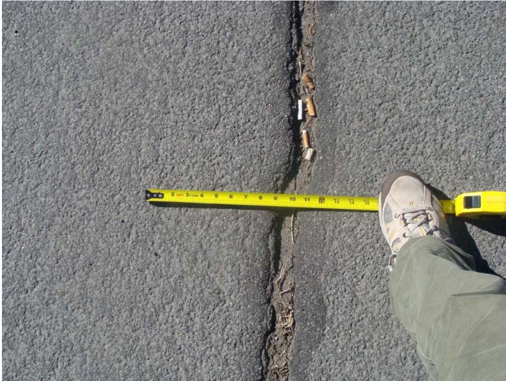
Department of Motor Vehicles Office - Site #9858 Description: Cracking in paved parking area.
