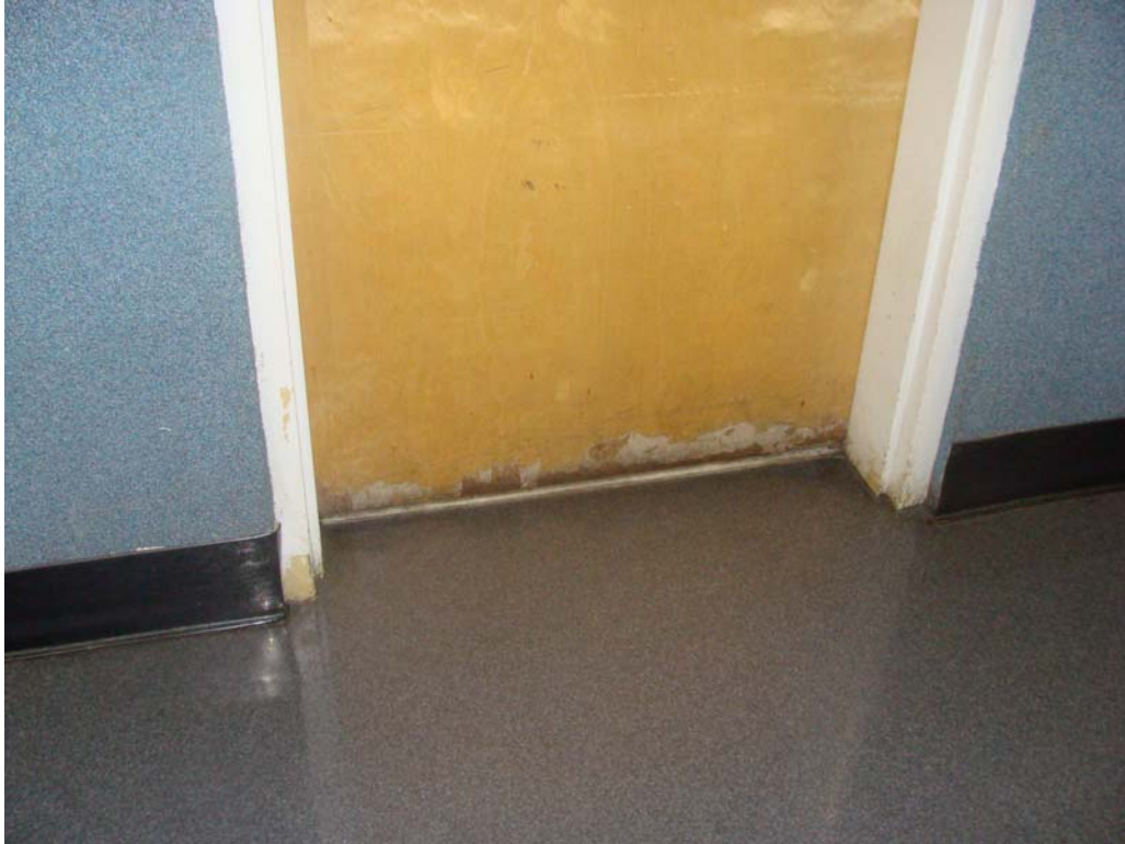
DMV Reno Office - Building #0272 Description: Typical interior wood door in need of refinishing.
