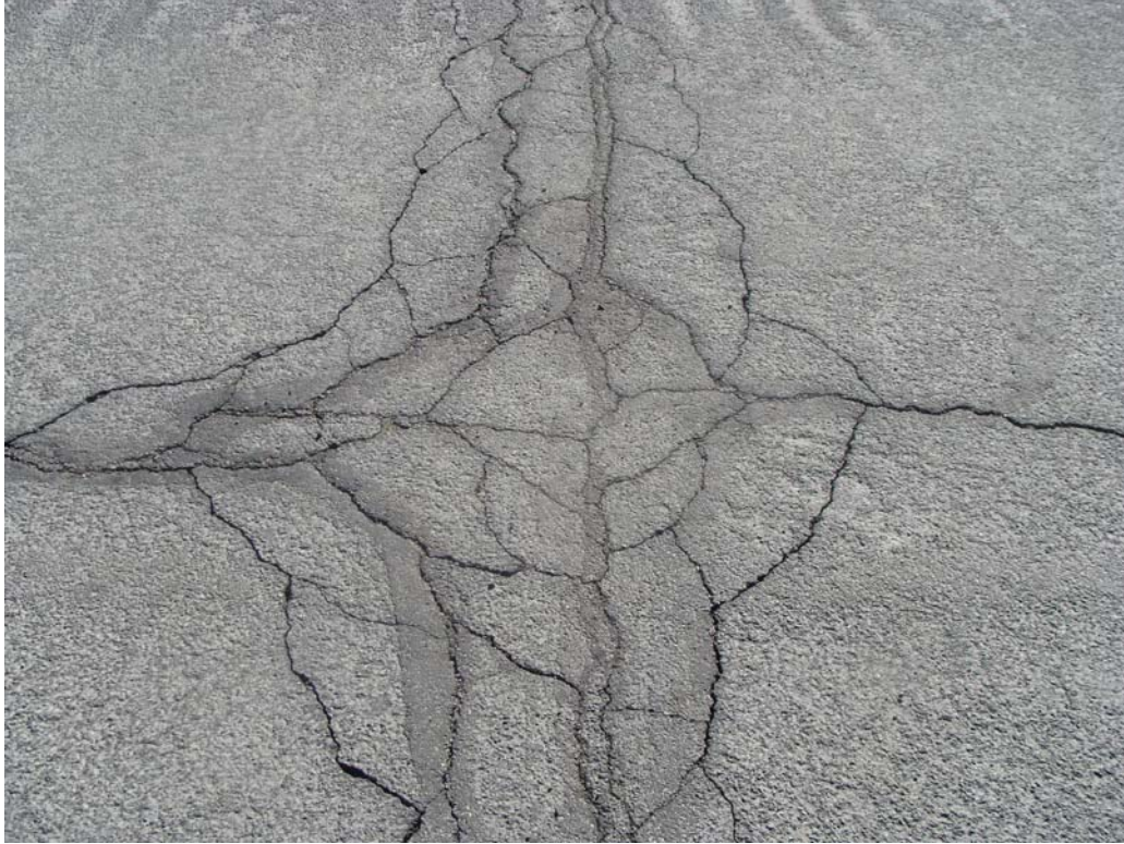
Department of Motor Vehicles Office - Site #9858 Description: Alligator cracking in pavement.
