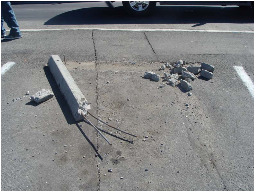
Department of Motor Vehicles Office - Site #9858 Description: Damaged wheel stop.
