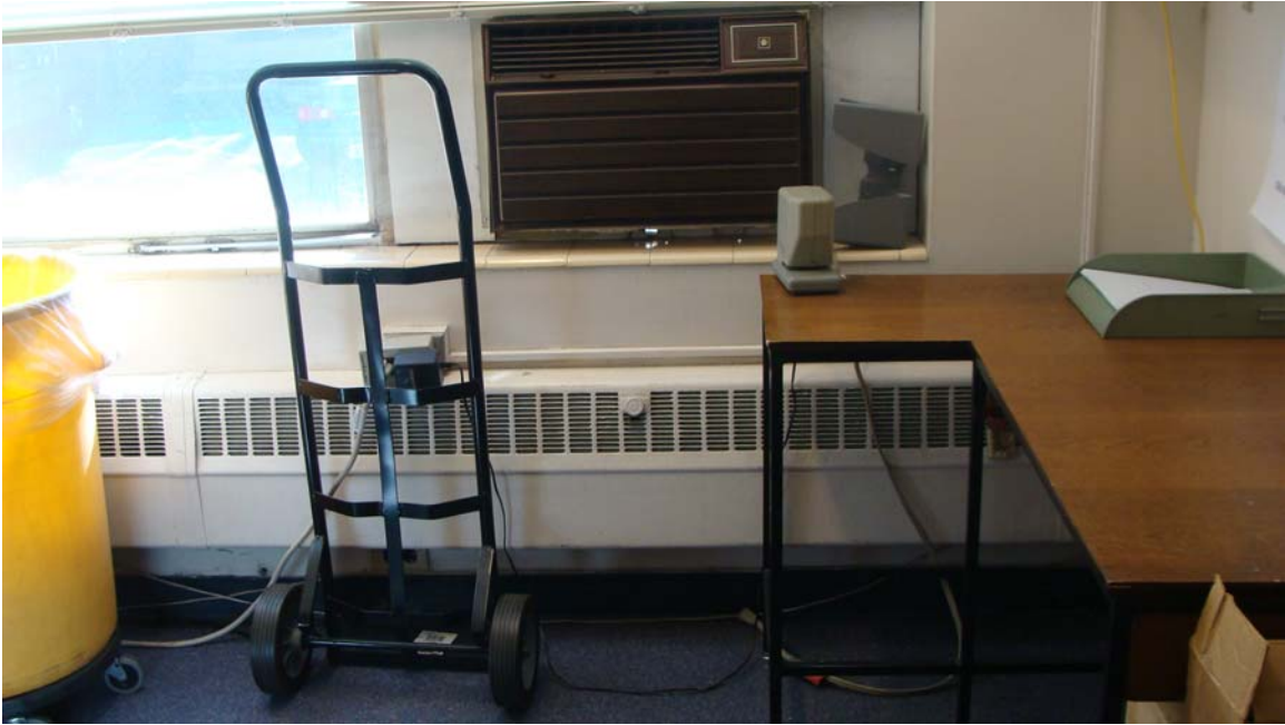
Blasdel Office Building - Building #0200 Description: Typical exterior wall mounted radiator.
