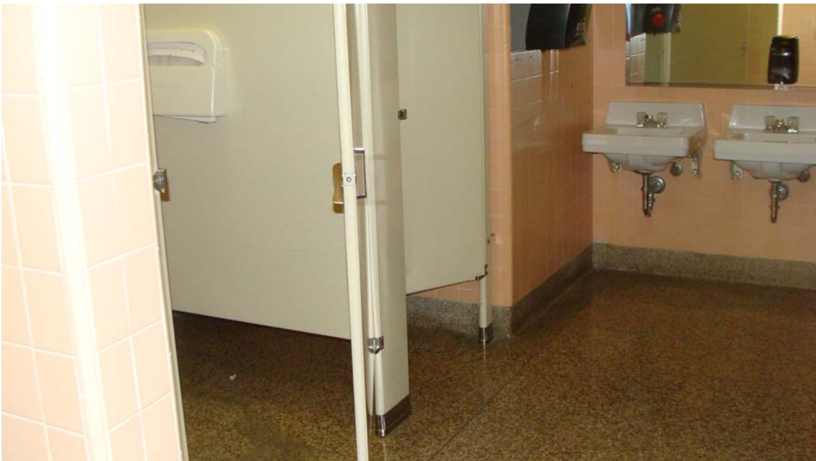
Blasdel Office Building - Building #0200 Description: Women's restroom in need of ADA upgrades.
