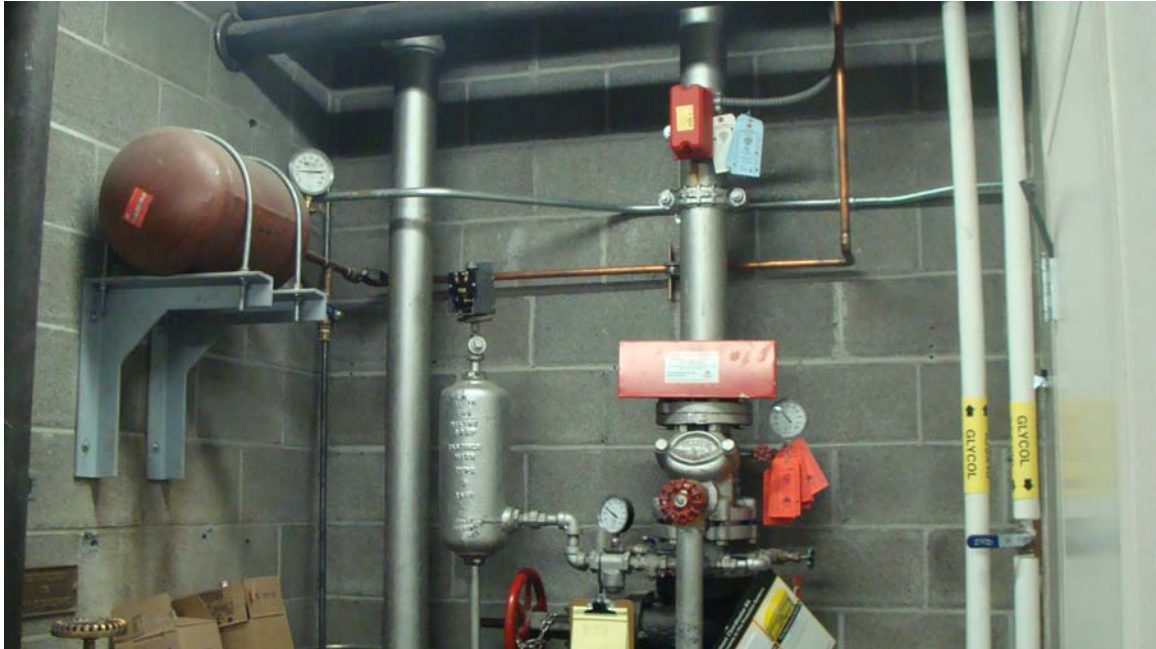
Blasdel Office Building - Building #0200 Description: Fire sprinkler riser in basement.
