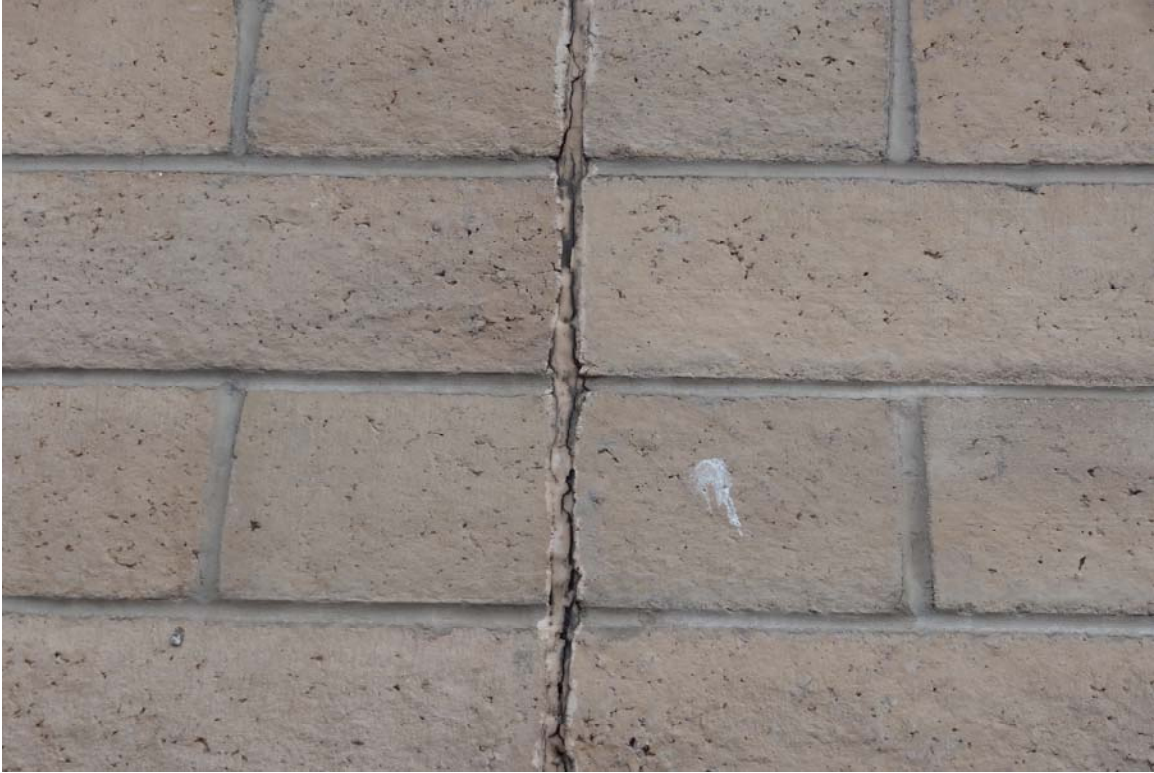
Carson City Motor Pool - Building #0204 Description: Control joint in need of caulking.
