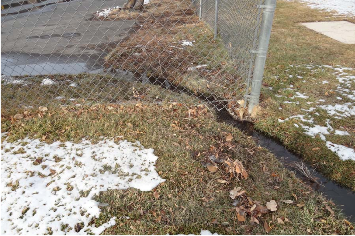
Carson City Motor Pool Site - Site #9862 Description: Area where drainage improvements are needed.
