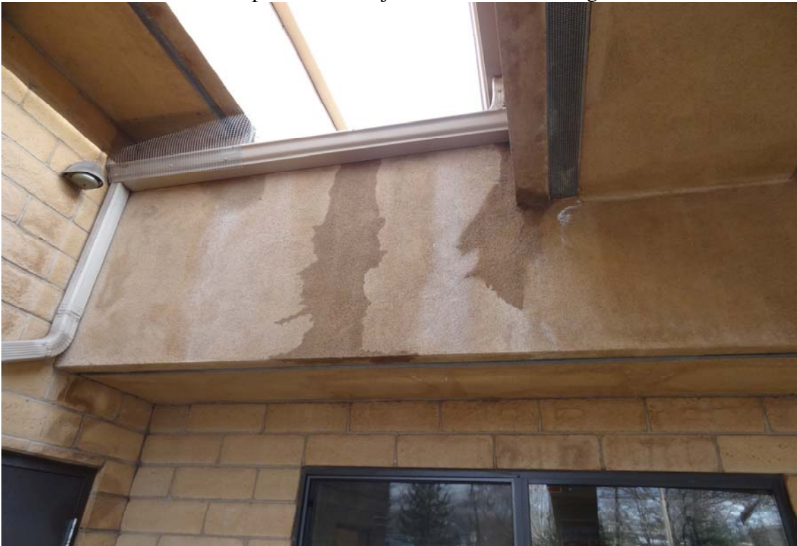
Carson City Motor Pool - Building #0204 Description: Water damaged stucco / leaking gutters.
