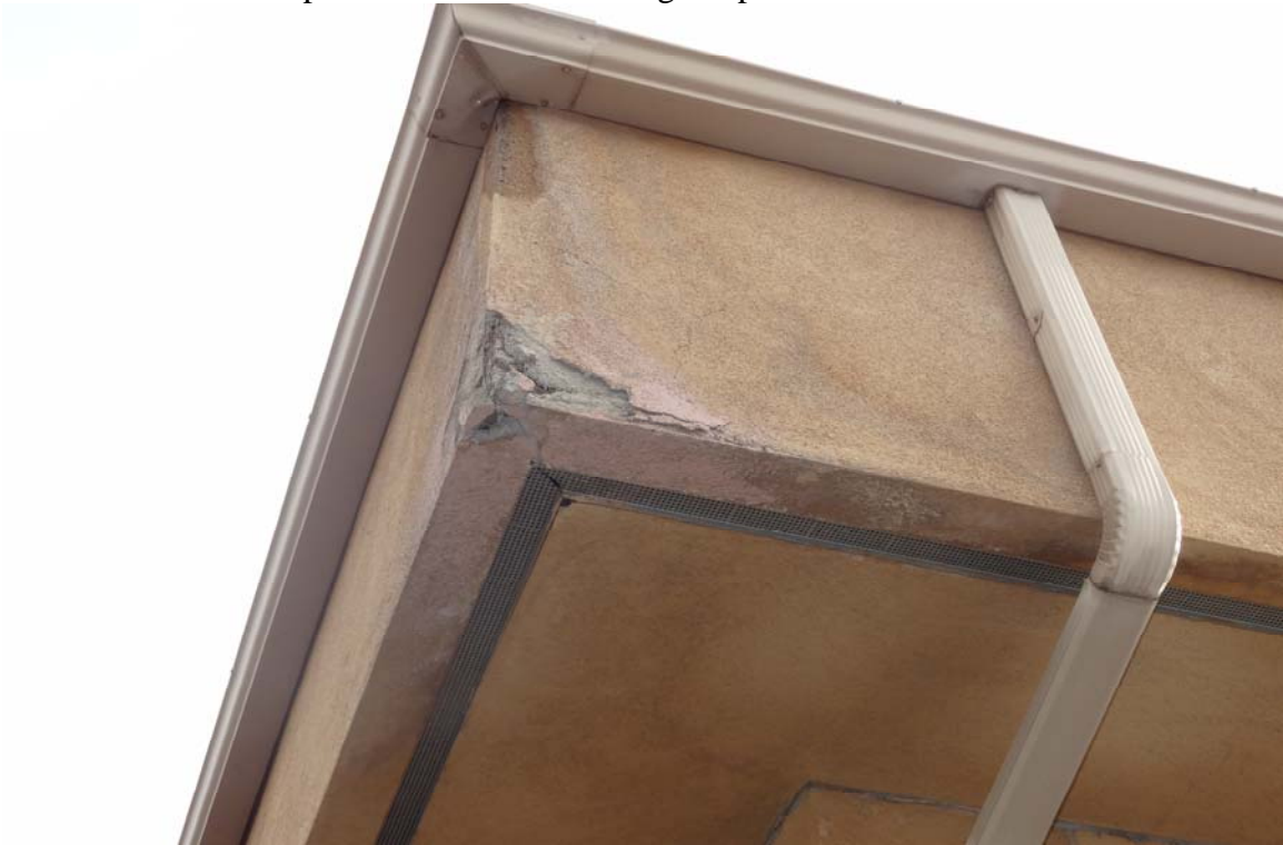
Carson City Motor Pool - Building #0204 Description: Damaged stucco fascia.
