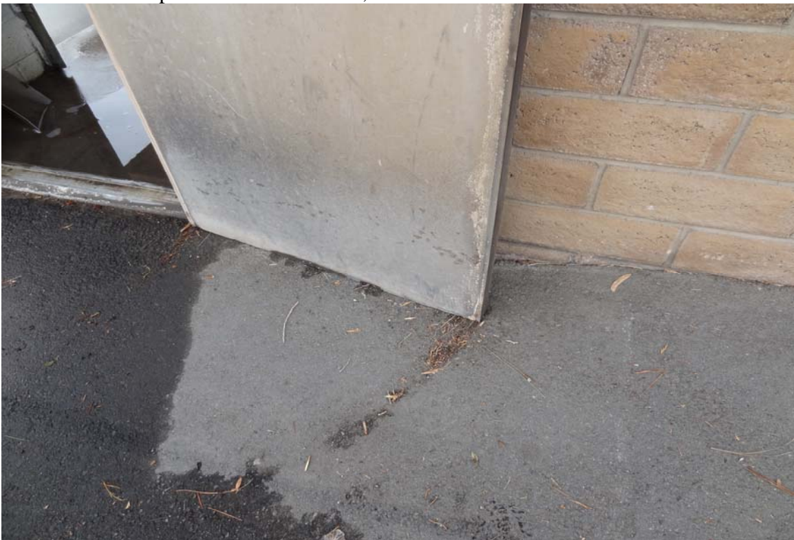
Carson City Motor Pool - Building #0204 Description: Damaged exterior door.
