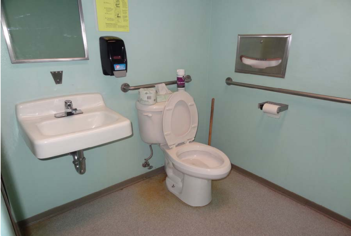
Carson City Motor Pool - Building #0204 Description: Unisex restroom, note fixture locations and toilet seat.
