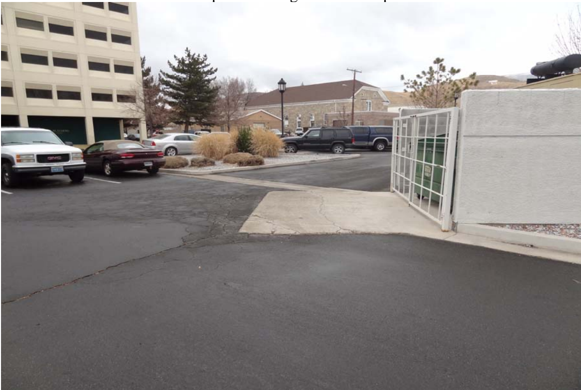
Carson City State Offices Site - Site #9864 Description: Dumpster area paving / concrete damage.
