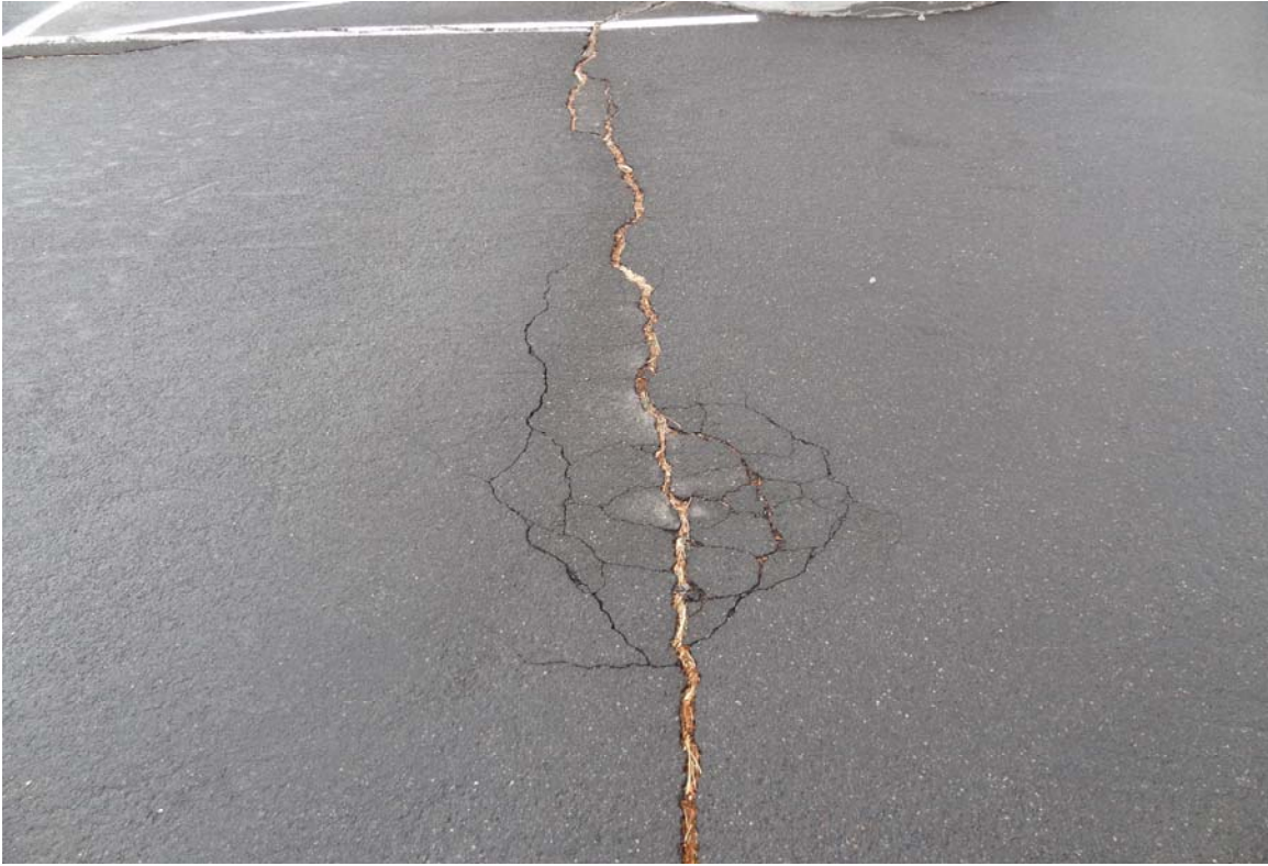
Carson City State Offices Site - Site #9864 Description: Paving in need of repair.
