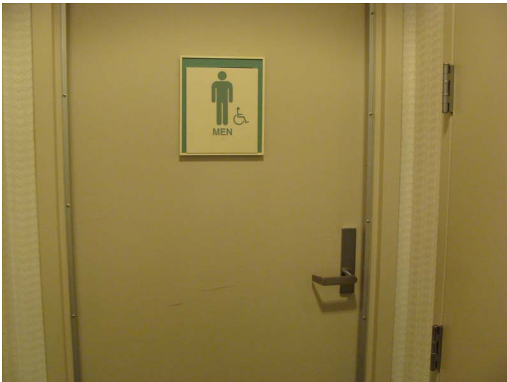
Nevada State Library & Archives - Building #1675 Description: ADA signage in wrong location.
