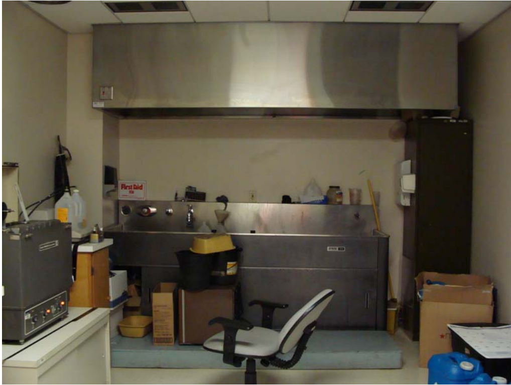
Nevada State Library & Archives - Building #1675 Description: Non-operational fume hood.
