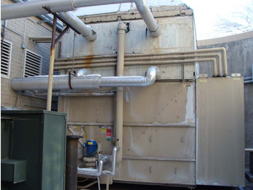
Nevada State Library & Archives - Building #1675 Description: Non-operational cooling tower.
