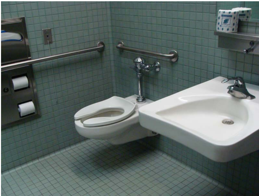
Nevada State Library & Archives - Building #1675 Description: ADA unisex restroom, note flush handle on wrong side.
