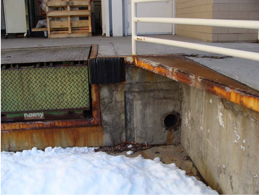
Nevada State Library & Archives - Building #1675 Description: Loading dock in need of rehabilitation.
