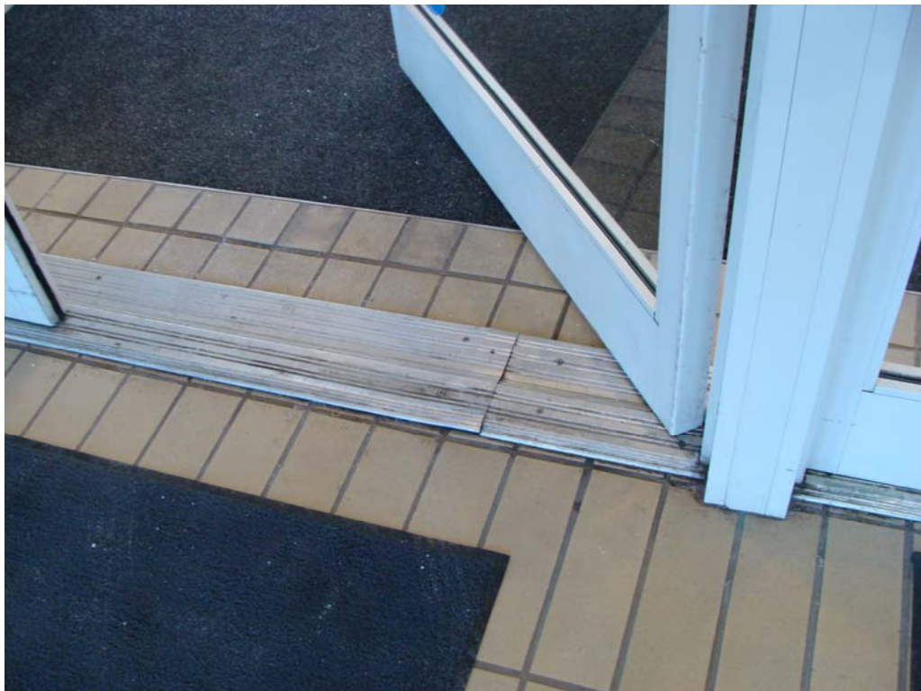
Nevada State Library & Archives - Building #1675 Description: Lobby entrance threshold in need of replacement.
