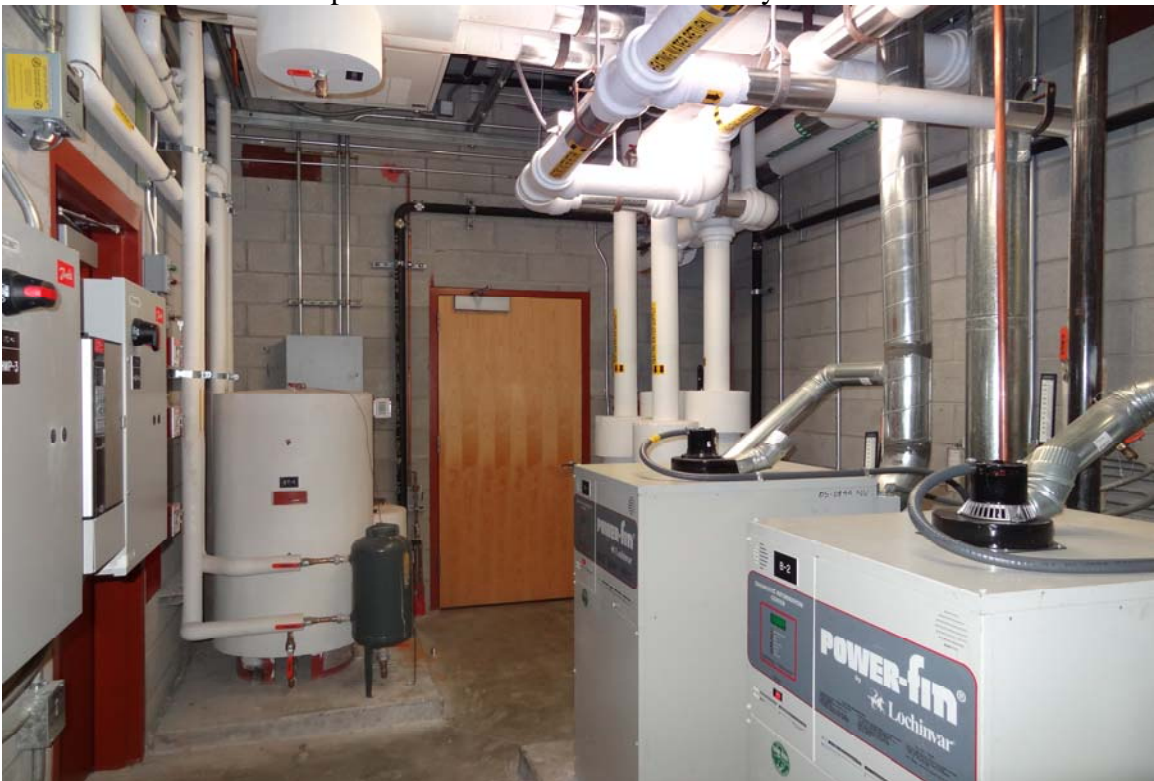
North Decatur DMV Services Center - Building #2453 Description: View of the mechanical room.
