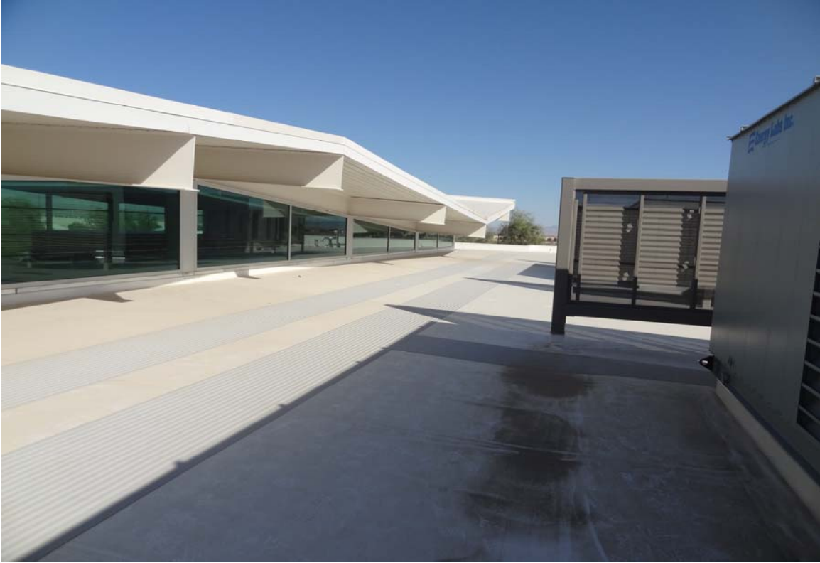
North Decatur DMV Services Center - Building #2453 Description: View of the roof / clerestory windows.
