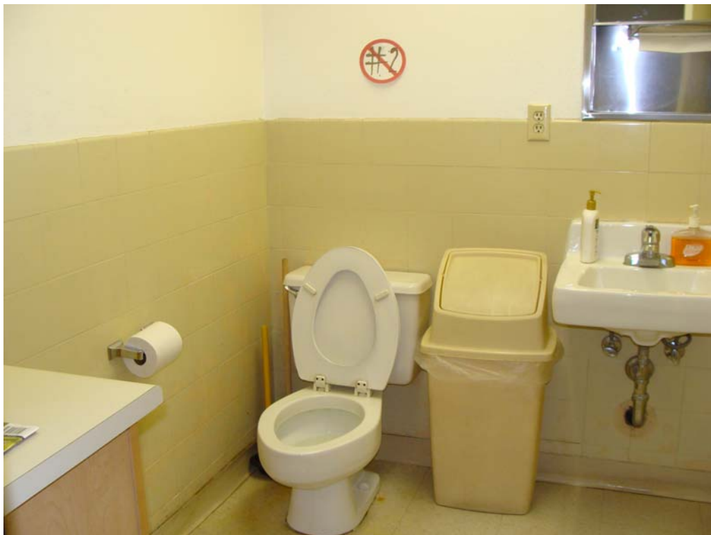
Wildlife Office Annex - Building #0704 Description: Restroom in need of an upgrade.
