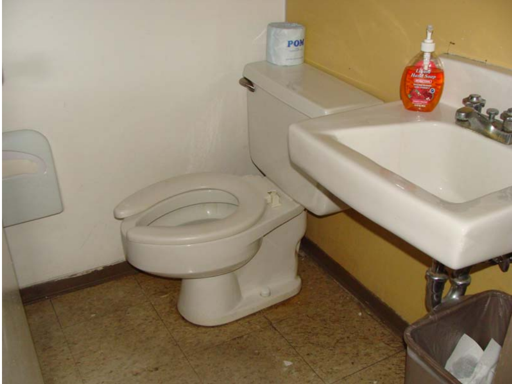
NDOW Regional Office - Building #0260 Description: Restroom in need of upgrading.
