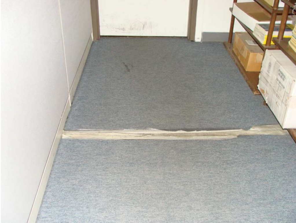
NDOW Regional Office - Building #0260 Description: Carpet in need of replacement.
