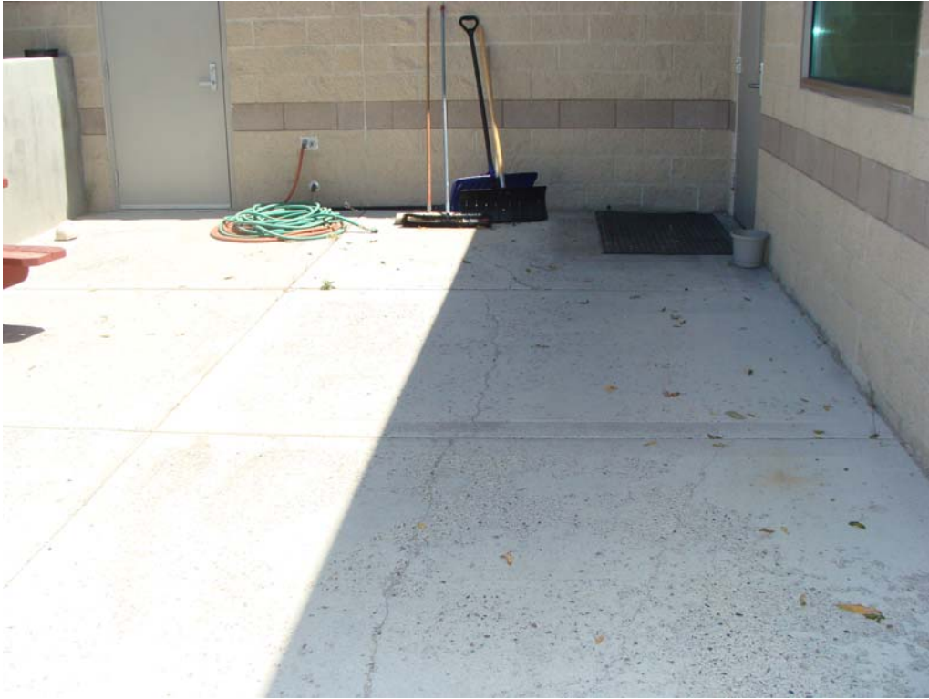
Eastern Region NDOW Office - Building #2297 Description: Area of damaged P. C. concrete.
