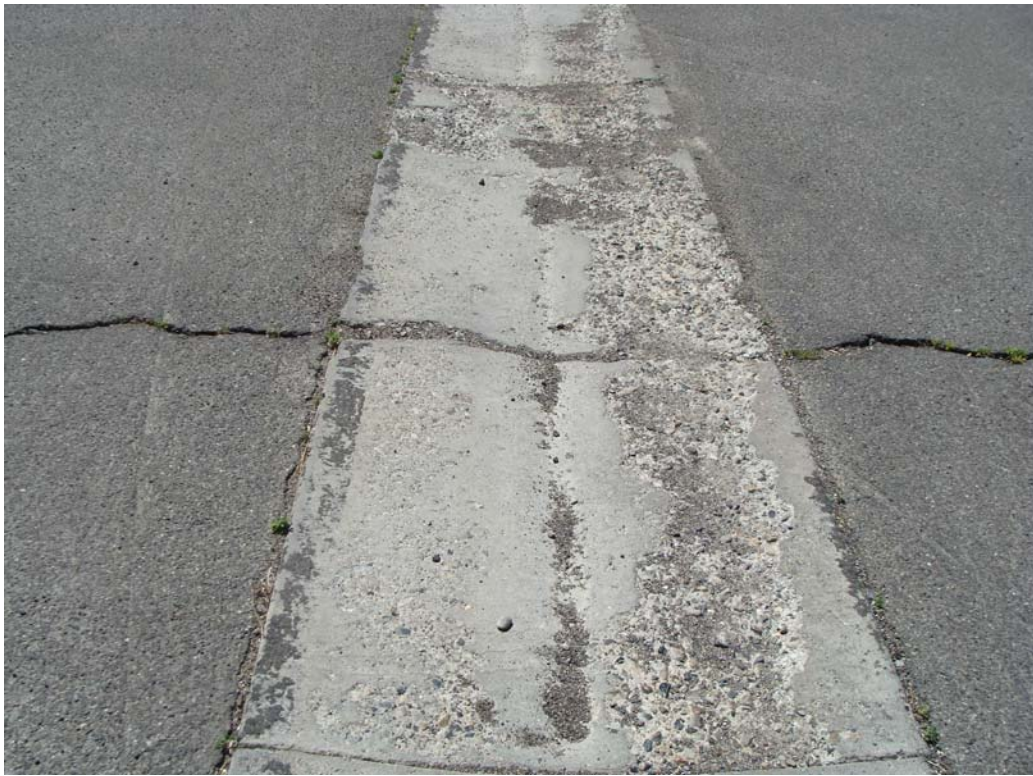
Eastern Regional Office Site - Site #9880 Description: Damaged valley gutter.
