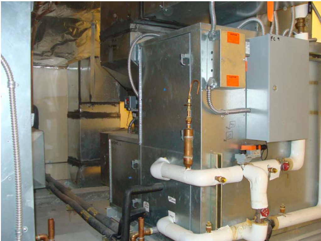
Eastern Region NDOW Office - Building #2297 Description: HVAC equipment in Mezzanine.
