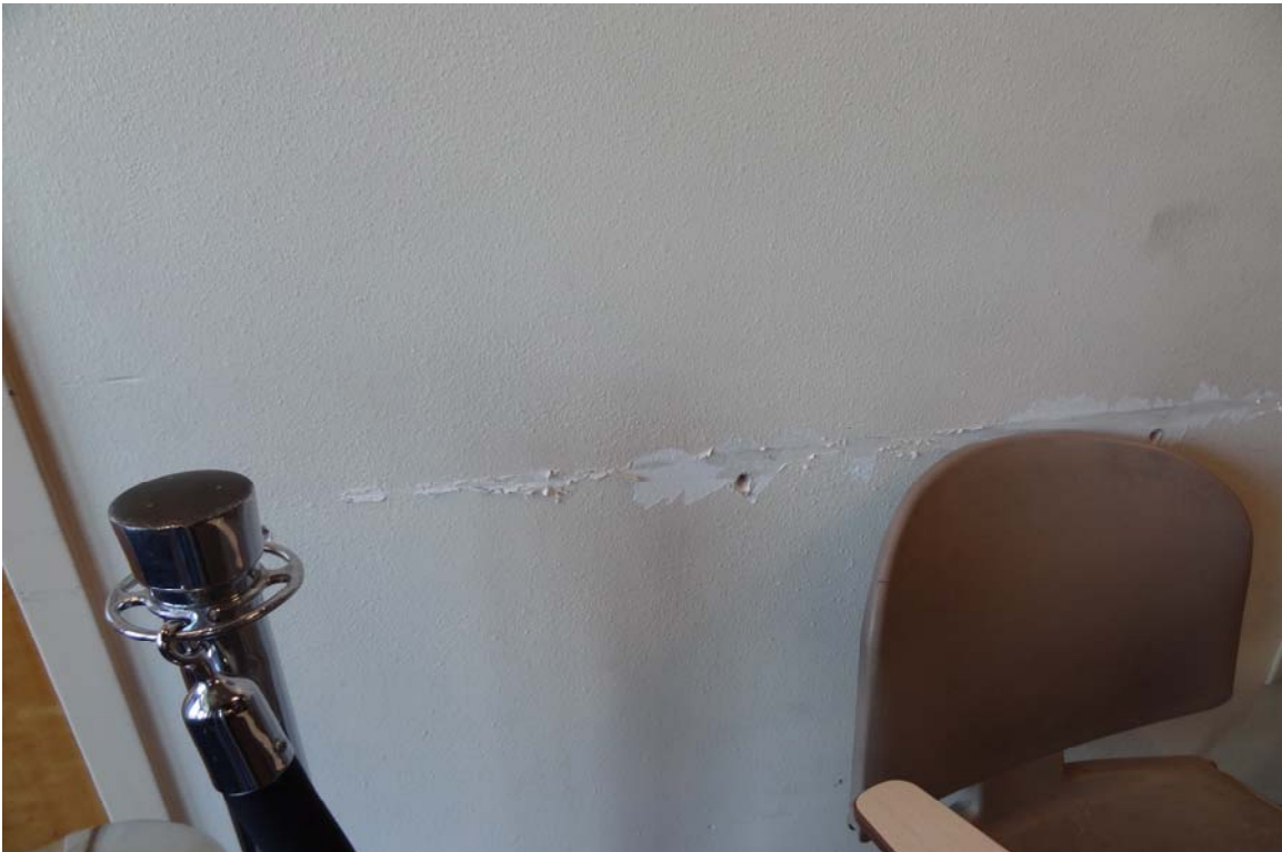
Henderson DMV Office - Building #2000 Description: Damage to wall surface in public waiting area.
