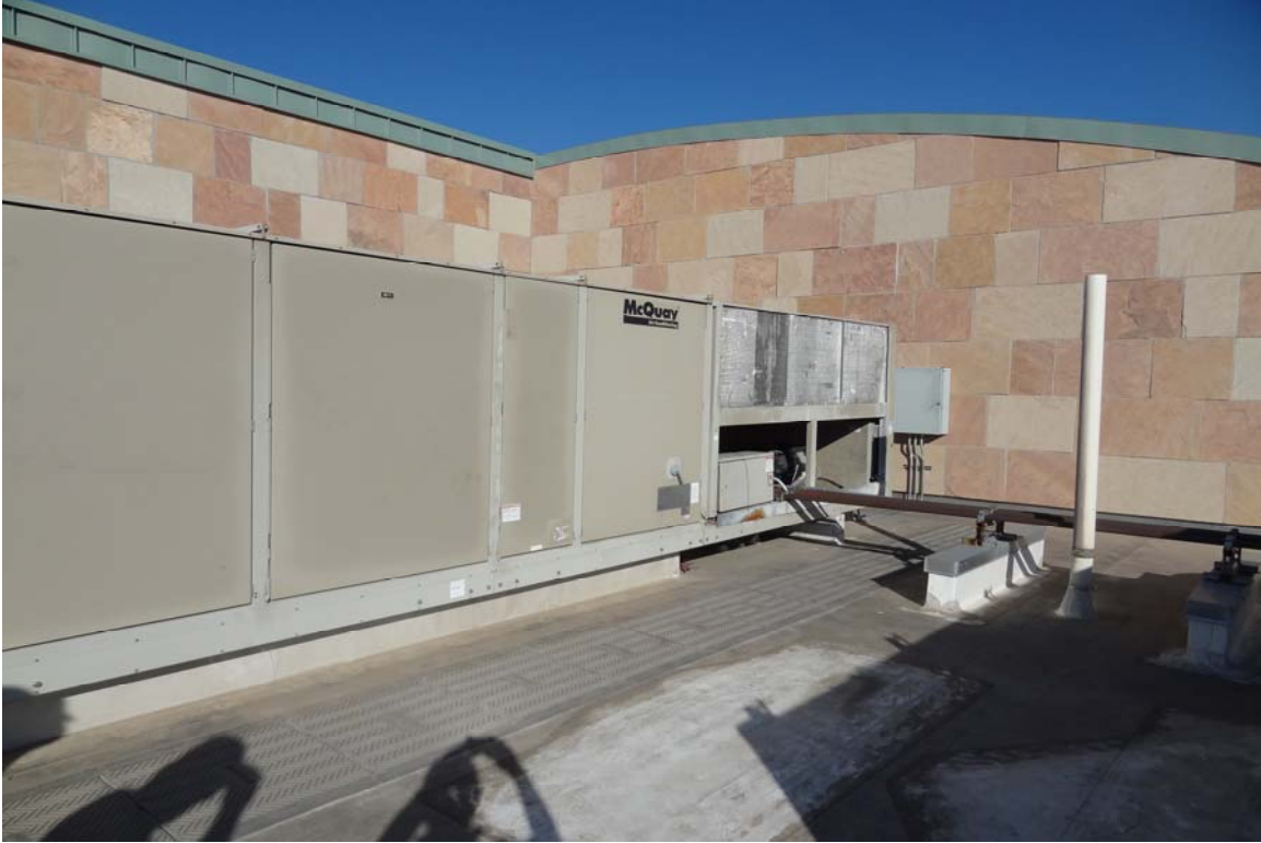
Henderson DMV Office - Building #2000 Description: Roof mounted HVAC unit.
