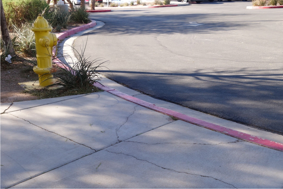
Southern Nevada Veterans Home Site – FCA Site #9889 Description: Sidewalk Replacement Needed.
