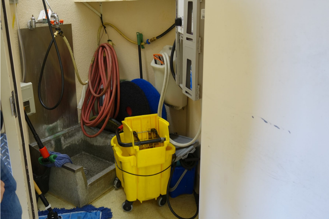
Southern Nevada Veterans Home – FCA Building #2106 Description: Janitors Closet Repairs Needed.
