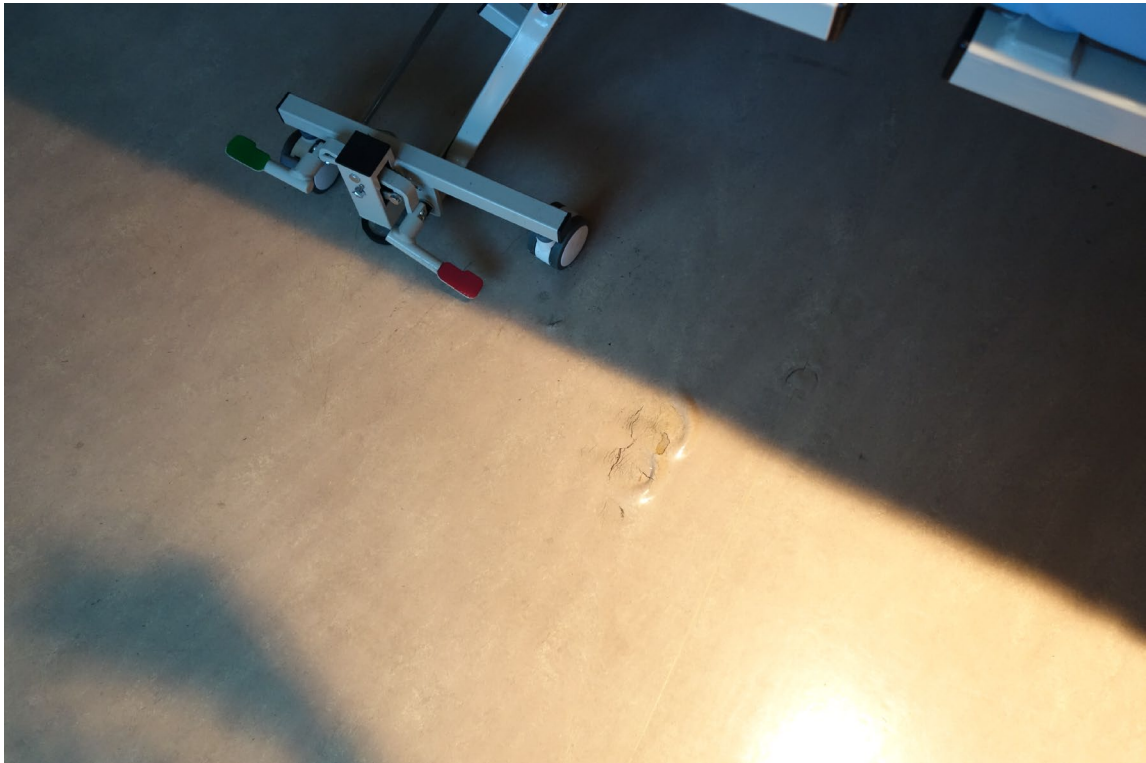
Southern Nevada Veterans Home – FCA Building #2106 Description: Flooring Replacement Needed.
