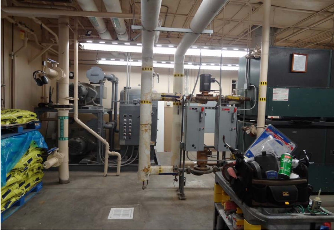
Southern Nevada Veterans Home - Building #2106 Description: View of the mechanical space.
