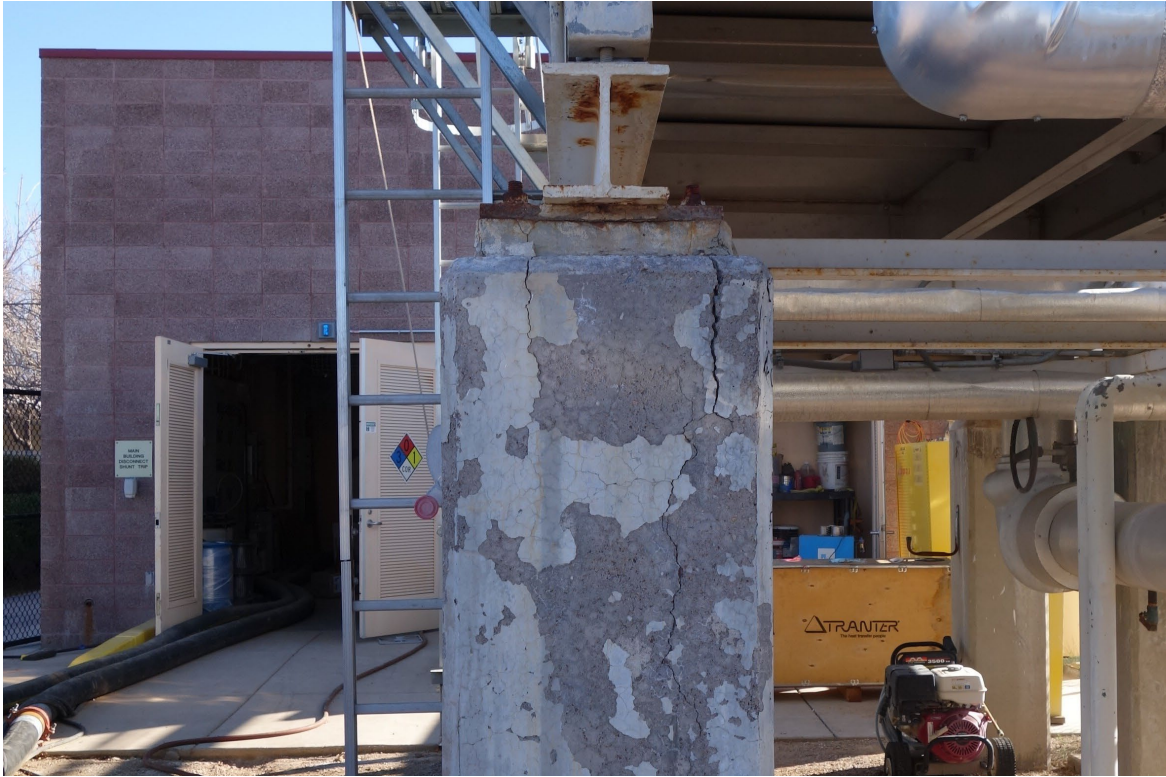
Southern Nevada Veterans Home – FCA Building #2106 Description: Cooling Tower Pier Replacement Needed.
