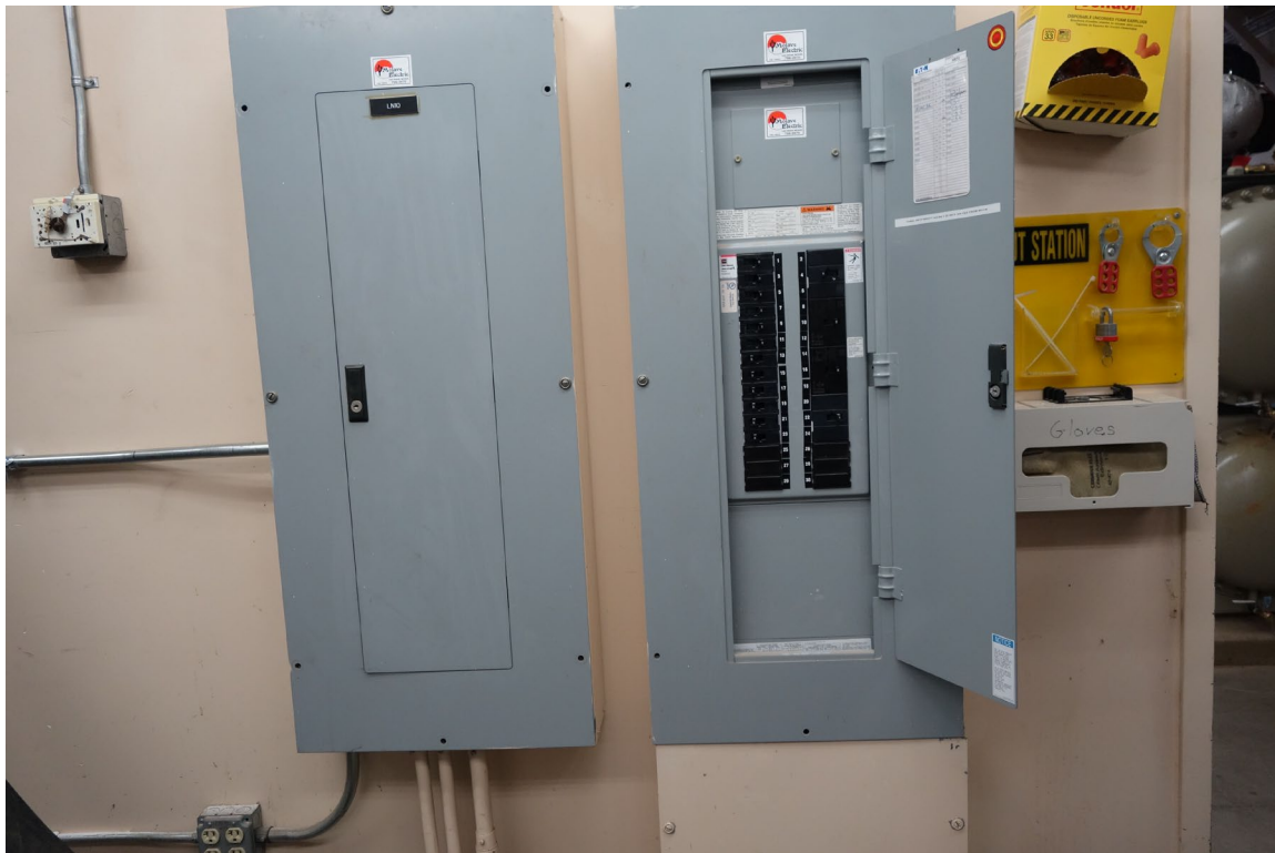
Southern Nevada Veterans Home – FCA Building #2106 Description: Arc Flash & Electrical Coordination Study Needed.
