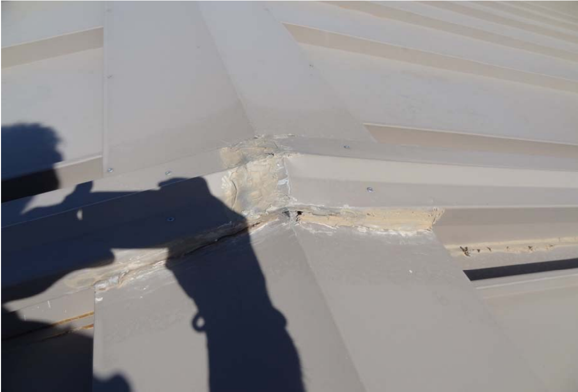
Southern Nevada Veterans Home - Building #2106 Description: Area of leaking metal roof panels.
