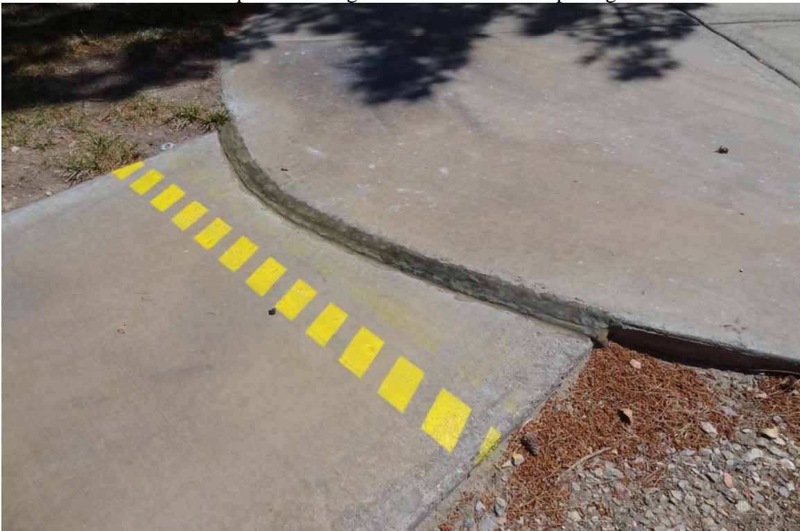
Southern Nevada Veterans Memorial Cemetery Site – FCA Site #9890 Description: Concrete step in need of grinding.
