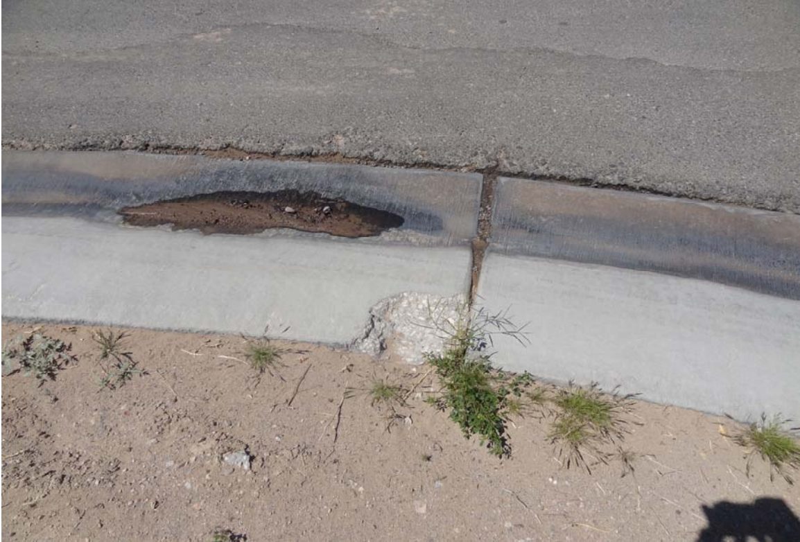
Southern Nevada Veterans Memorial Cemetery Site – FCA Site #9890 Description: Damaged roll curb and A. C. paving.
