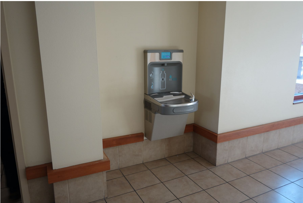
Rawson-Neal Psychiatric Hospital – FCA Building #2508 and #2510 Description: Dual Level Drinking Fountain Needed.
