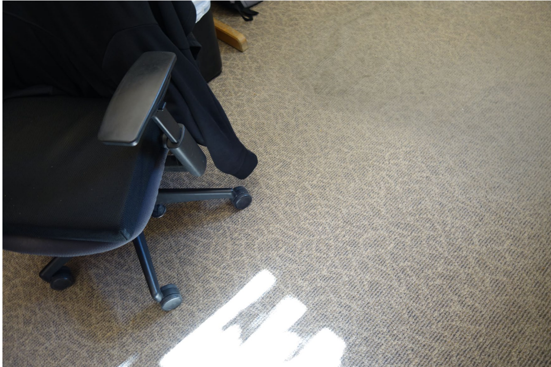
Rawson-Neal Psychiatric Hospital – FCA Building #2508 and #2510 Description: Office Carpet Replacement Needed.
