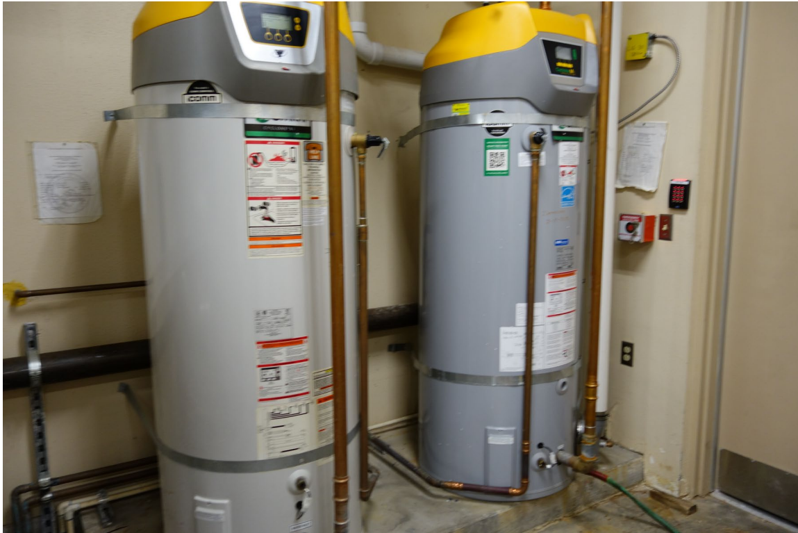
Rawson-Neal Psychiatric Hospital – FCA Building #2508 and #2510 Description: Water Heater Replacement Needed.
