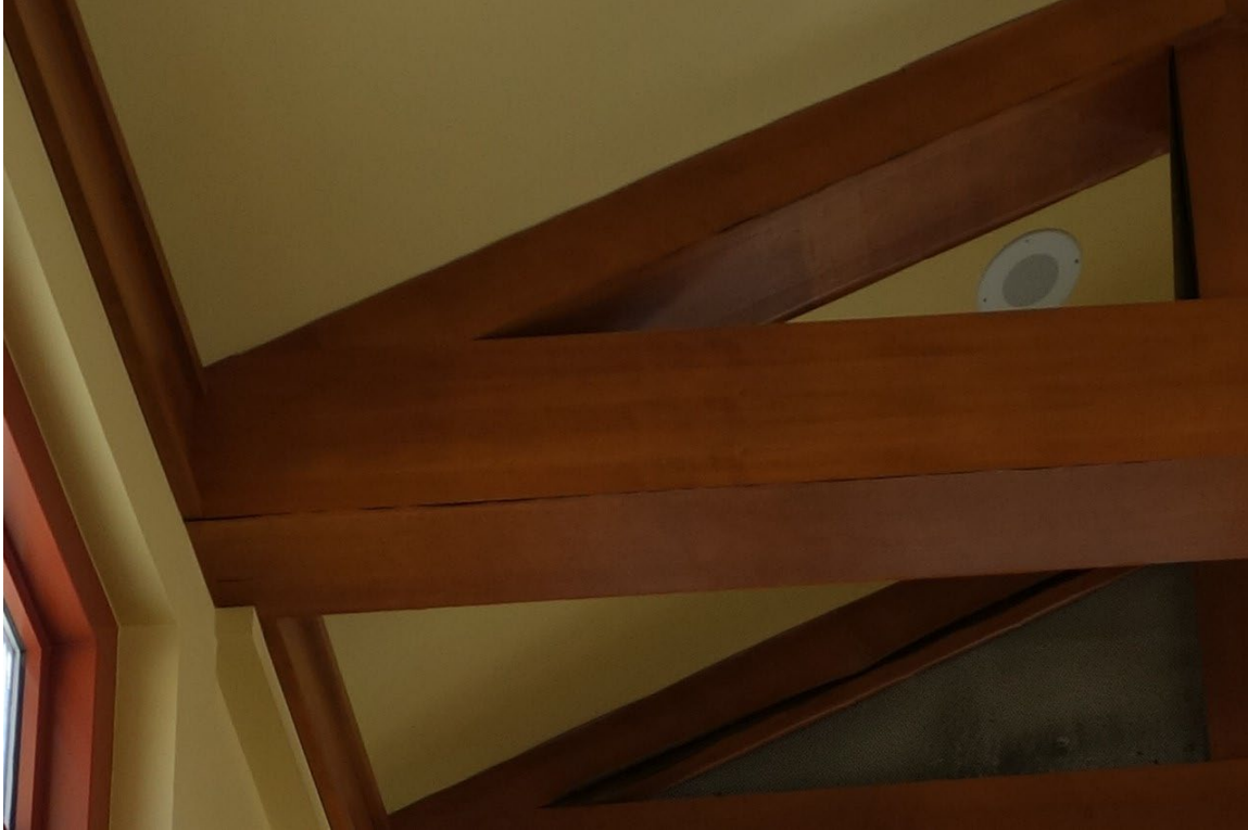
Rawson-Neal Psychiatric Hospital – FCA Building #2508 and #2510 Description: Delaminating Beams in Lobby.
