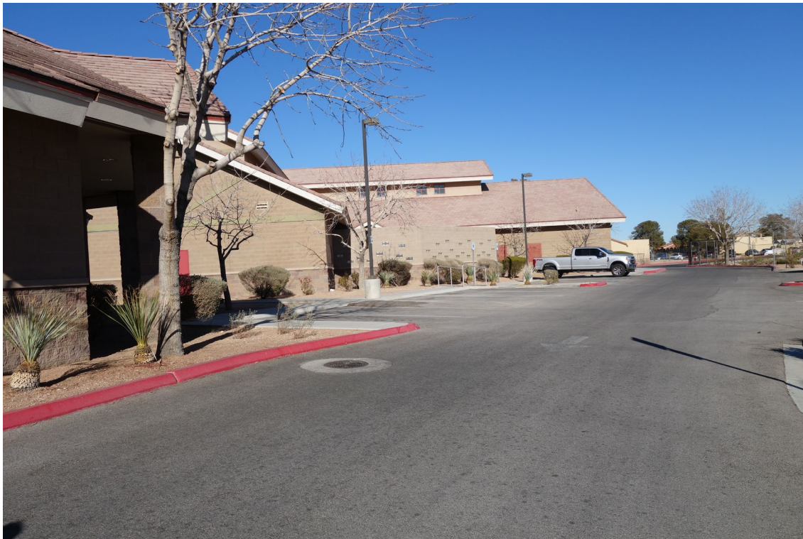
Rawson-Neal Psychiatric Hospital Site – FCA Site #9894 Description: View of the AC Paved East Parking Area.
