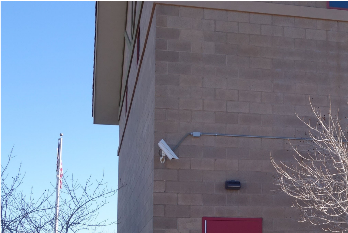
Rawson-Neal Psychiatric Hospital – FCA Building #2508 and #2510 Description: Security Surveillance Upgrade Recommended.
