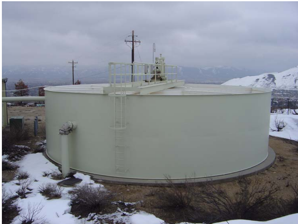
Marlette Lake / Ash Canyon- Building Index # 2504 Description: 1.5 Million Gallon Storage Tank / Waste Separator
