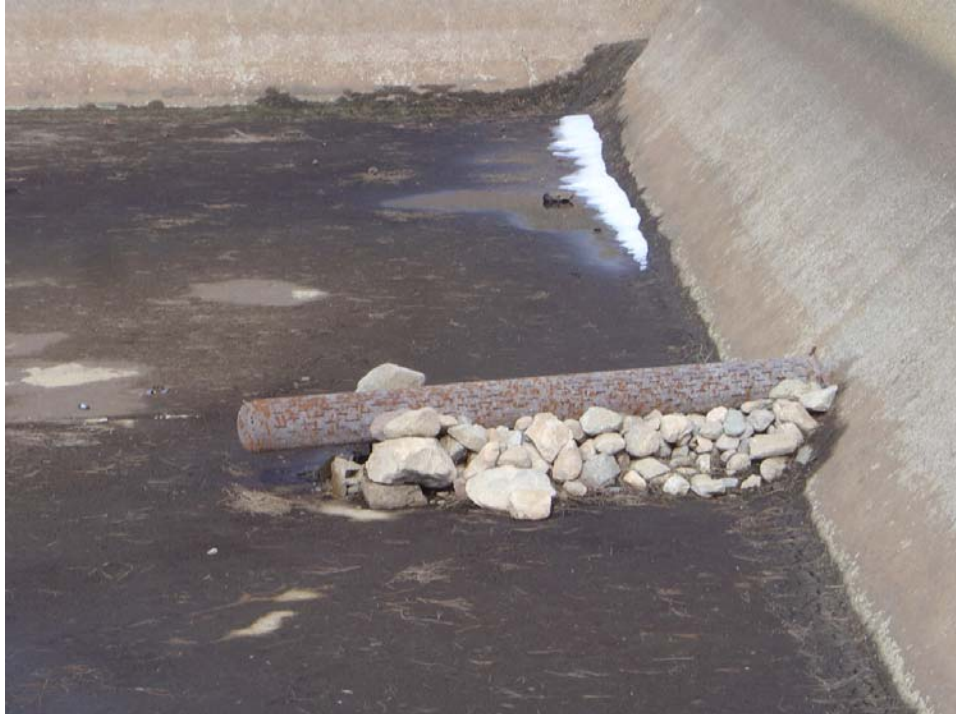
Marlette Lake / Ash Canyon – Building Index #2486 Description: Drain Outlet of 1 Million Gallon Storage Reservoir
