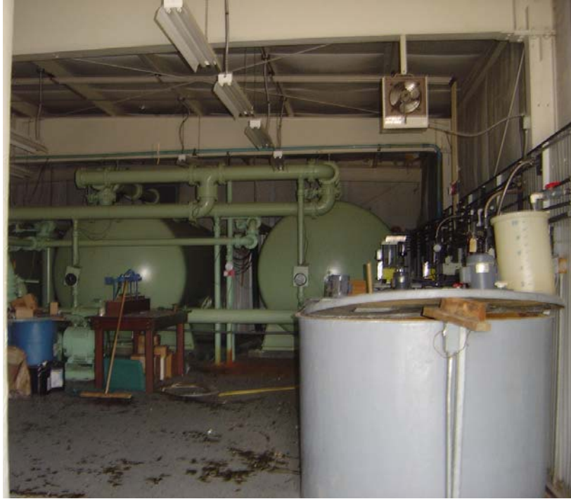
Marlette Lake / Ash Canyon – Building Index #2487 Description: Interior of Water Treatment Building; Rodent Droppings on Floor
