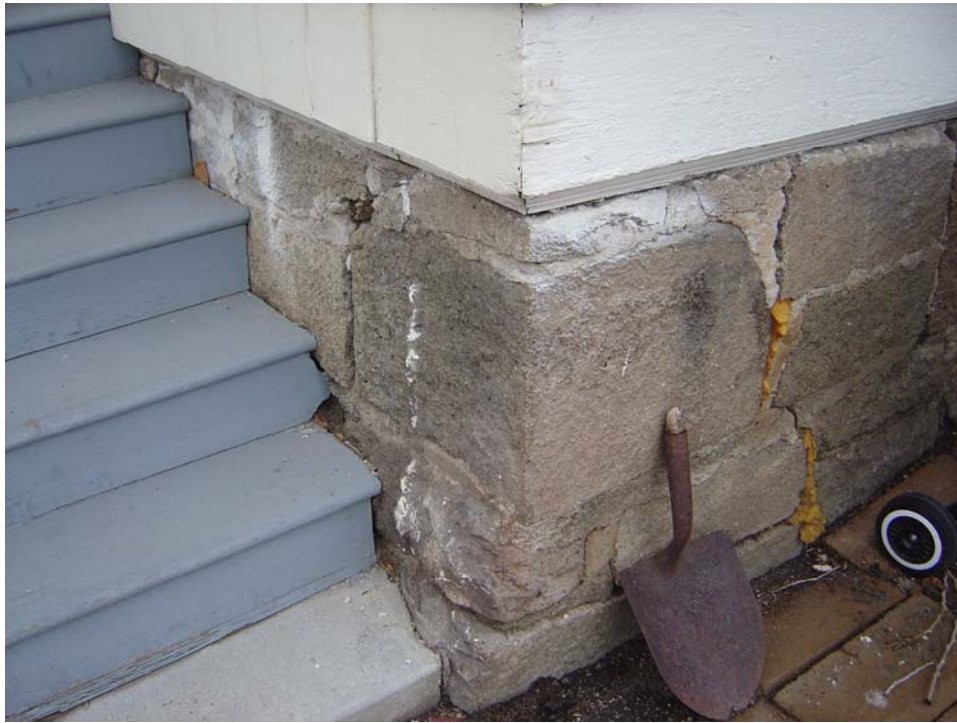
Marlette Lake Site – Building Number 2484 Description: Cracks in the foundation.
