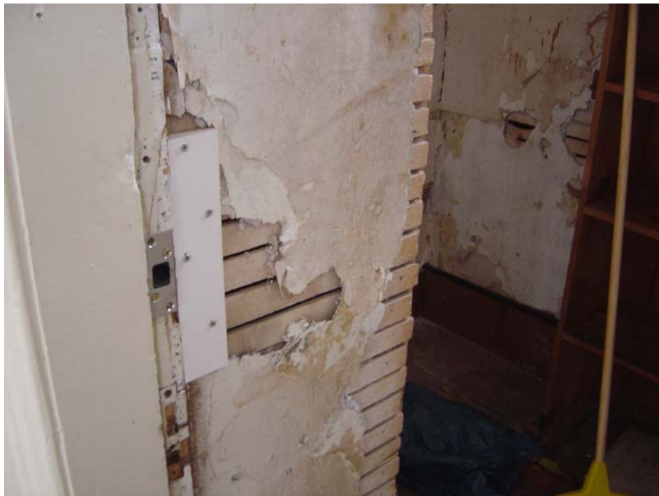
Marlette Lake Site – Building Number 2484 Description: Damage to wall at interior of pantry.
