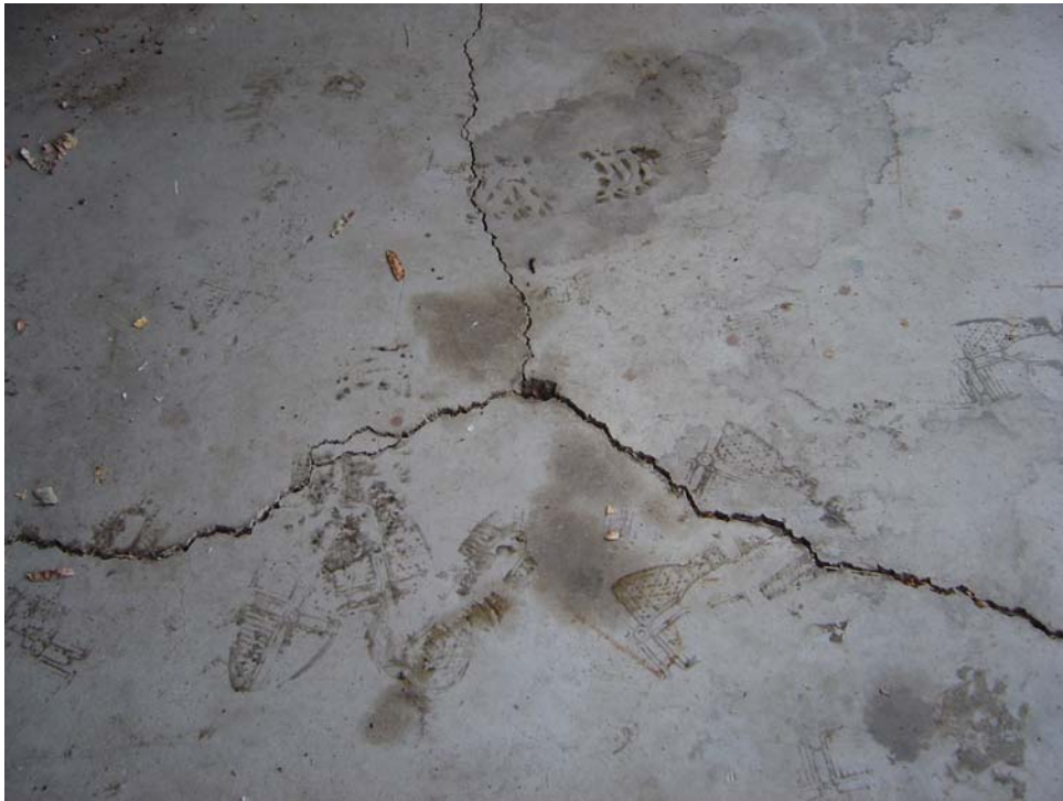
Marlette Lake Site - Building Number 2498 Description: Concrete spalling and cracking in equipment shed.
