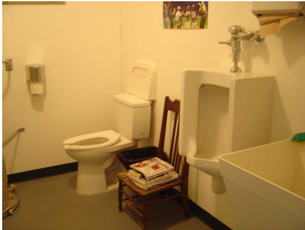
Marlette Lake Site - Building Number 2488 Description: Non-ADA compliant restroom in office.
