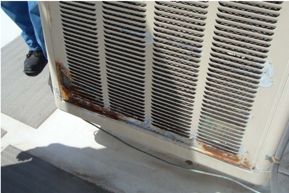
DMV Flamingo Office - Building #0338 Description: Roof mounted evaporative cooler.
