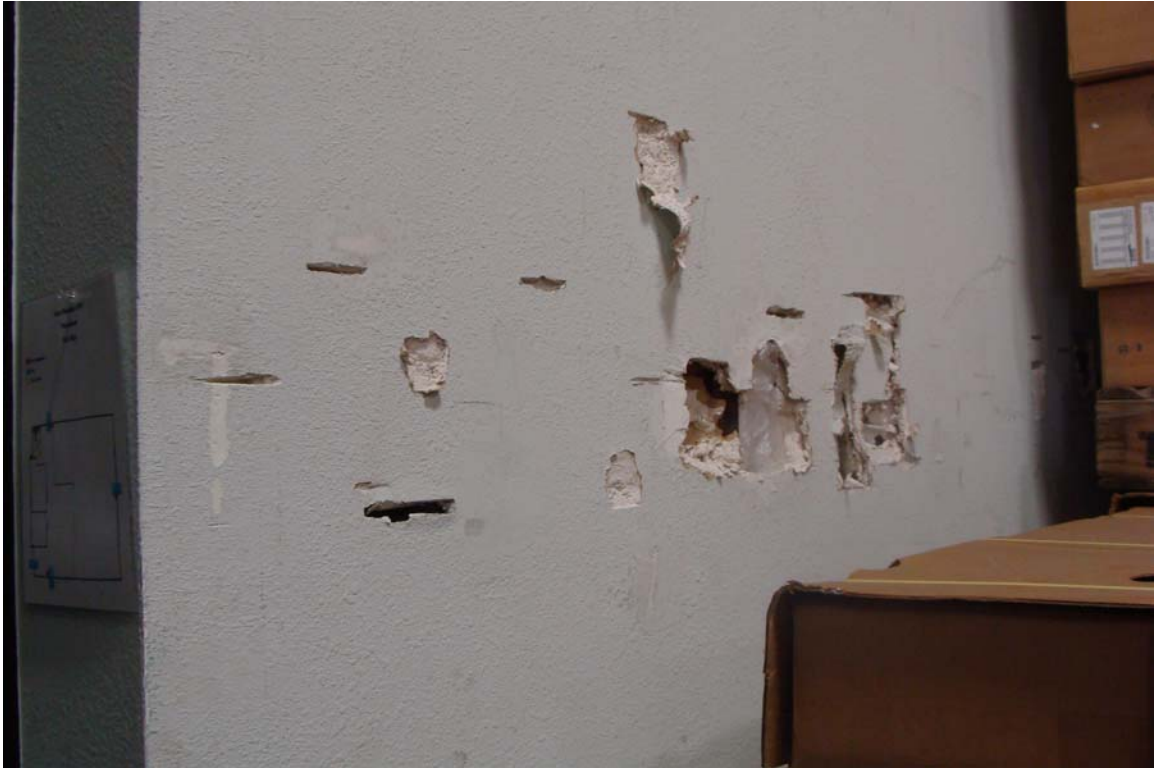
DMV Flamingo Warehouse - Building #0520 Description: Damaged gypsum board in the warehouse.
