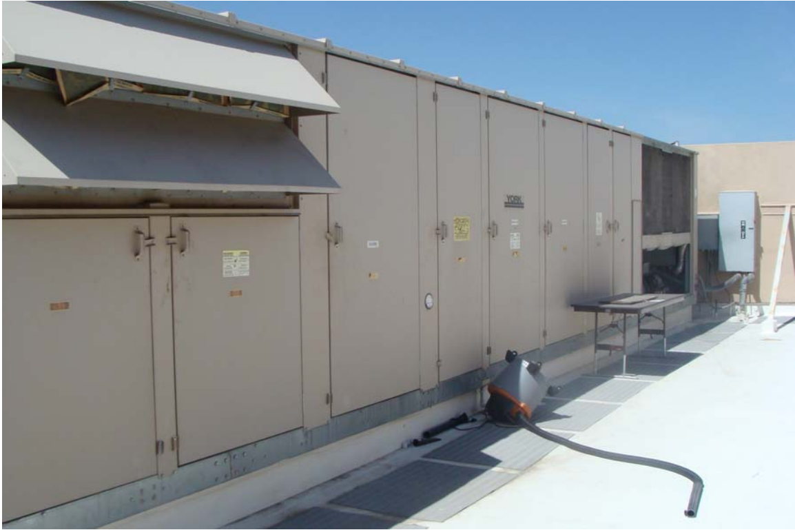
DMV Flamingo Office - Building #0338 Description: View of roof mounted HVAC unit.
