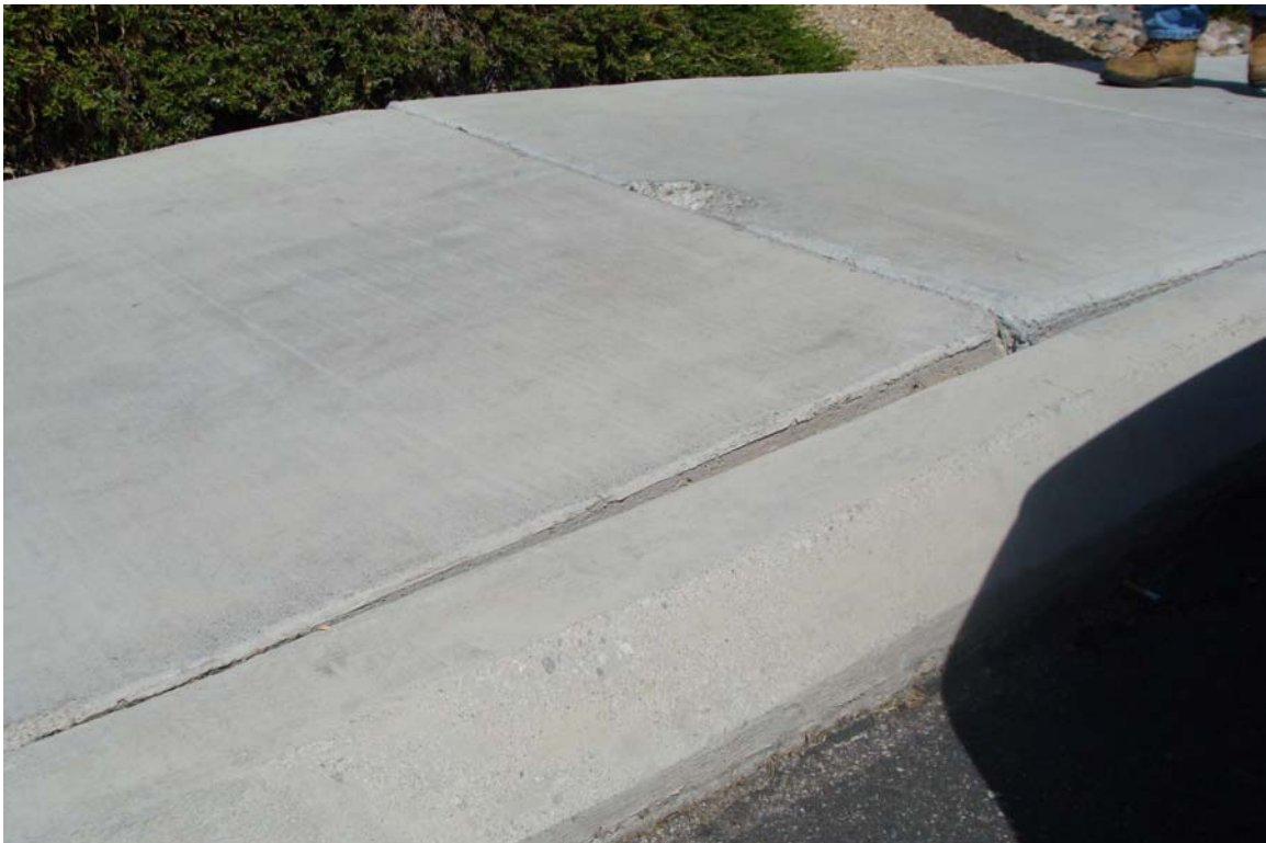
DMV Flamingo Road Site - Site #9901 Description: Heaving concrete at ADA accessible walkway.
