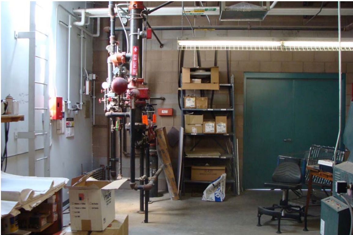
DMV Flamingo Office - Building #0338 Description: Fire sprinkler riser assembly.
