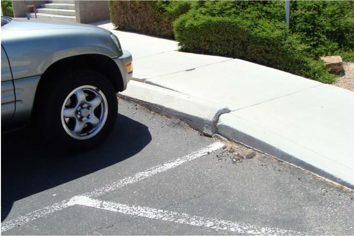
DMV Flamingo Road Site - Site #9901 Description: Damaged ADA accessible concrete walkway.
