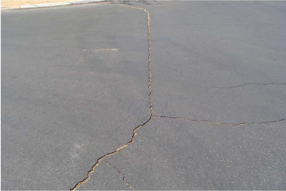
DMV Flamingo Road Site - Site #9901 Description: AC paving in need of crack filling and sealing.
