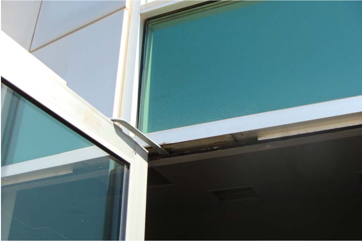
DMV Flamingo Office - Building #0338 Description: Storefront door that is leaking.
