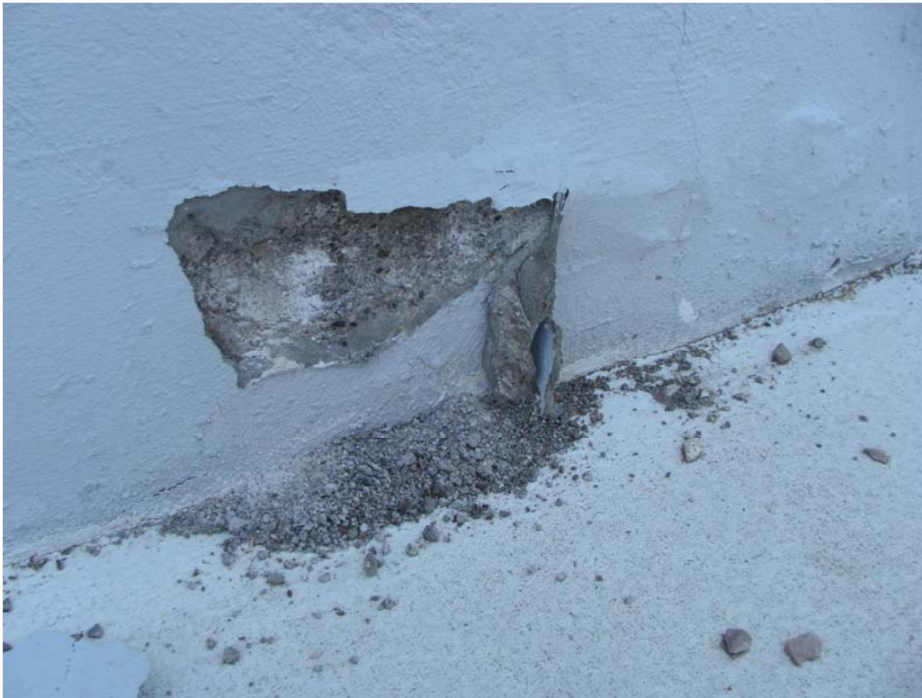
Field Office - Building #0633 Description: Damaged exterior plaster.
