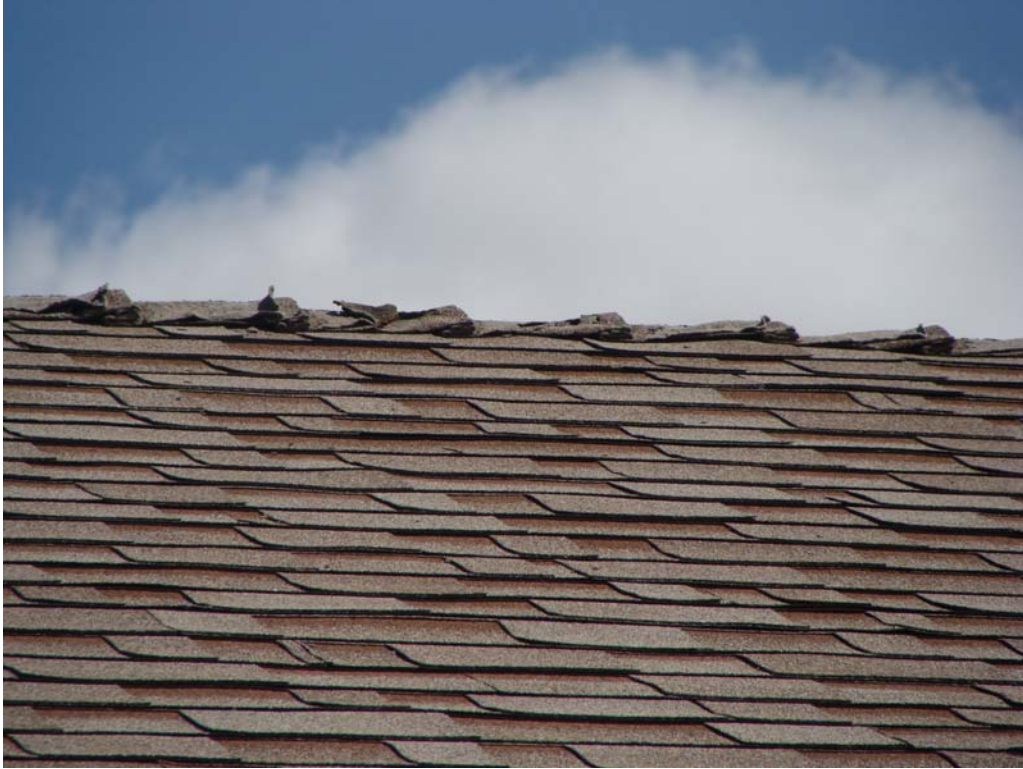
Field Office - Building #0633 Description: Damaged roof shingles.
