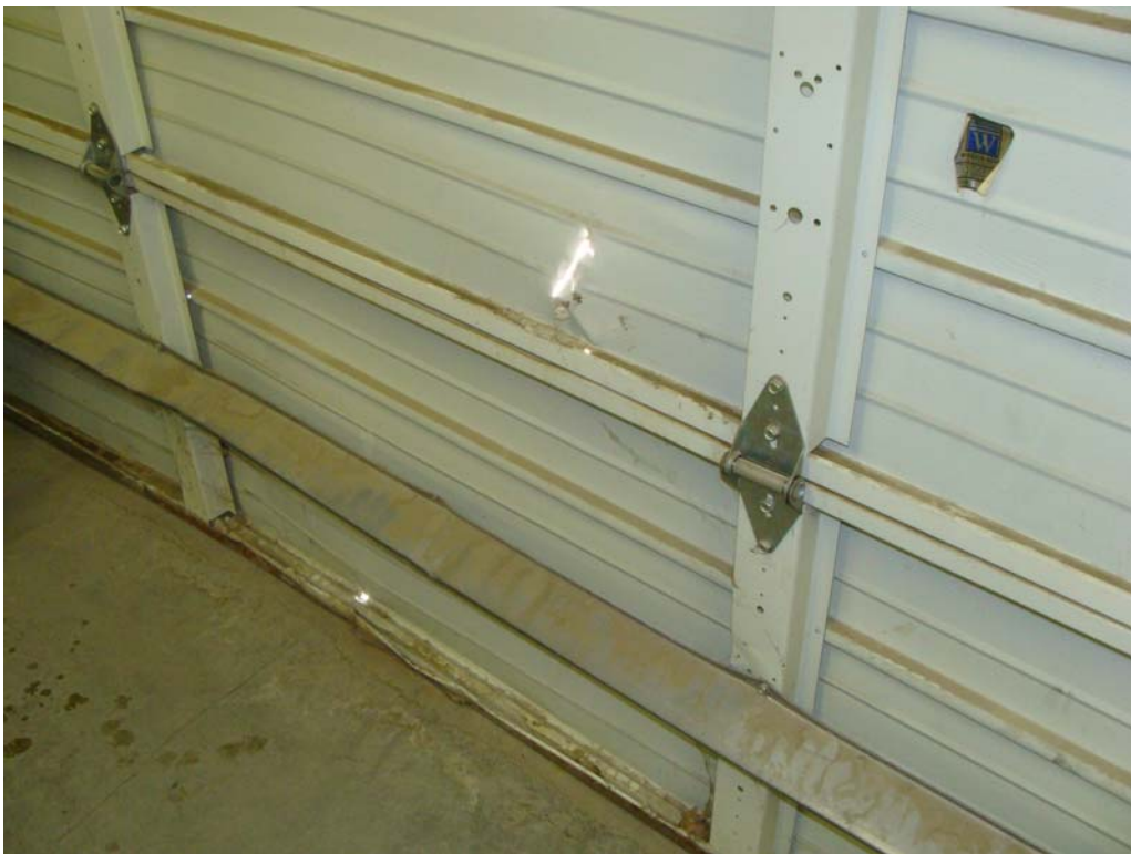
Boat Storage Facility - Building #1438 Description: Damaged overhead door.
