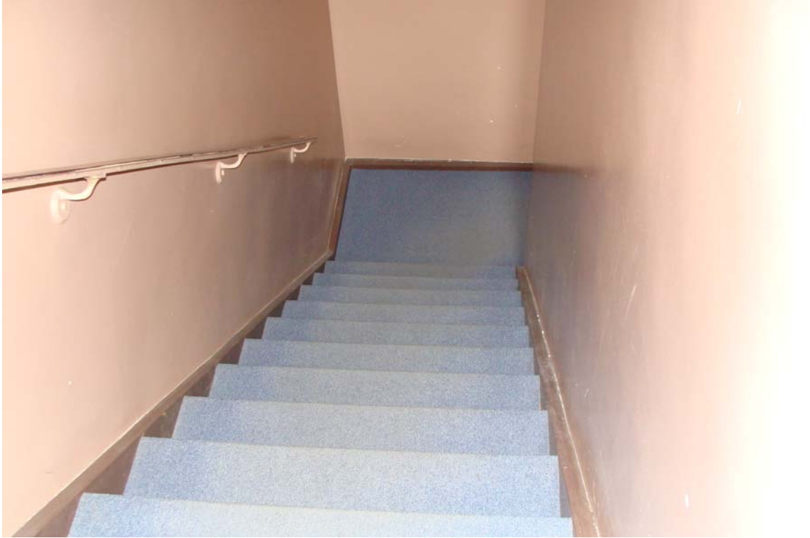
Nevada State Capitol - Building #0235 Description: Interior stairway handrails in need of upgrade.
