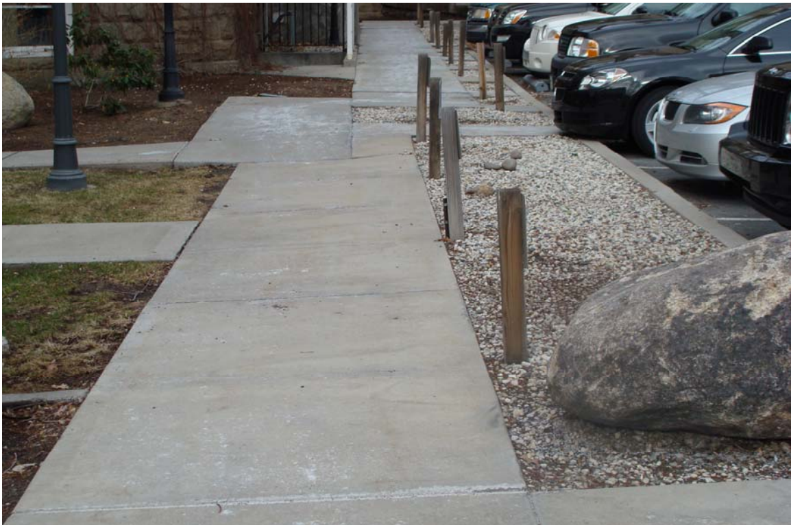
Nevada State Capitol - Site #9918 Description: ADA accessible route with cross slope exceeding 2%.
