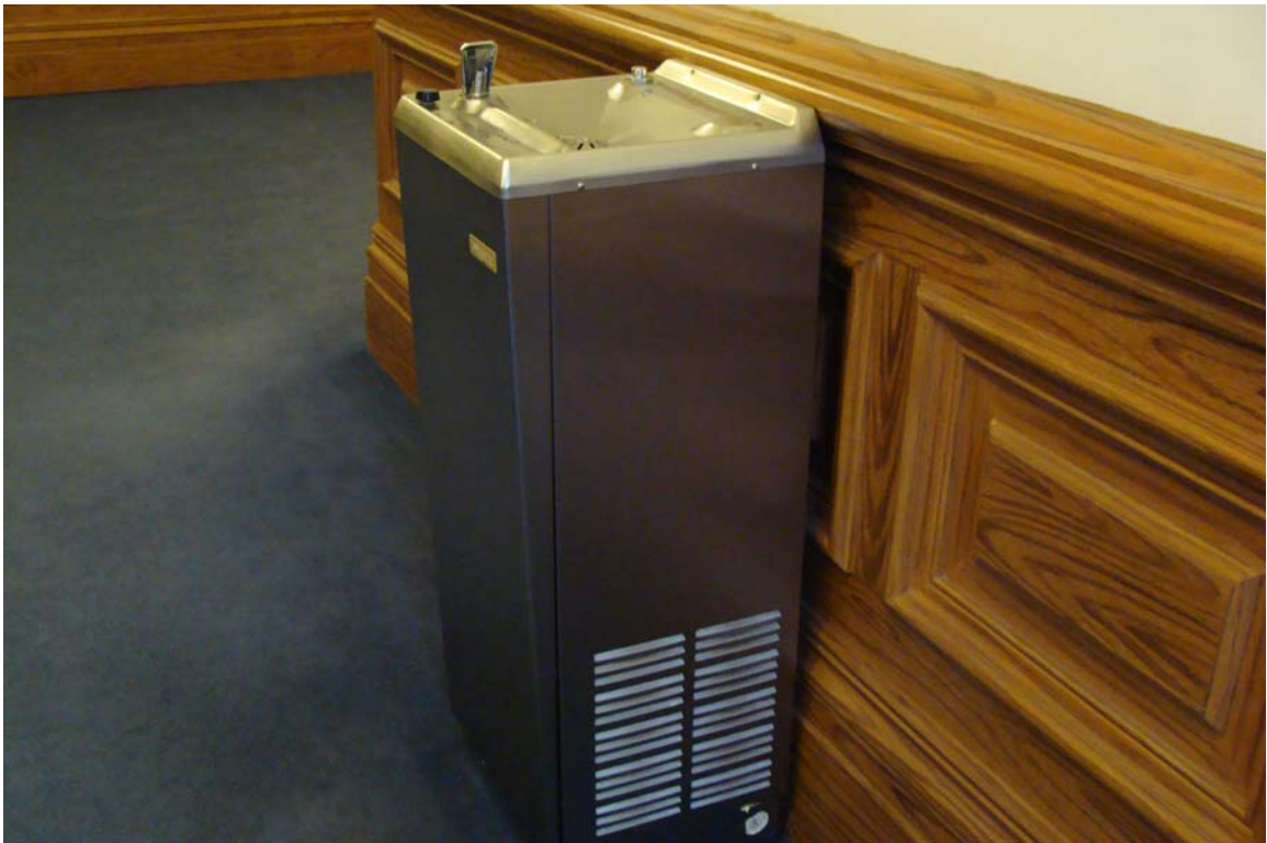
Nevada State Capitol - Building #0235 Description: Drinking fountain in need of replacement.
