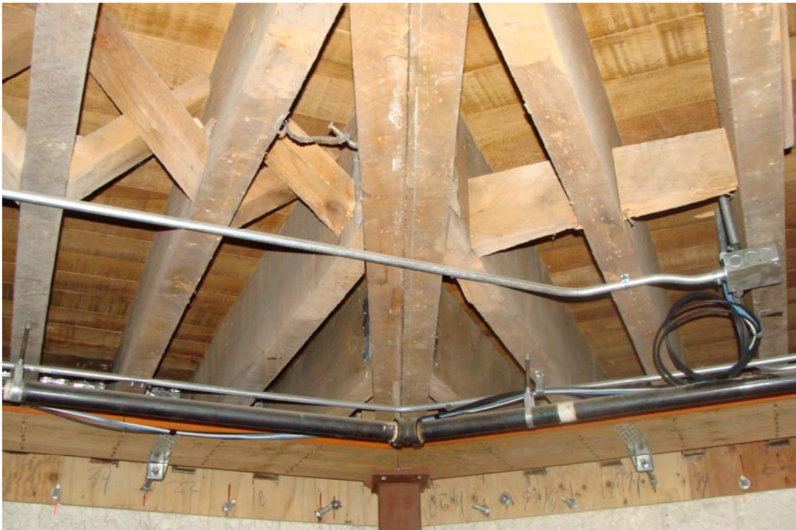
Nevada State Capitol Annex - Building #0203 Description: View of seismic retrofit completed in 2005.
