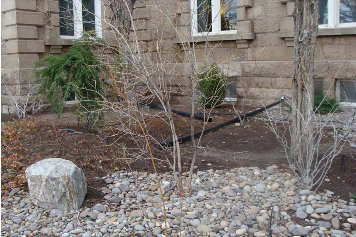
Nevada State Capitol - Site #9918 Description: Area in need of drainage improvements.
