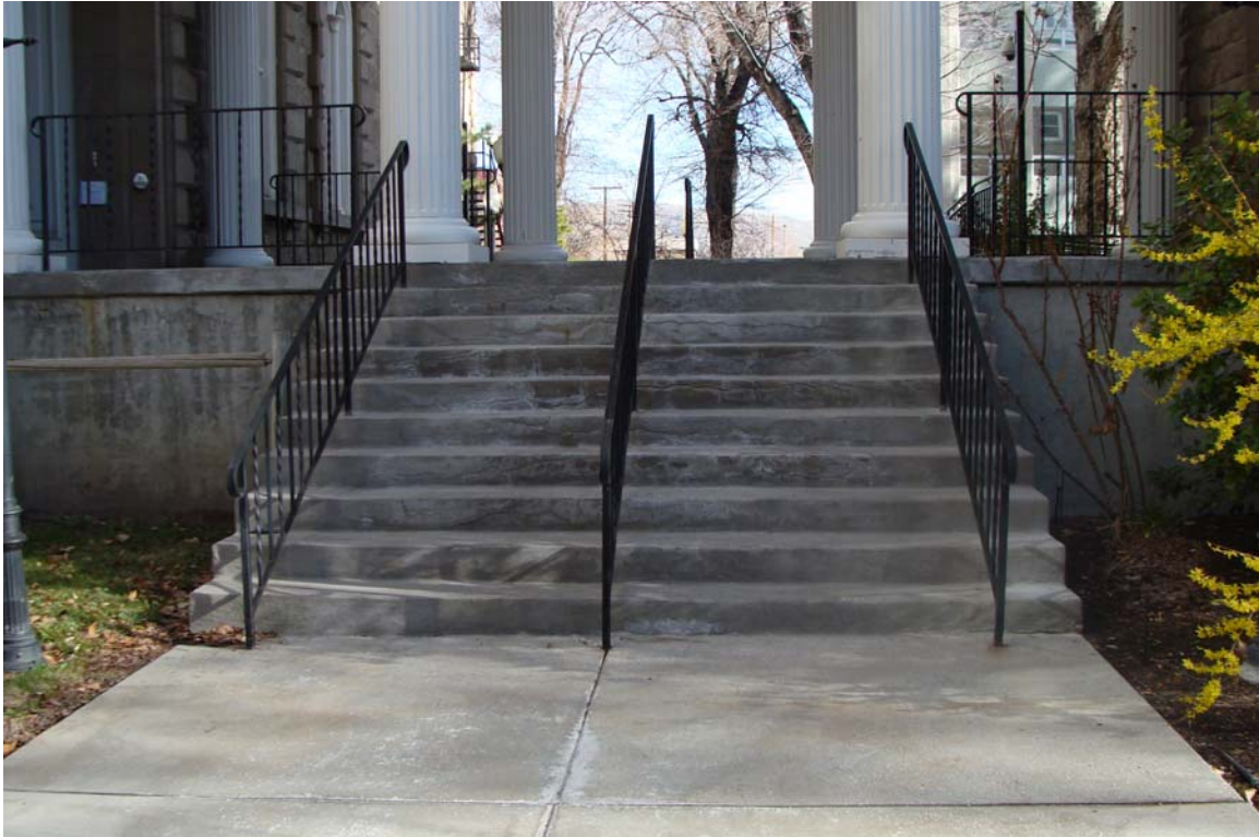
Nevada State Capitol - Site #9918 Description: Stairs / rails in need of replacement.
