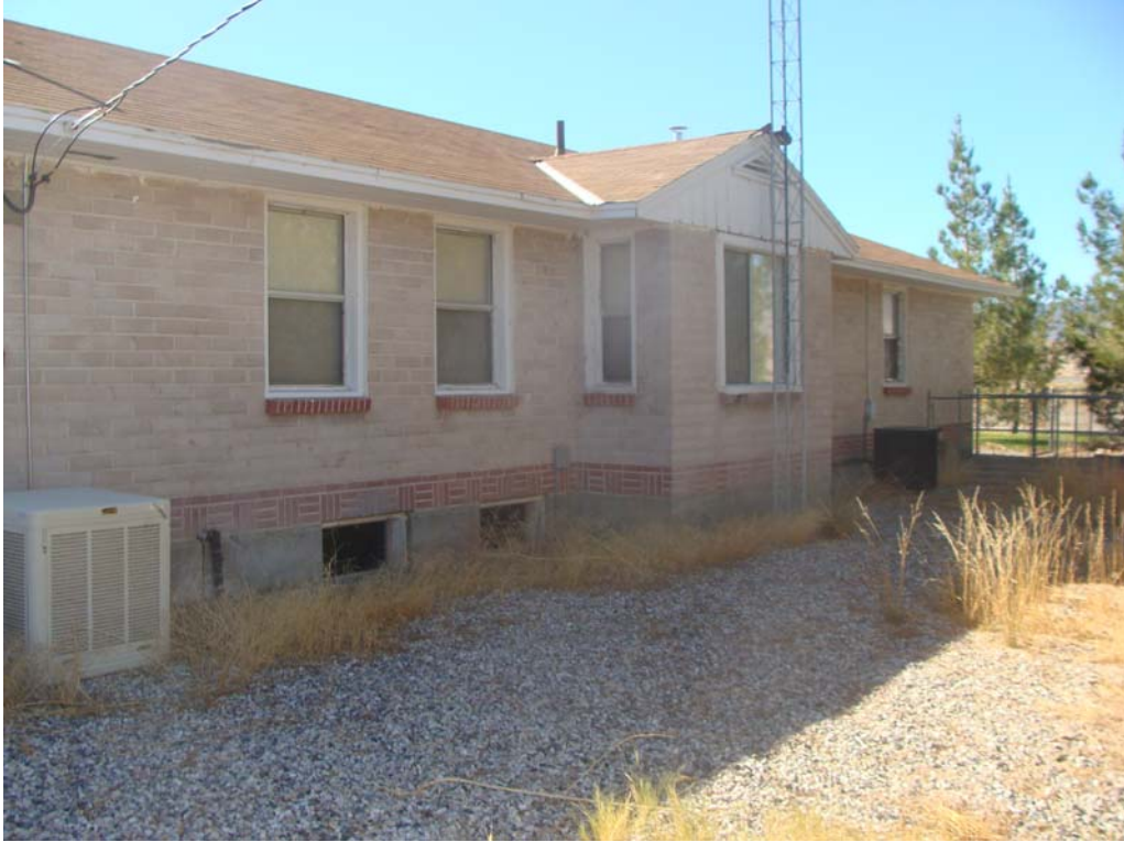
WMA Supervisor's Residence - Building #0903 Description: Area in need of drainage improvements.
