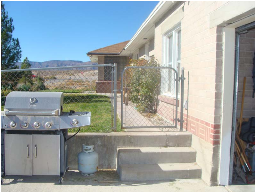
WMA Supervisor's Residence - Building #0903 Description: Stairs in need of handrails.
