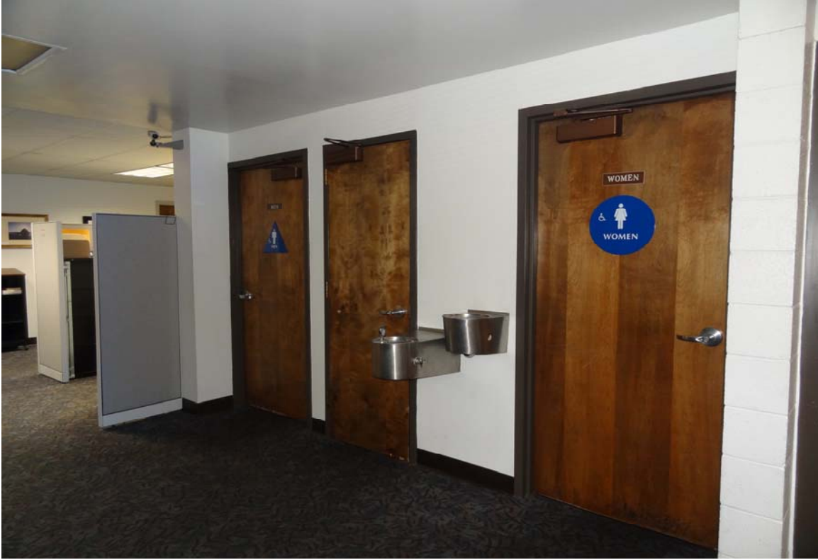
Lakes Crossing Center - Building #0342 Description: Non-ADA compliant staff restroom entrances.
