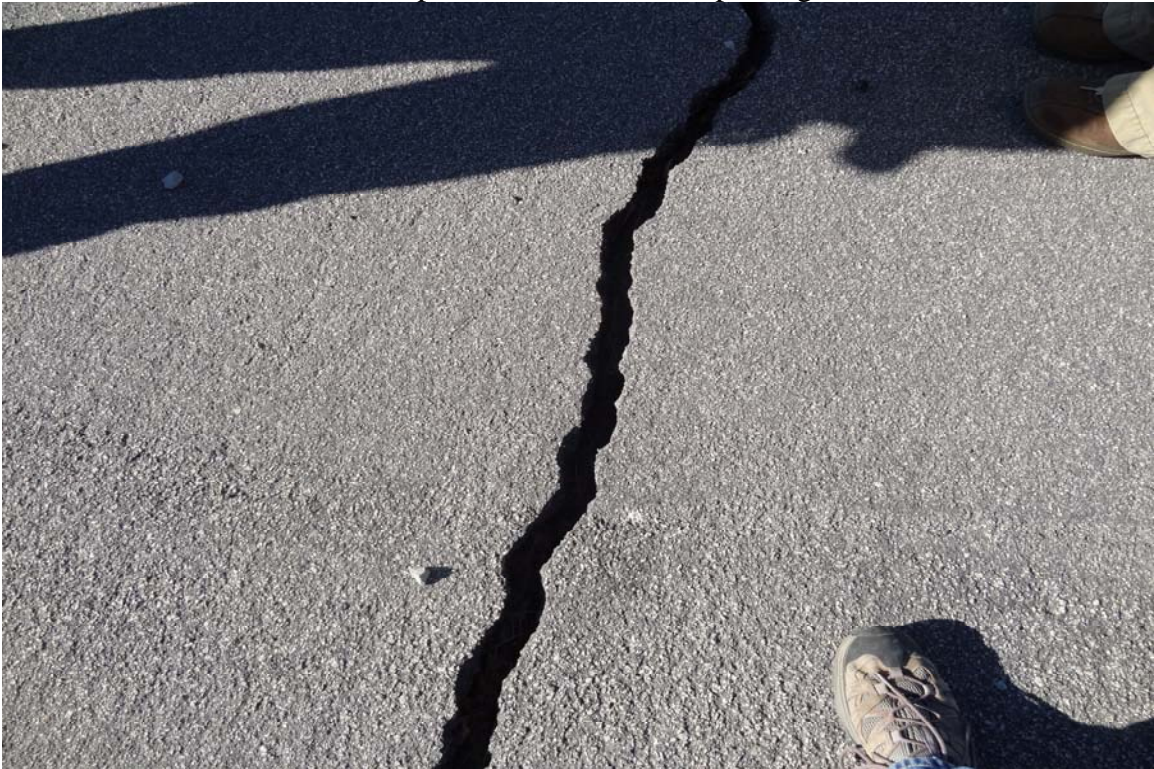
Lakes Crossing Center Site - Site #9980 Description: Access road pavement in need of crack filling.
