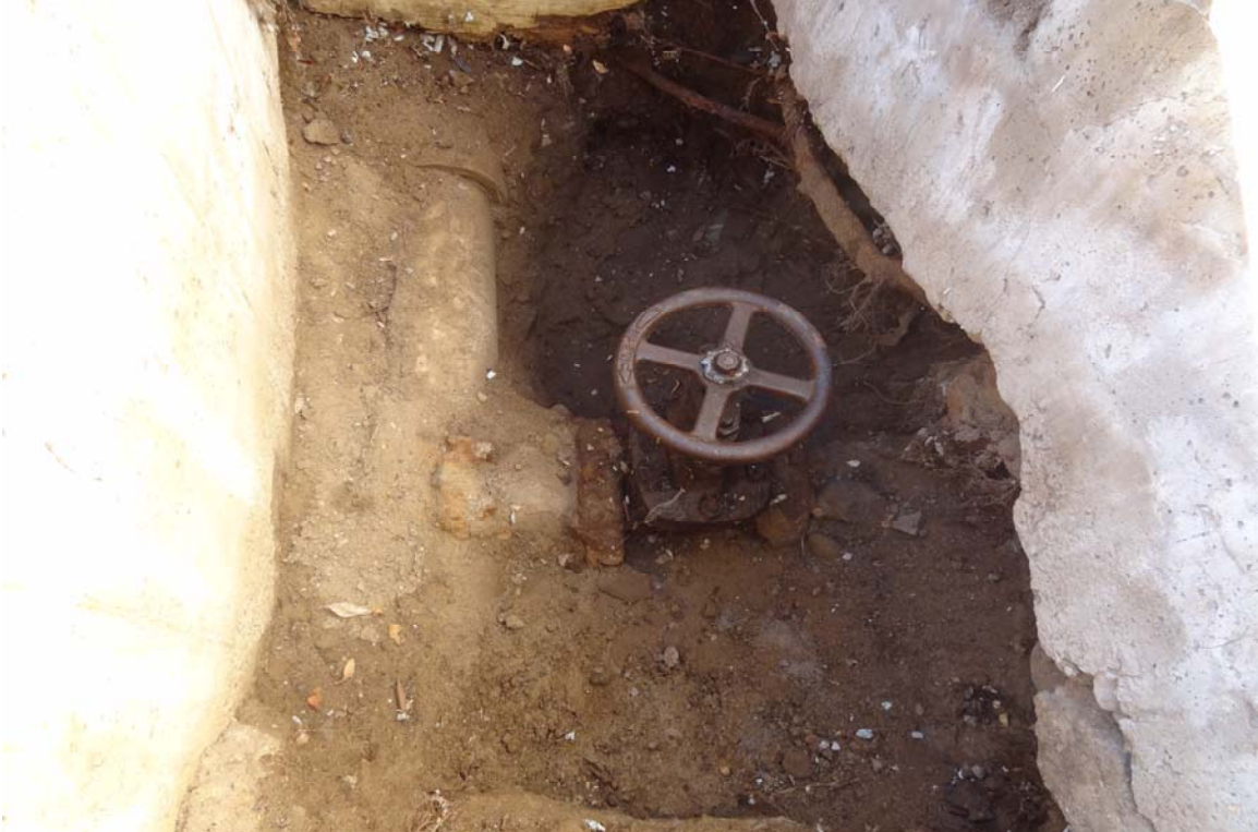
Lakes Crossing Center - Building #0342 Description: View of leaking irrigation gate valve.
