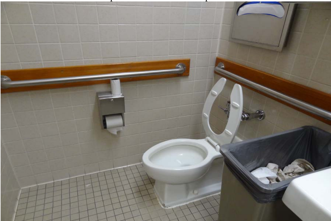
Lakes Crossing Center - Building #0342 Description: Non-ADA compliant staff Men's restroom.
