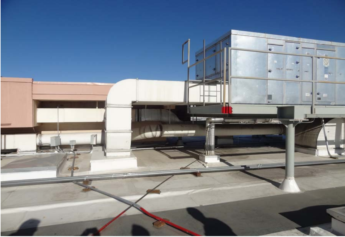
Lakes Crossing Center - Building #0342 Description: View of the roof mounted HVAC unit.
