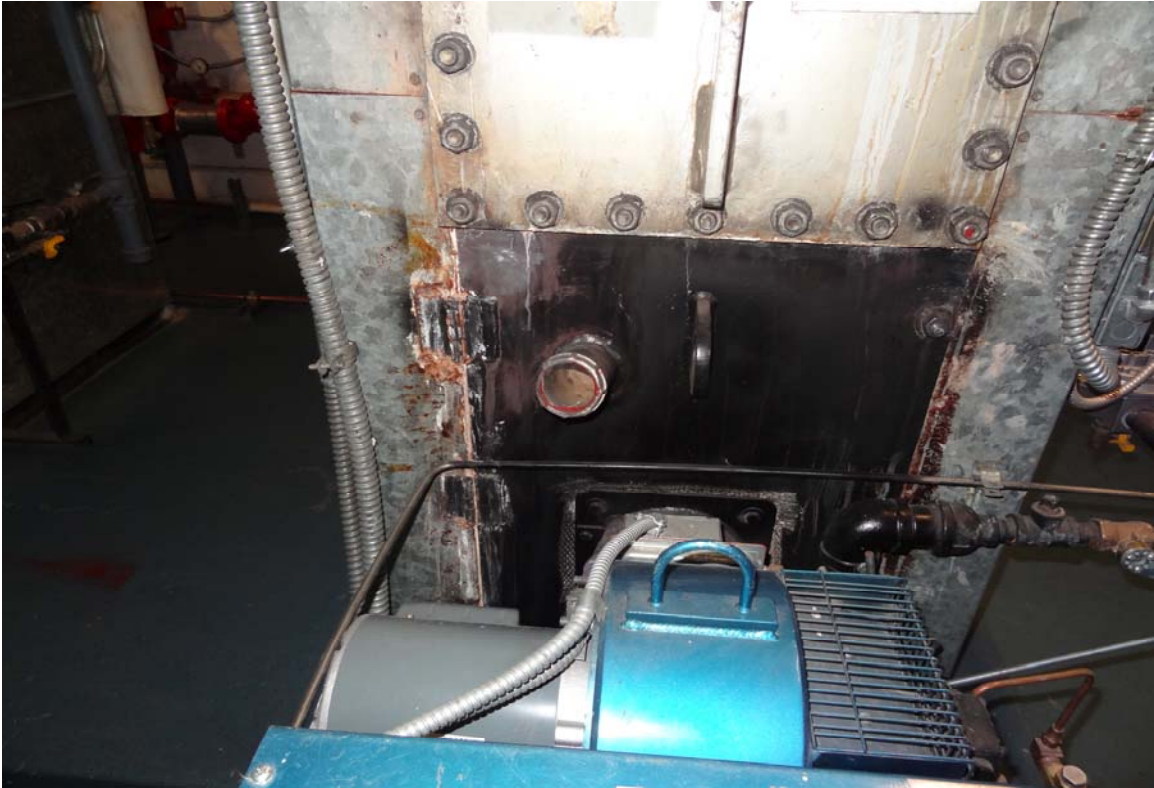
Lakes Crossing Center - Building #0342 Description: Boiler in need of replacement.
