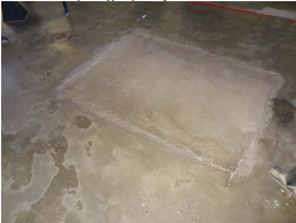
Housing Unit #8 – FCA Building #1481 Description: One of several areas of concrete removal and replacement to access clogged sewer piping.
