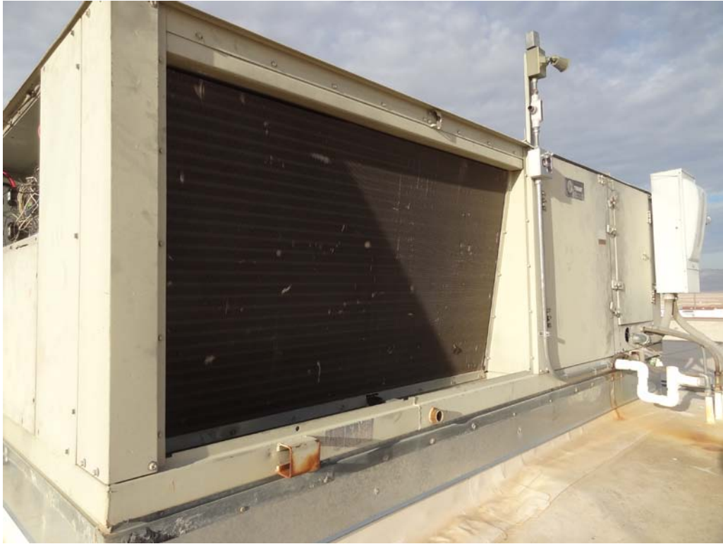
Housing Unit #8 – FCA Building #1481 Description: 30 year old HVAC equipment.
