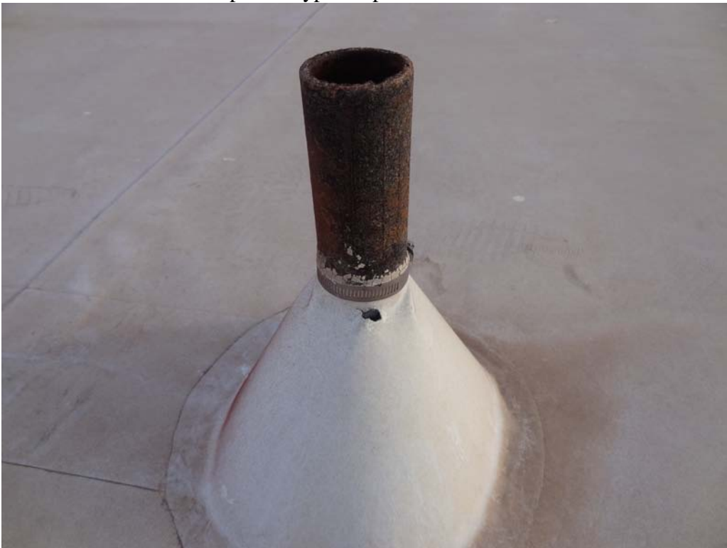
Housing Unit #8 – FCA Building #1481 Description: Typical roof penetration with deteriorated sealants and punctures in the membrane.
