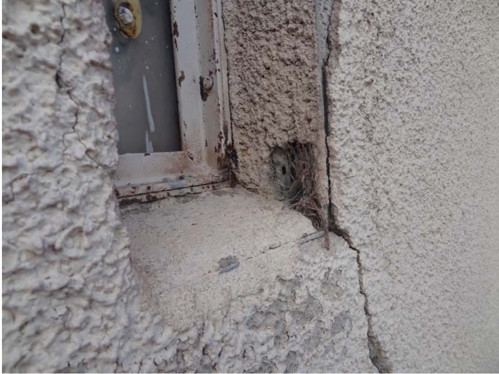
Housing Unit #8 – FCA Building #1481 Description: Damage to exterior finishes.
