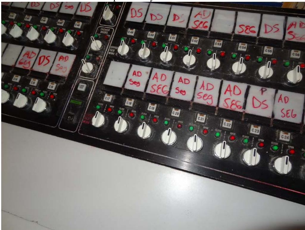
Housing Unit #8 – FCA Building #1481 Description: 30 year old cell door control panel.
