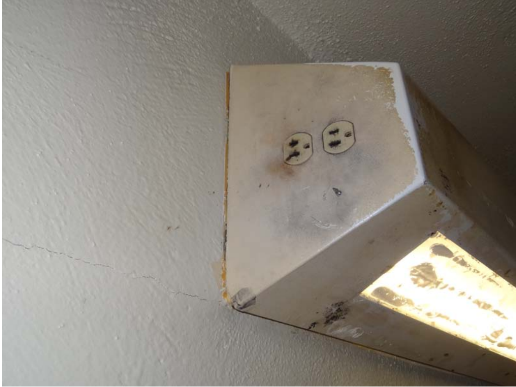
Housing Unit #8 – FCA Building #1481 Description: Typical lighting and electrical in cells.
