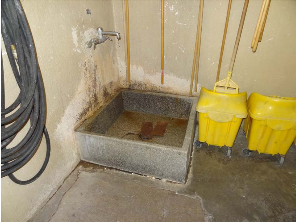
Housing Unit #8 – FCA Building #1481 Description: Cracked mop sink and damaged interior finishes.
