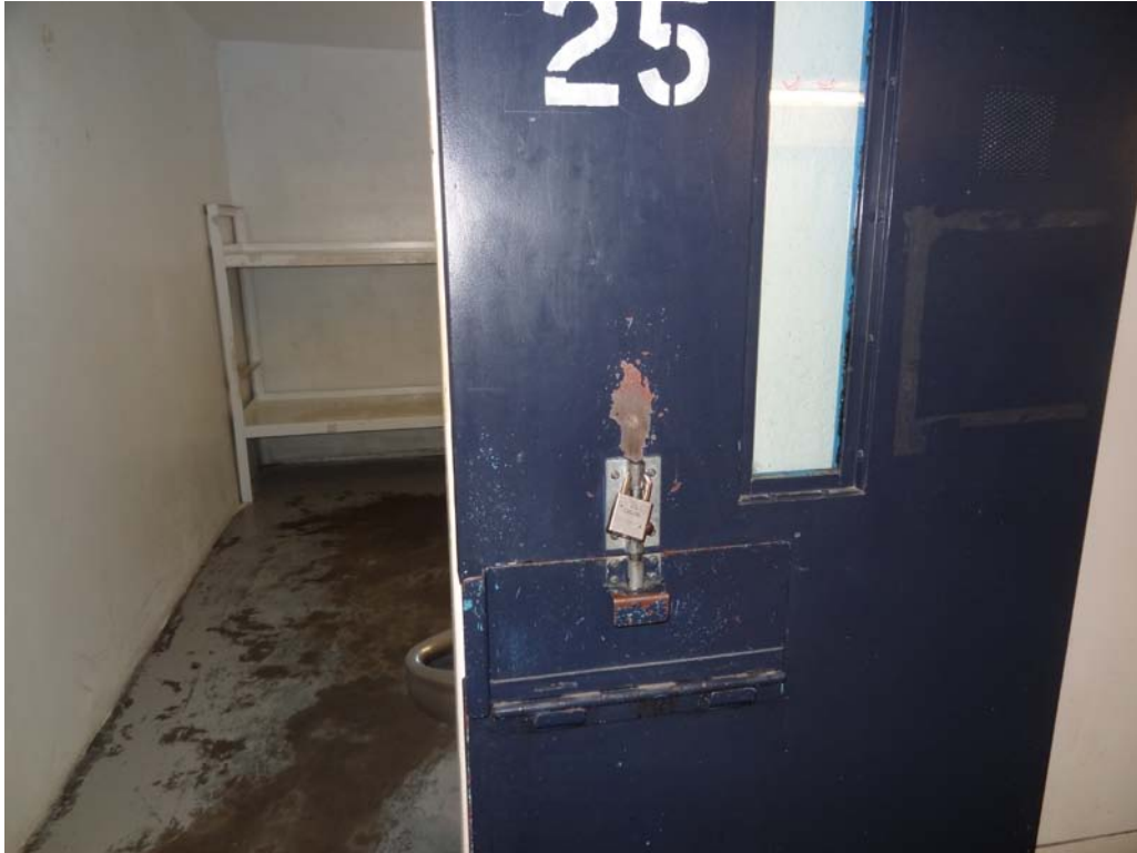
Housing Unit #8 – FCA Building #1481 Description: 30 year old cell door.
