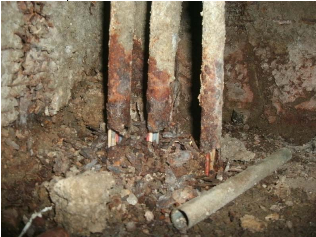
Housing Unit #8 – FCA Building #1481 Description: Rusted electrical conduit in utility chase.
