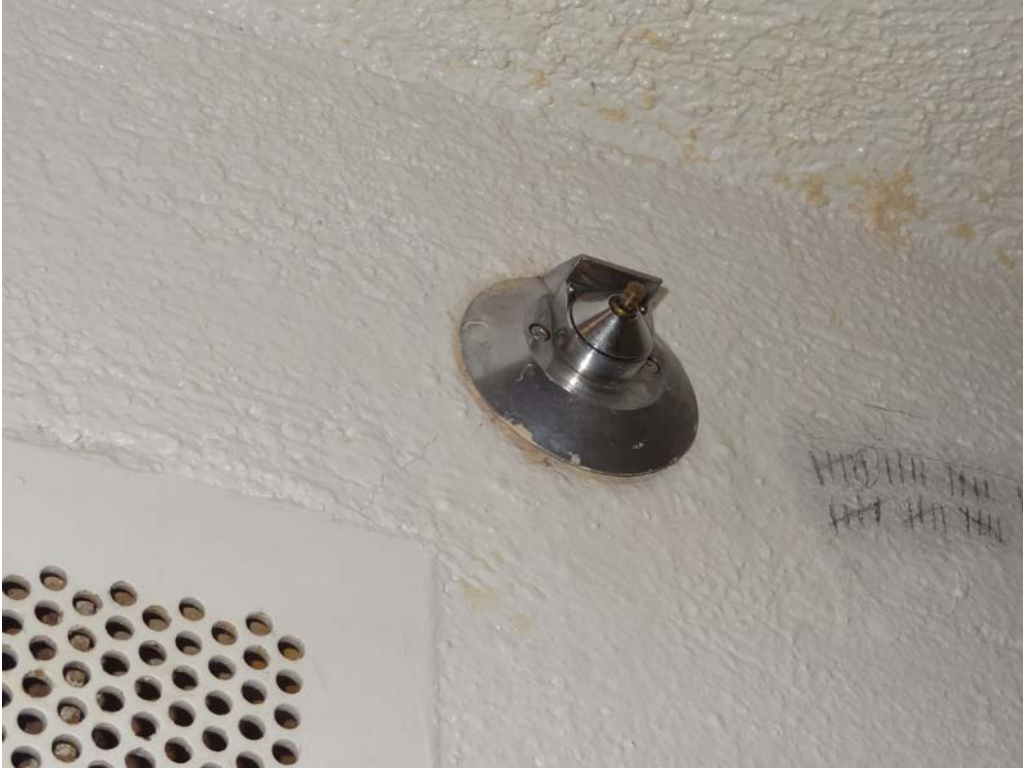
Housing Unit #8 – FCA Building #1481 Description: Typical sprinkler head in cell.
