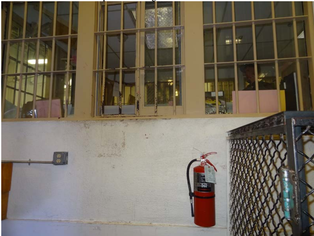
Housing Unit #8 – FCA Building #1481 Description: Damage to interior finishes.
