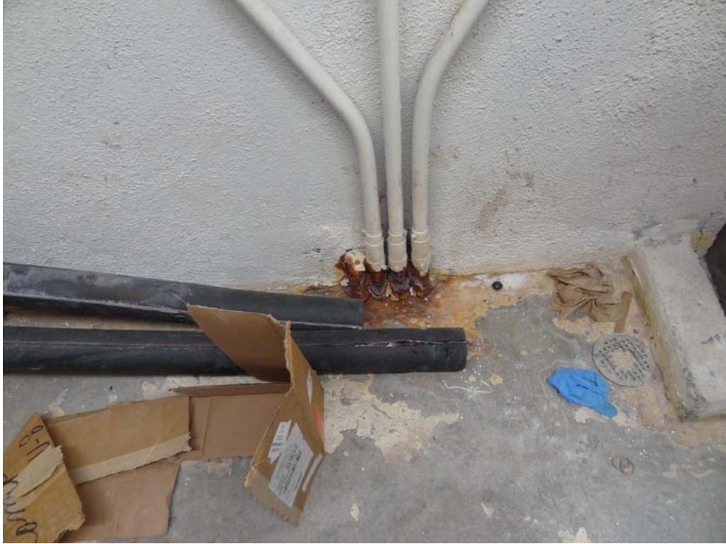
Housing Unit #8 – FCA Building #1481 Description: Rusted electrical conduit in Mechanical Room.
