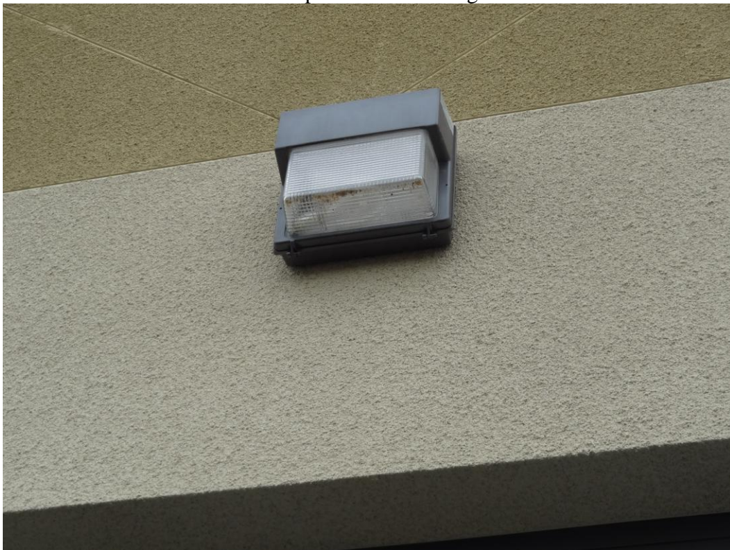
Fleet Services – Las Vegas – FCA Building #3155 Description: Exterior Wall Pack Light Fixtures
