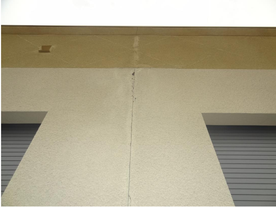
Fleet Services – Las Vegas – FCA Building #3155 Description: EIFS Damage
