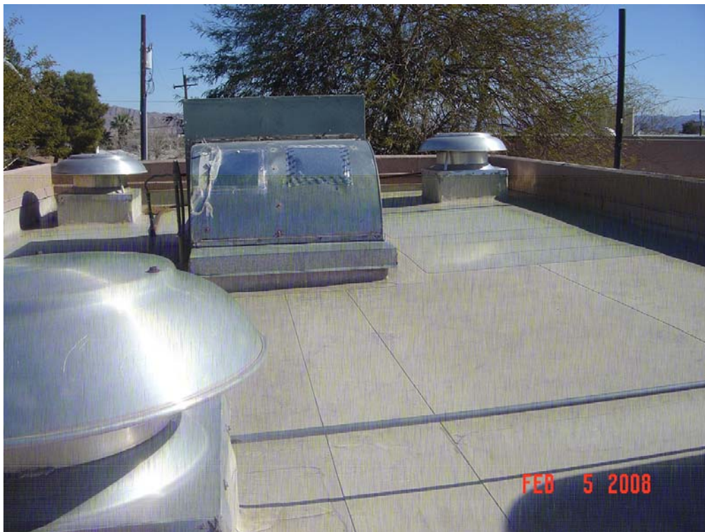
Agriculture Office - Building #0418 Description: Roof top equipment.
