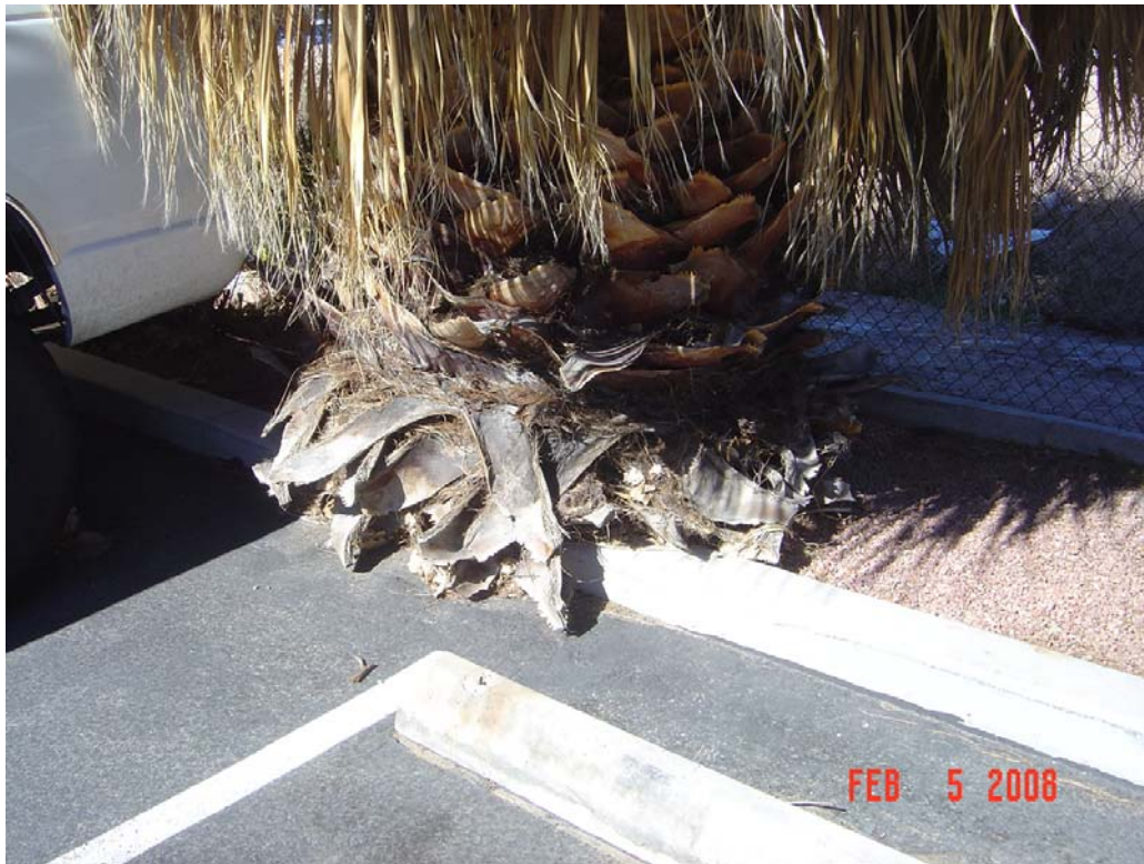
Agriculture Site - Site #9818 Description: Curb damage from palm tree.
