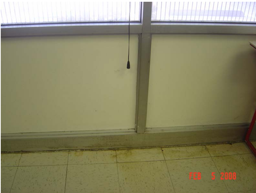
Agriculture Office - Building #0418 Description: Single pane window system.
