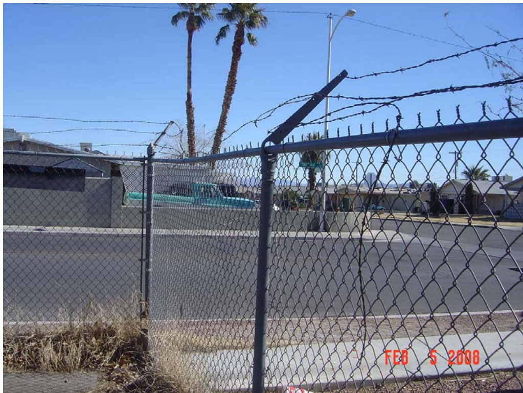
Agriculture - Site #9818 Description: Damaged perimeter fencing.
