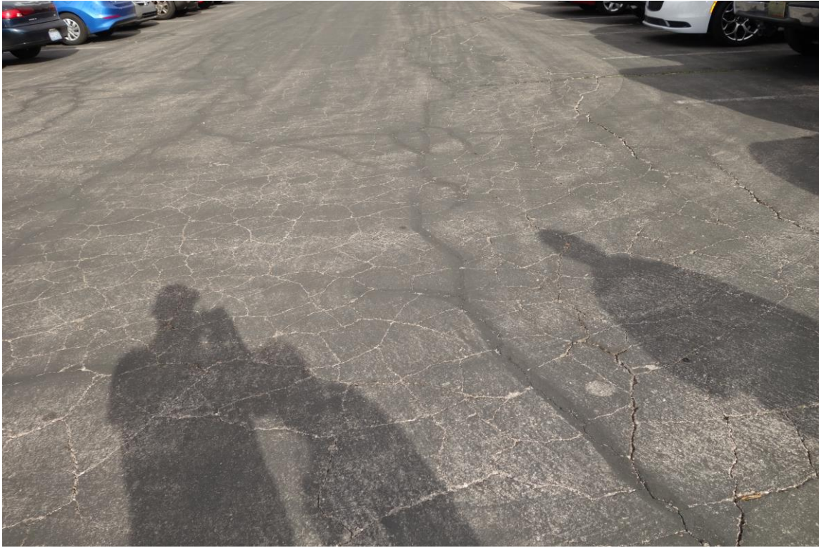
Belrose Office Building Site - Site #9831 Description: Damaged Paving in West Parking Area Needing Replacement.
