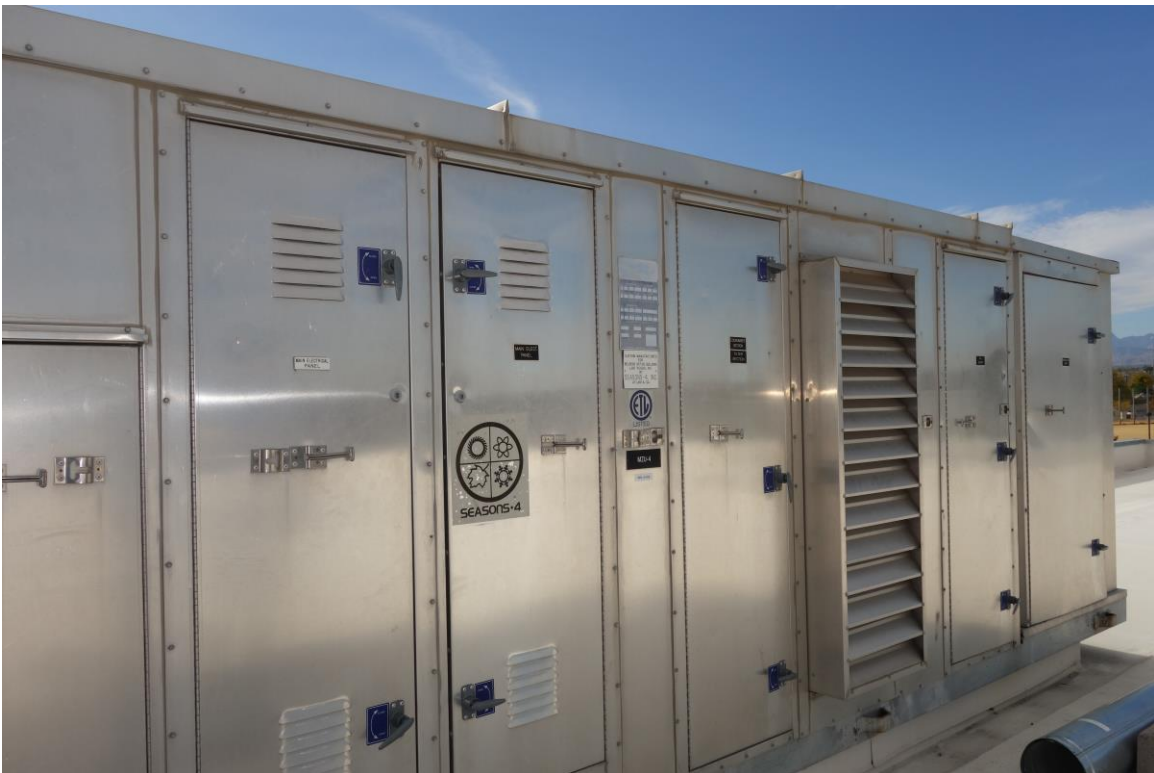
Belrose Office Building - Building #0286 Description: HVAC Equipment Replacement.
