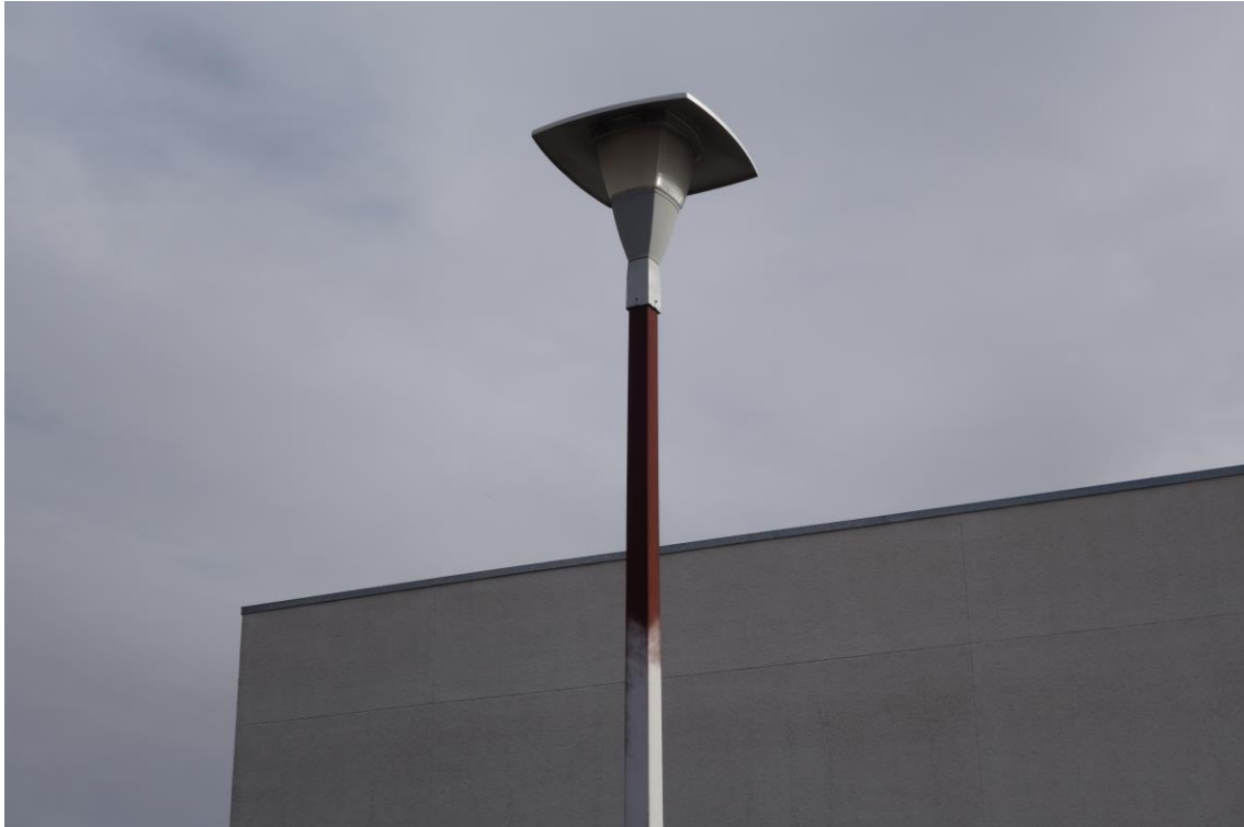
Belrose Office Building Site - Site #9831 Description: Exterior Site Lighting Upgrade Needed.
