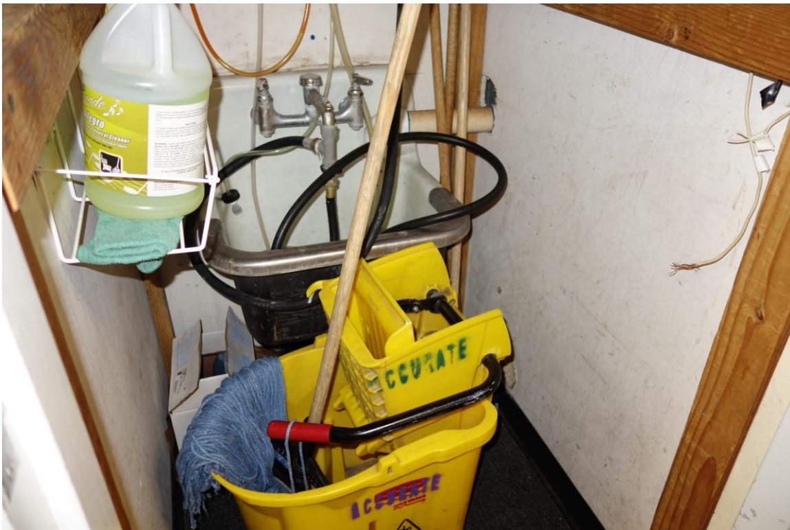
Belrose Office Building - Building #0286 Description: Janitor's Closet Upgrades Needed.
