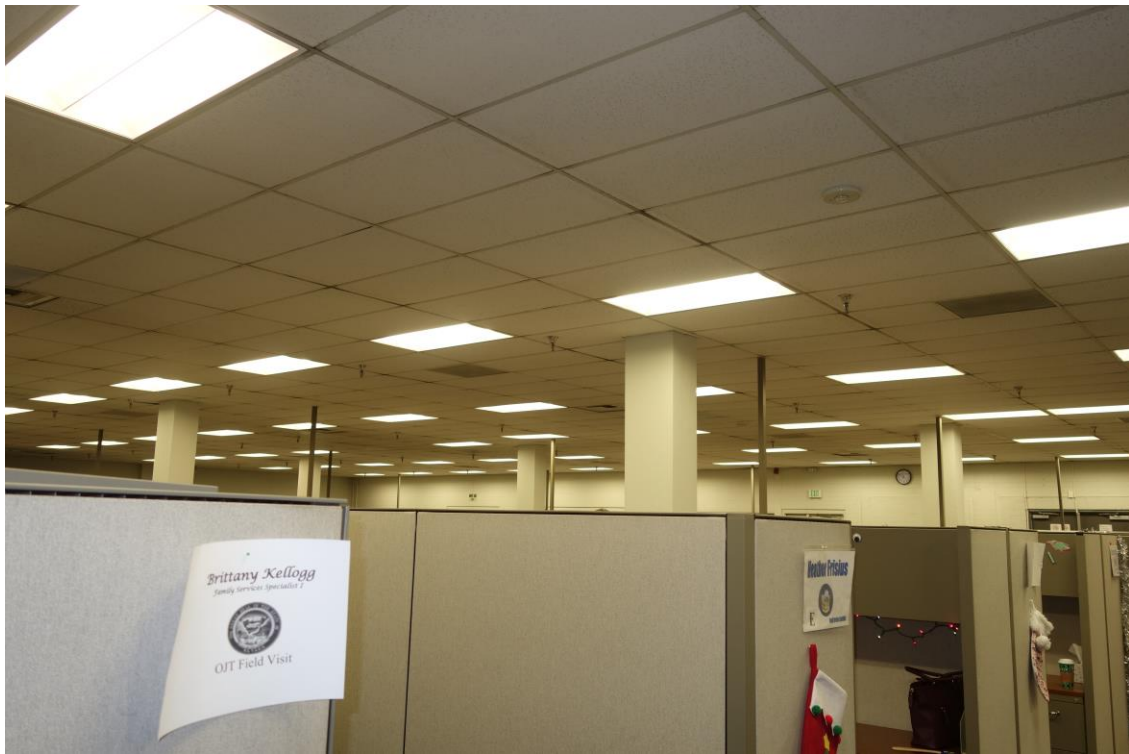
Belrose Office Building - Building #0286 Description: Suspended Ceiling and Lighting Upgrade Needed.
