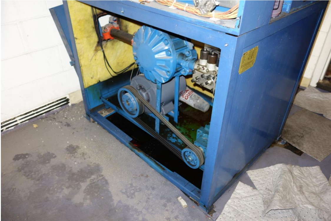
Belrose Office Building - Building #0286 Description: Elevators in Need of Replacement.
