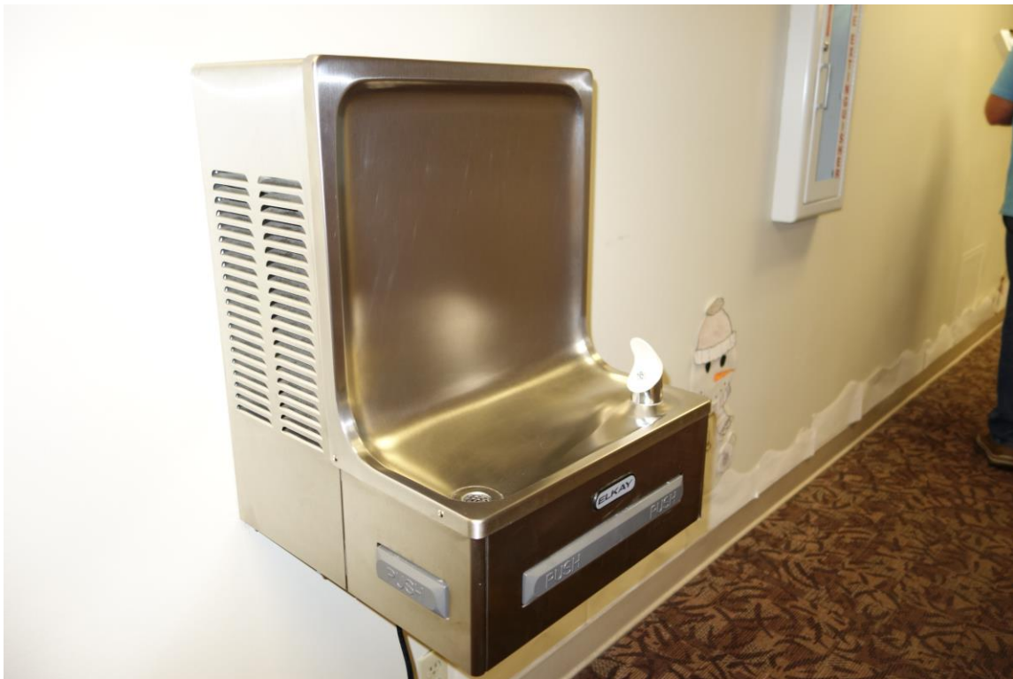
Belrose Office Building - Building #0286 Description: Dual Level Drinking Fountains Needed.
