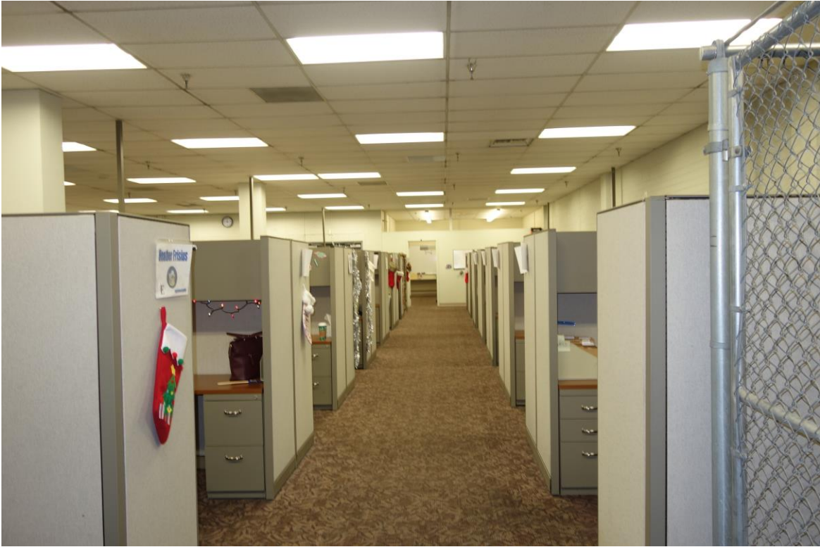
Belrose Office Building - Building #0286 Description: Flooring Replacement Needed.
