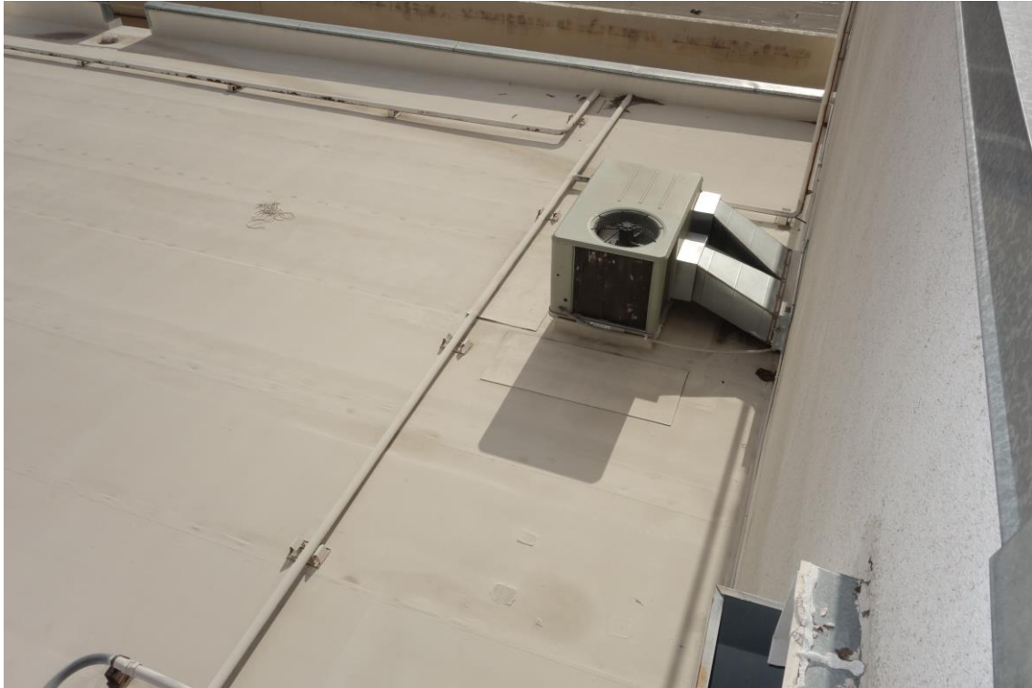
Belrose Office Building - Building #0286 Description: Roof Replacement Needed.
