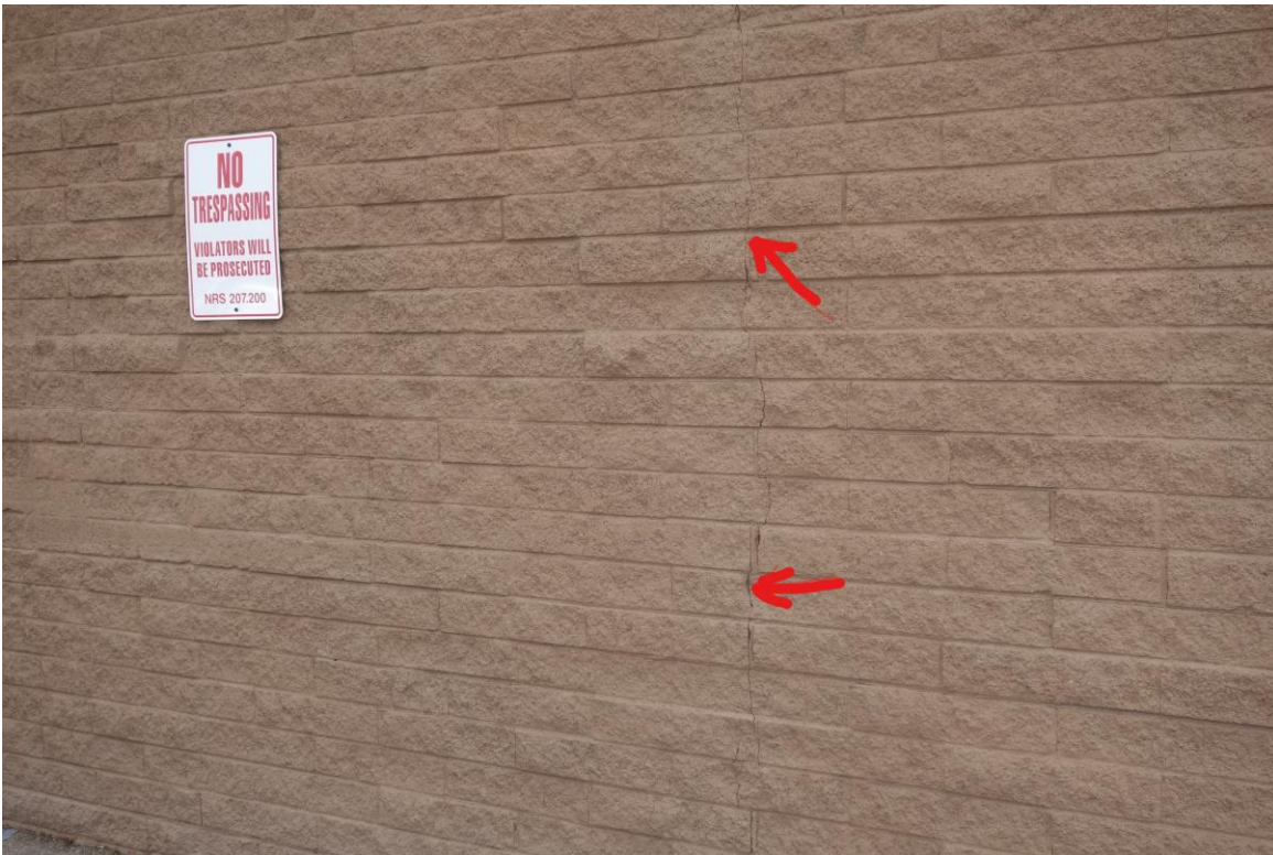
Belrose Office Building - Building #0286 Description: CMU Wall Crack in West Exterior Wall.
