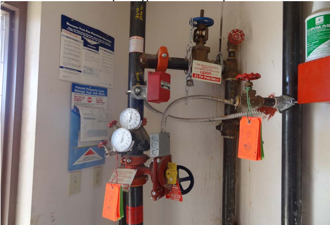
DMV Express Office - Building #0265 Description: Fire sprinkler riser.
