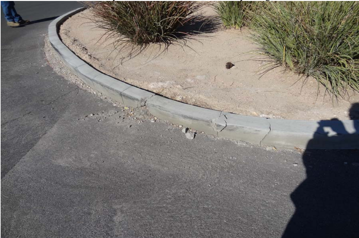
DMV Express Office Site - Site #9832 Description: Damaged curb at entrance to parking area.
