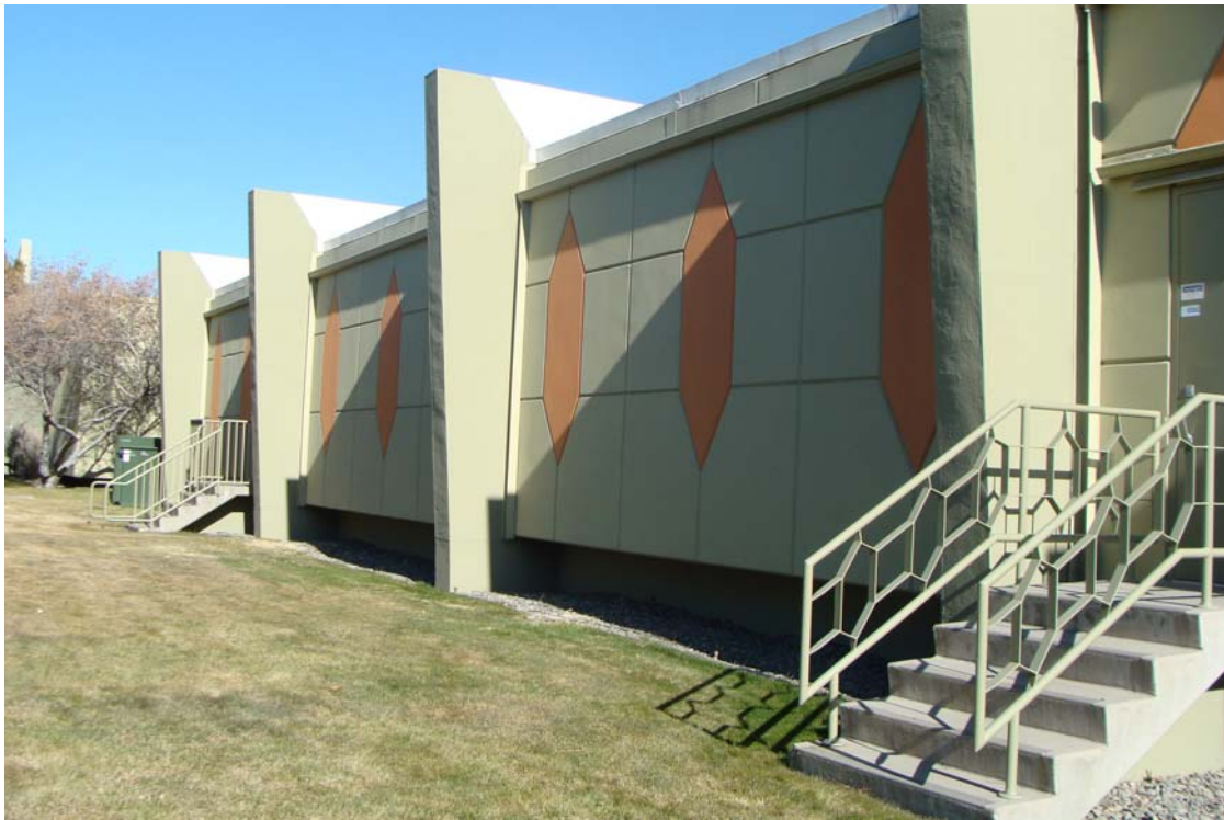
Nevada Historical Society - Building #0401 Description: Exit stairs in need of a landing.
