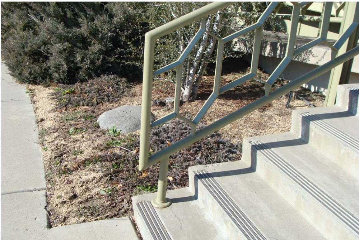
Nevada Historical Society - Building #0401 Description: Non compliant stairs and handrails.
