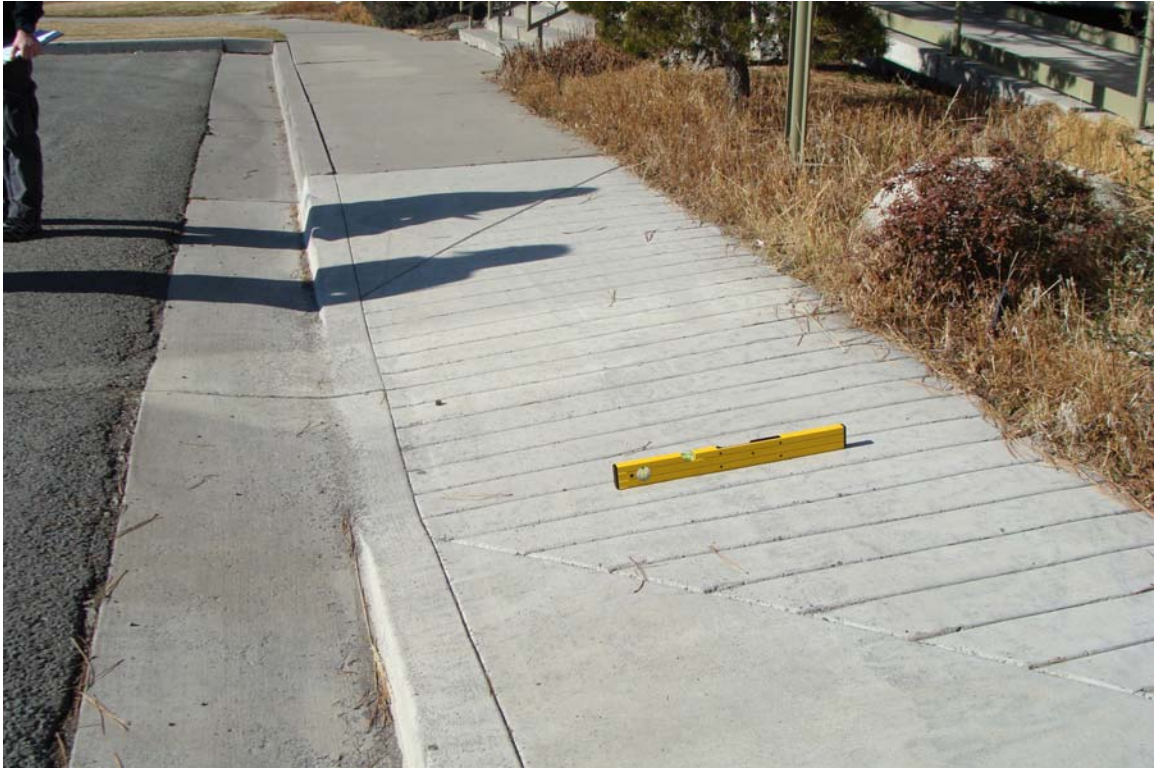
Nevada Historical Society - Building #0401 Description: ADA accessible route non compliant.
