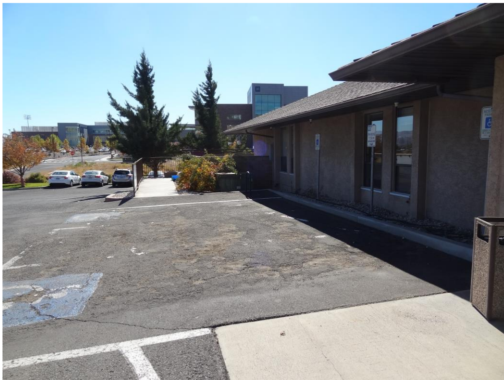
Nevada Early Intervention Services Site - Site #9859 Description: ADA Accessible Parking Upgrade Needed.
