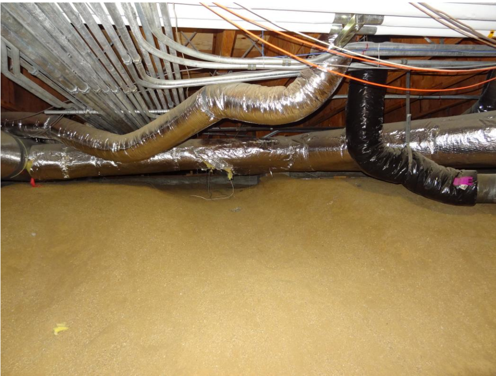
Nevada Early Intervention Services - Building #0515 Description: Fiberglass & Flex Replacement Needed.
