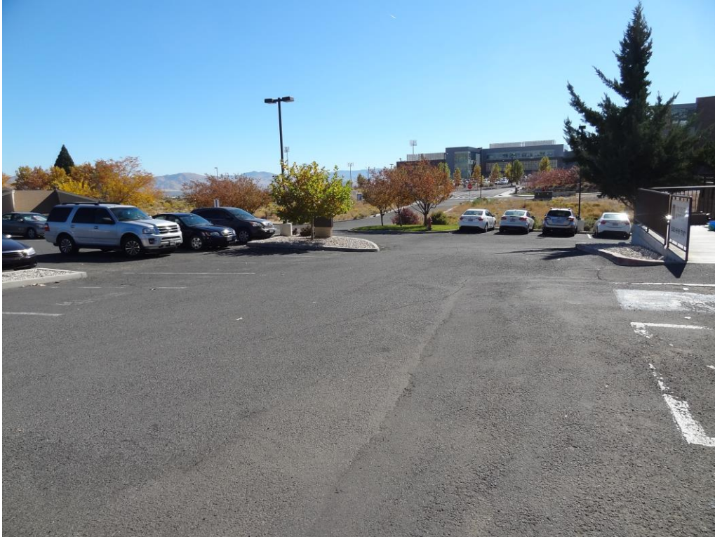
Nevada Early Intervention Services Site - Site #9859 Description: Slurry Seal & Striping Needed.
