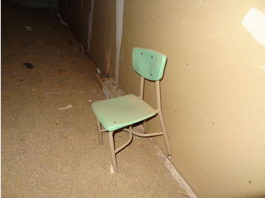
Nevada Early Intervention Services - Building #0515 Description: Regrade Crawlspace Needed .
