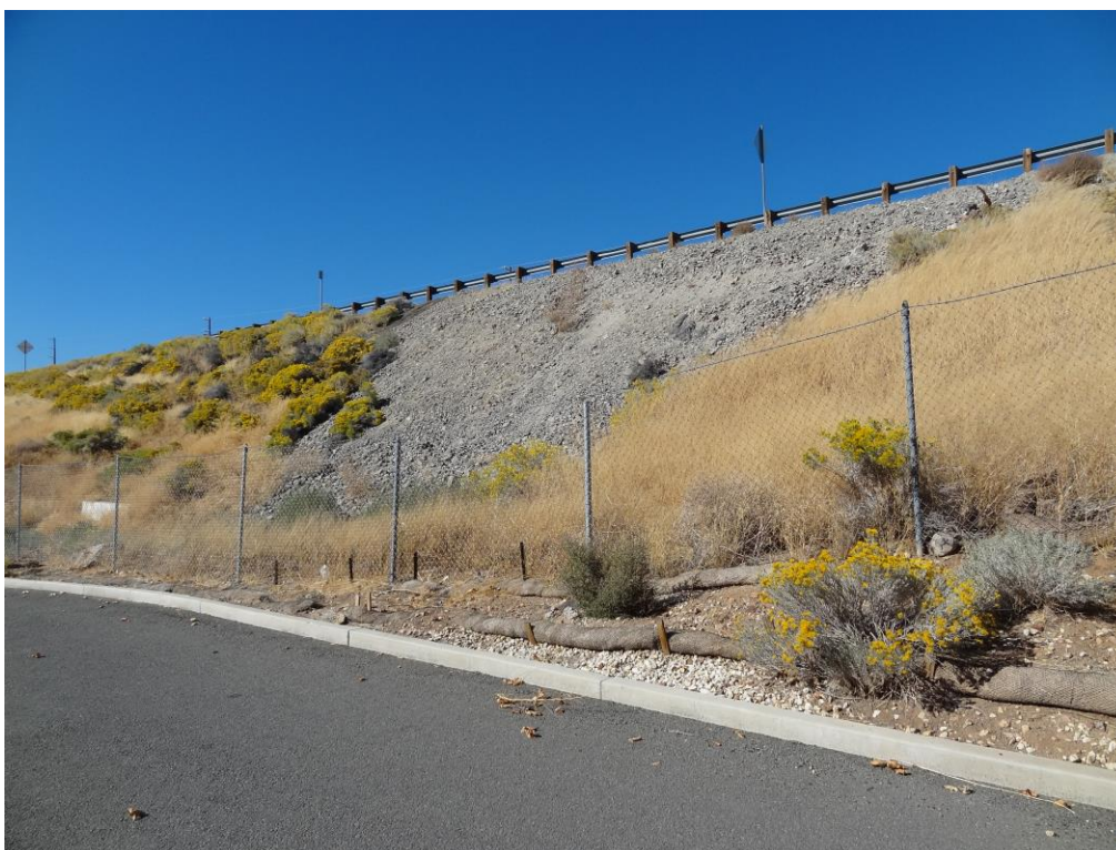
Nevada Early Intervention Services Site - Site #9859 Description: Additional Erosion Control Needed.
