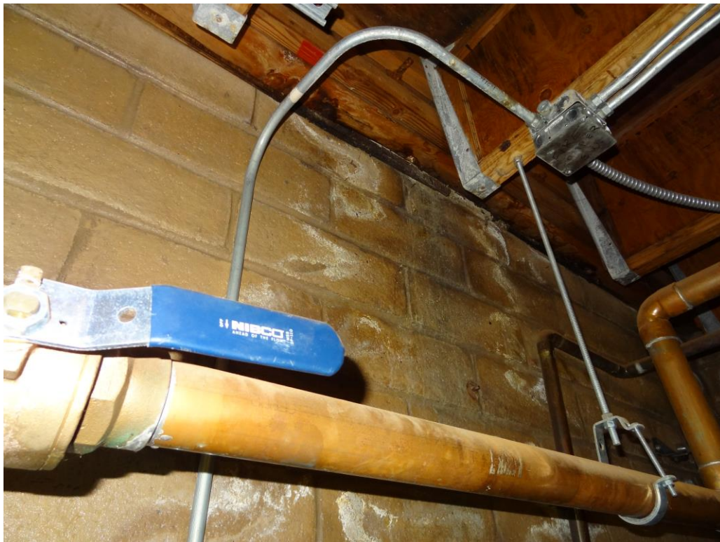
Nevada Early Intervention Services - Building #0515 Description: Evidence of Water Leaks – Waterproofing Upgrades.
