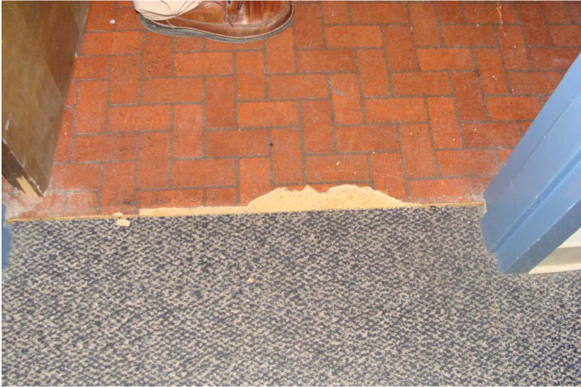
Nevada Early Intervention Services - Building #0515 Description: Typical worn flooring in original area of building.
