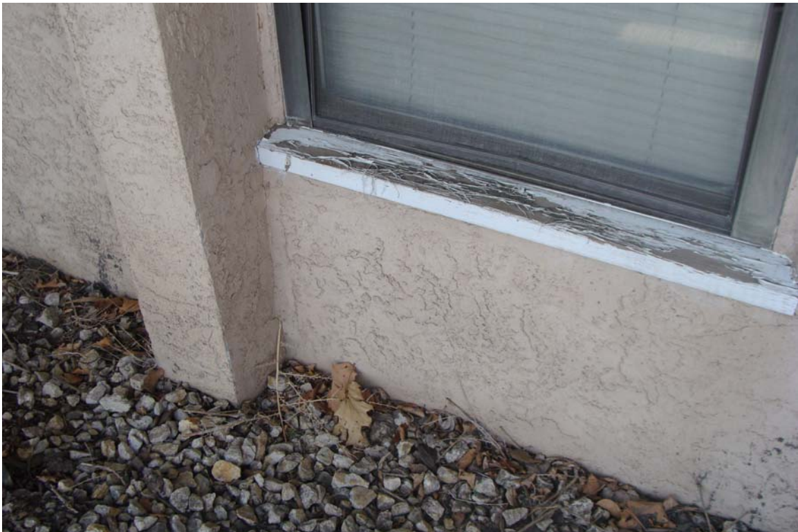
Nevada Early Intervention Services - Building #0515 Description: Window trim in need of paint.
