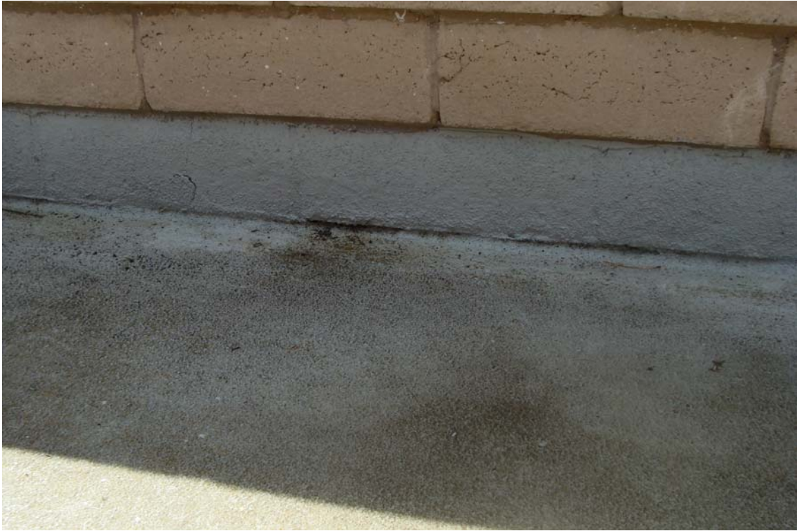
Nevada Early Intervention Services - Building #0515 Description: Area of possible water infiltration at exterior deck.
