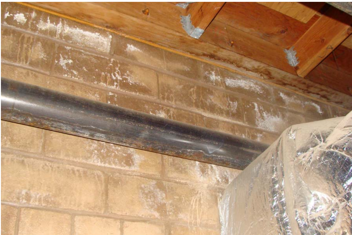
Nevada Early Intervention Services - Building #0515 Description: Evidence of water leaks.
