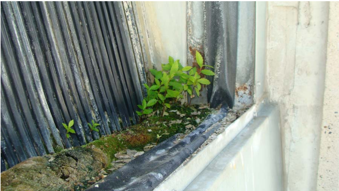
Blasdel Office Building - Building #0200 Description: Plant growth at cooling tower exhaust.
