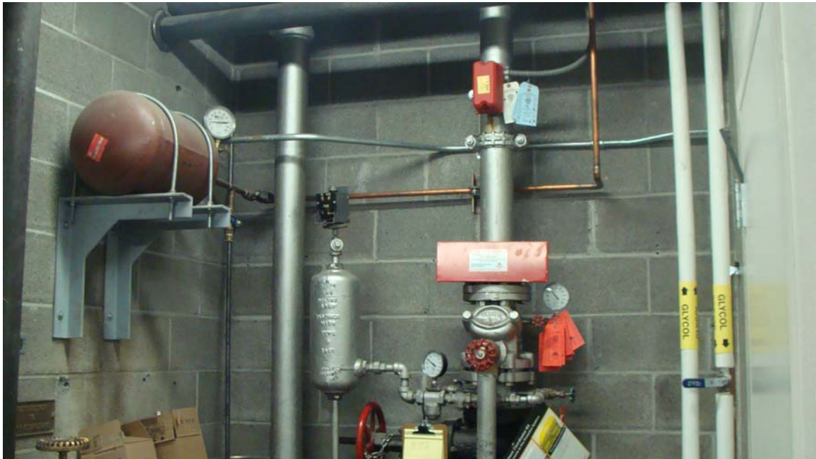
Blasdel Office Building - Building #0200 Description: Fire sprinkler riser in basement.
