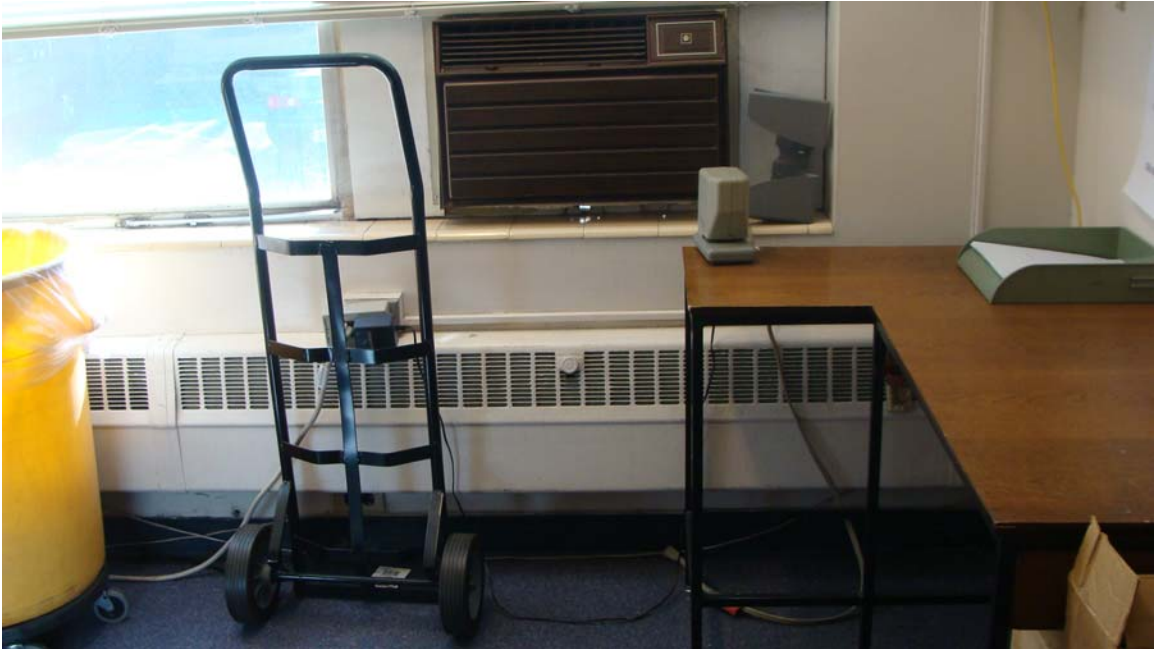
Blasdel Office Building - Building #0200 Description: Typical exterior wall mounted radiator.
