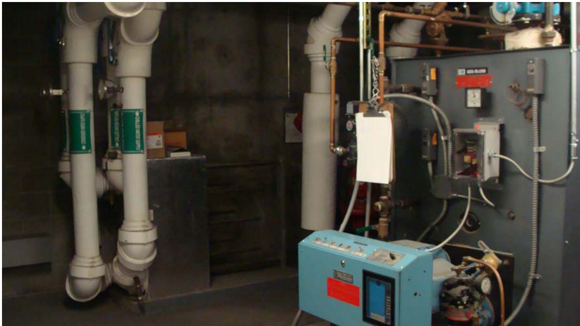
Blasdel Office Building - Building #0200 Description: Boiler in the basement Mechanical Room.
