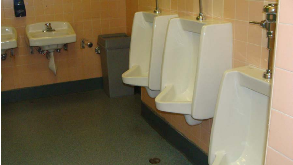
Blasdel Office Building - Building #0200 Description: Men's restroom in need of ADA upgrades.
