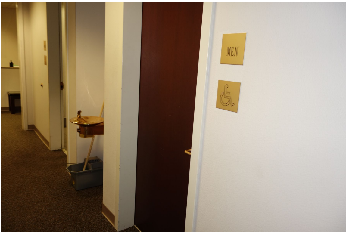
Supreme Court of Nevada - Building #1478 Description: ADA Signage Upgrade Needed.
