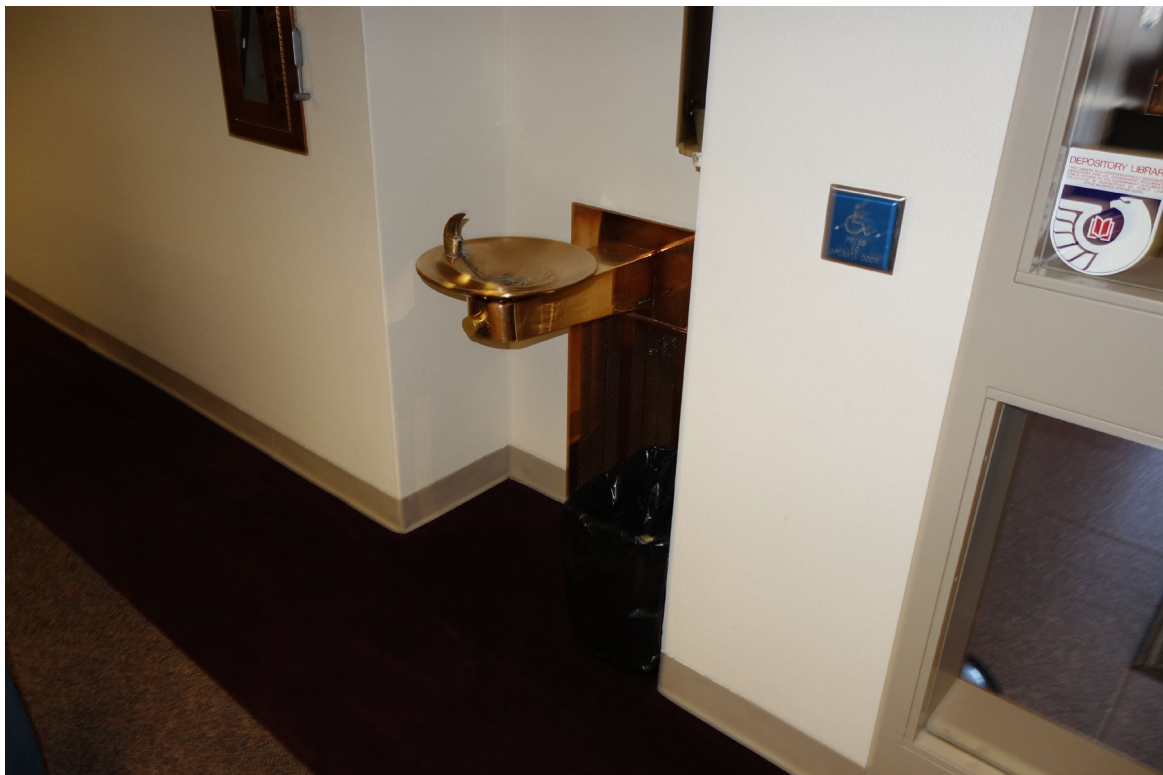
Supreme Court of Nevada - Building #1478 Description: Dual Level Drinking Fountains Needed.
