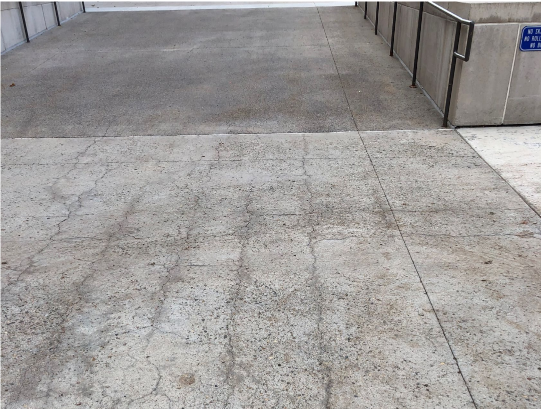
Supreme Court of Nevada - Site #9865 Description: Sidewalk Replacement Needed.
