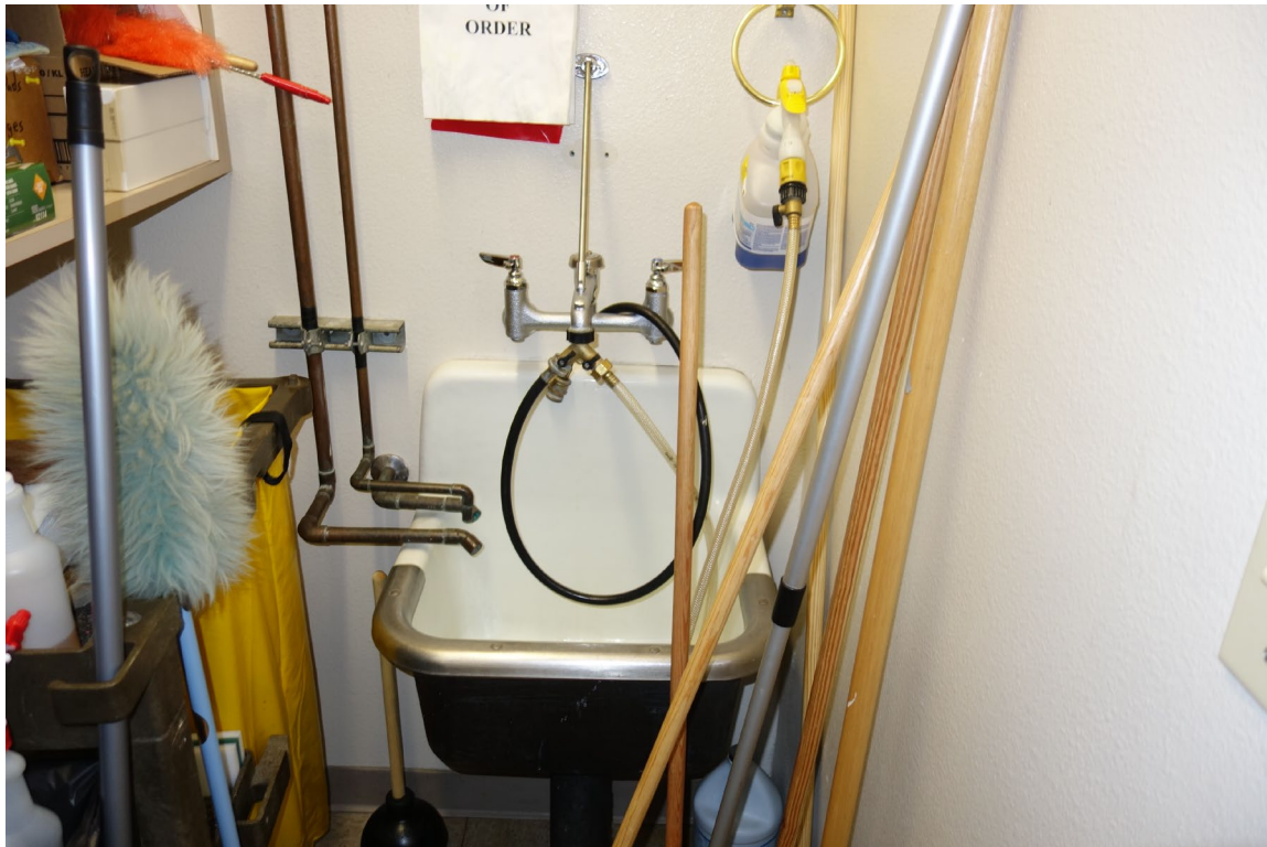
Supreme Court of Nevada - Building #1478 Description: Wall Protection at Janitor Sinks Needed.
