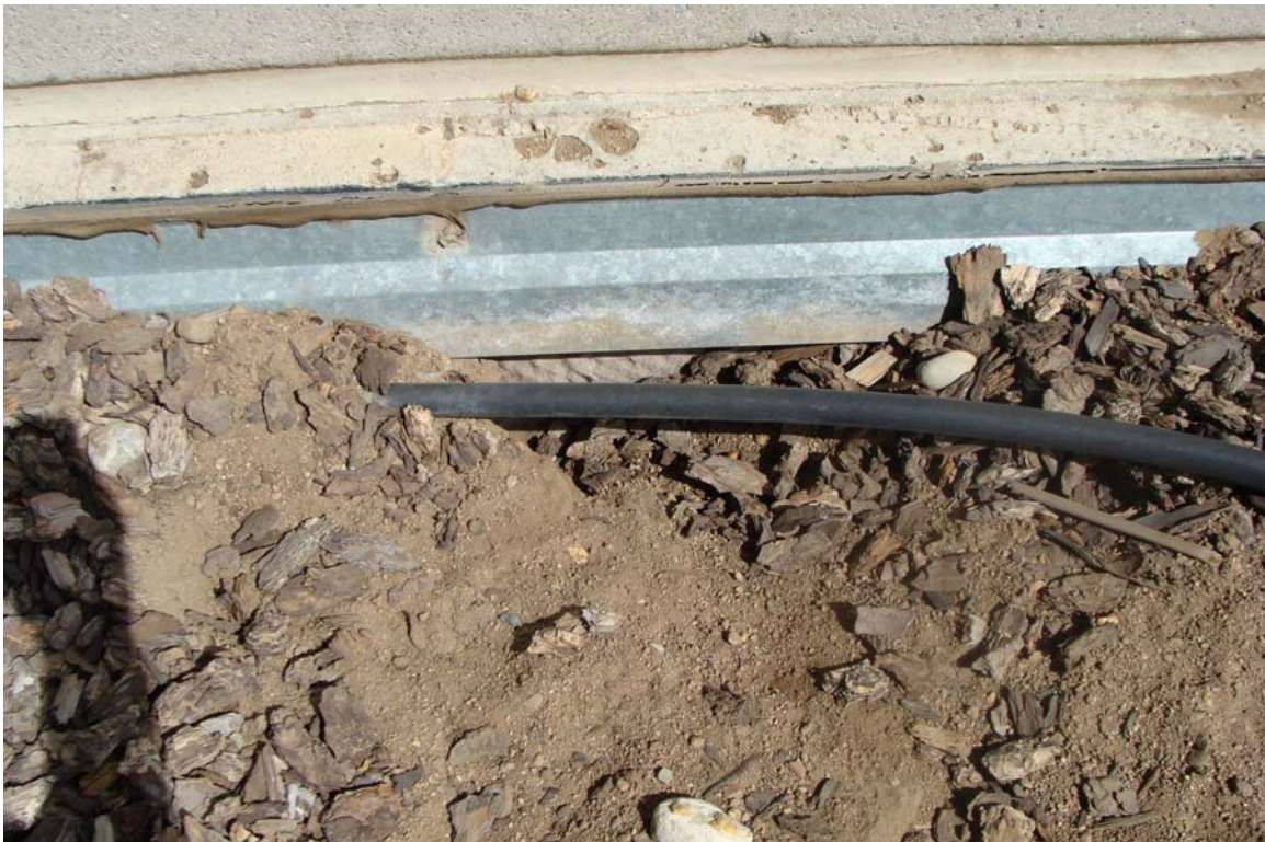
Supreme Court of Nevada - Building #1478 Description: Terrace planter in need of waterproof membrane repairs.
