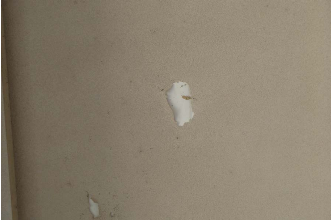
Supreme Court of Nevada - Building #1478 Description: Damage to EIFS at east entrance soffit.
