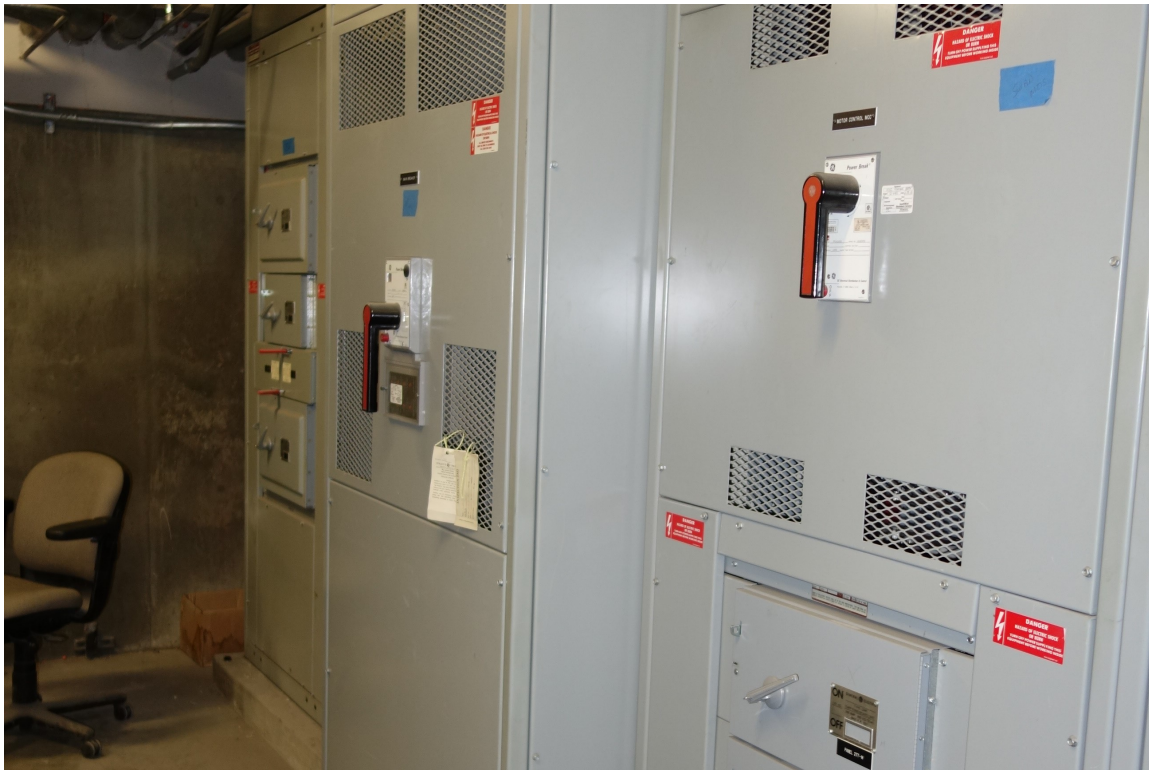
Supreme Court of Nevada - Building #1478 Description: Arc Flash & Breaker Coordination Needed.
