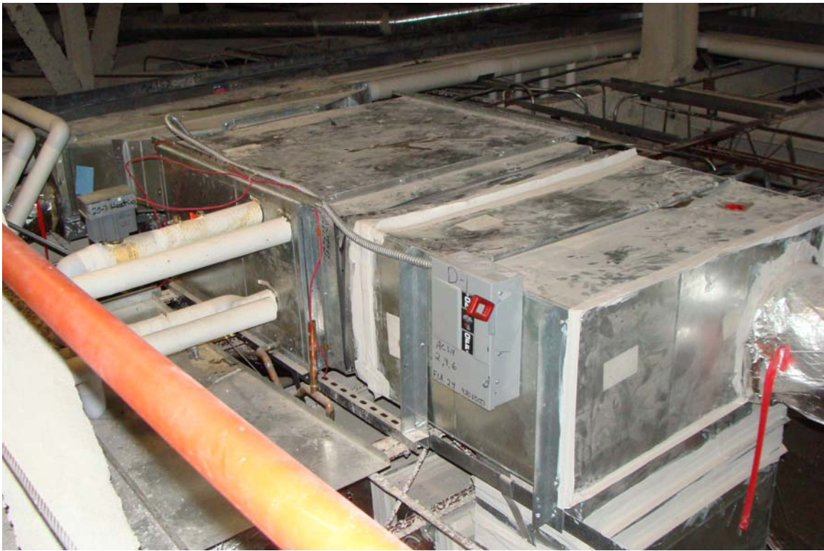
Supreme Court of Nevada - Building #1478 Description: Typical fan coil unit.
