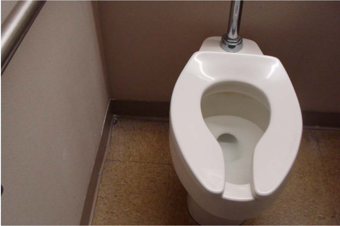
Supreme Court of Nevada - Building #1478 Description: Damaged VCT in restroom.
