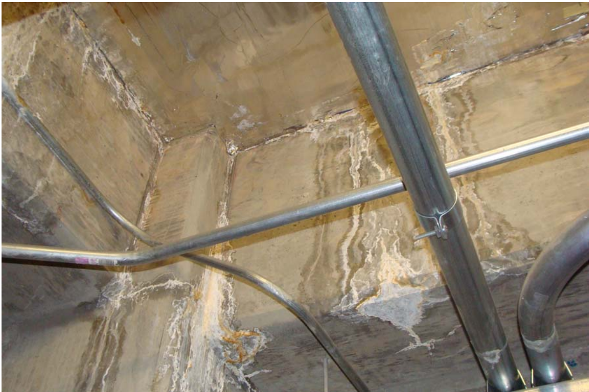
Supreme Court of Nevada - Building #1478 Description: Water infiltration in basement electrical switchgear room.
