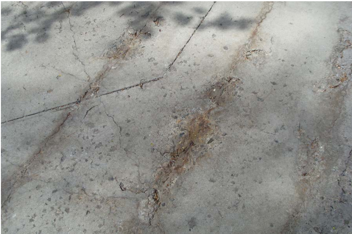
Supreme Court of Nevada - Building #1478 Description: Damaged walkway.
