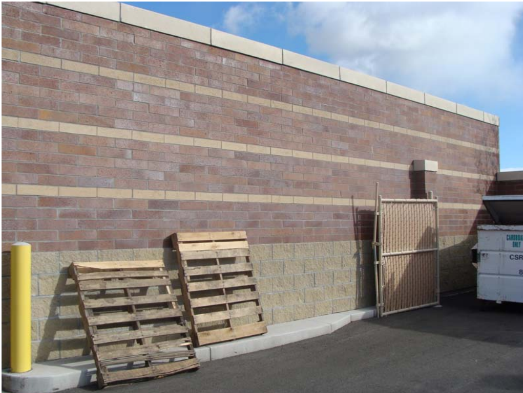
Richard H. Bryan Building - Building #2450 Description: Generator enclosure structure.
