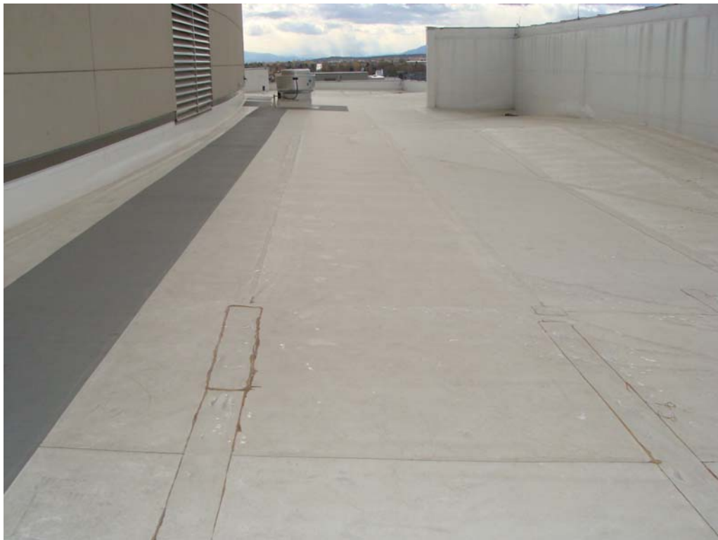
Richard H. Bryan Building - Building #2450 Description: Area of roof where ballooning is occurring during wind events.
