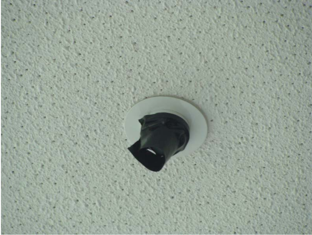
Richard H. Bryan Building - Building #2450 Description: Altered lighting sensor.
