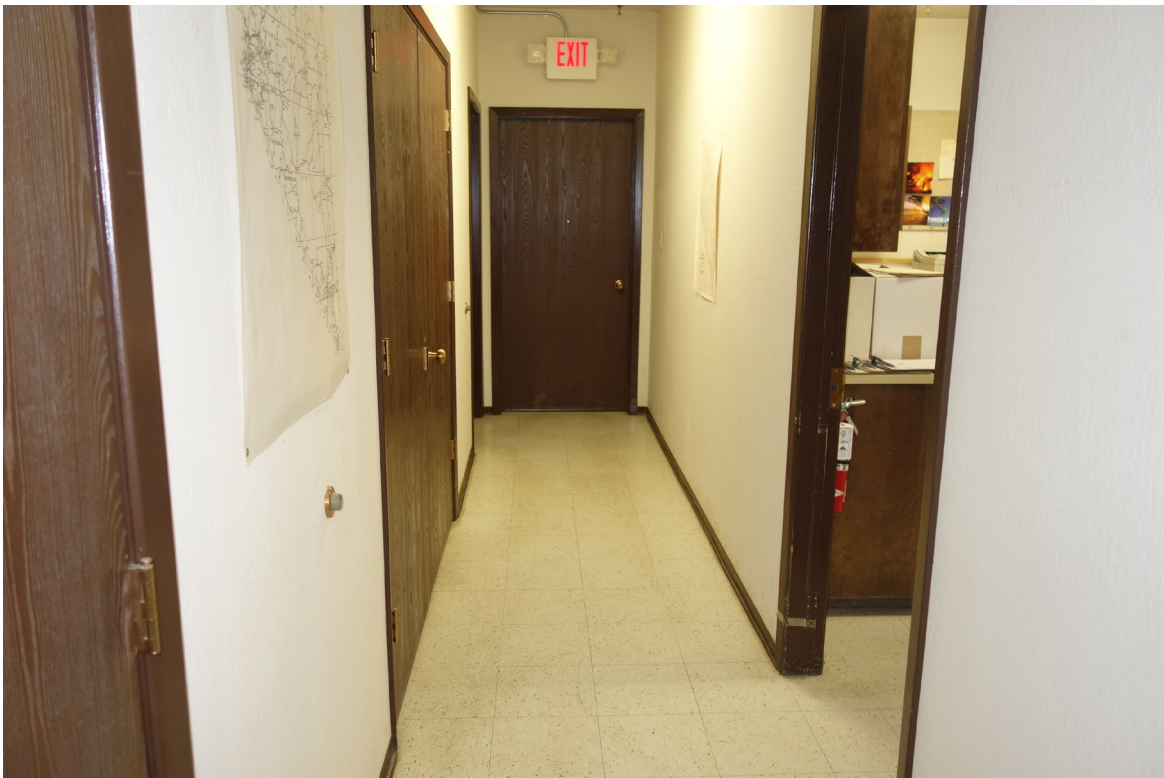
Indian Hills Warehouse – FCA Building #0860 Description: Accessible Door Hardware Needed
