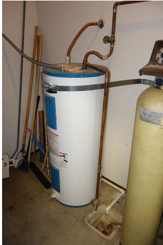
Indian Hills Warehouse – FCA Building #0860 Description: Water Heater Replacement Needed.
