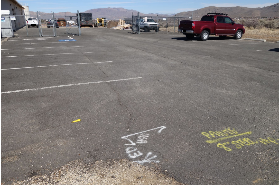
Nevada State Museum Indian Hills Site – FCA Site #9874 Description: Asphalt Crack Fill & Slurry Seal Recommended.
