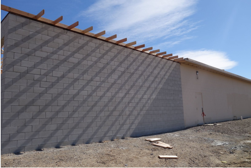
Indian Hills Warehouse – FCA Building #0860 Description: Exterior Insulation & Finish System (EIFS) Needed.
