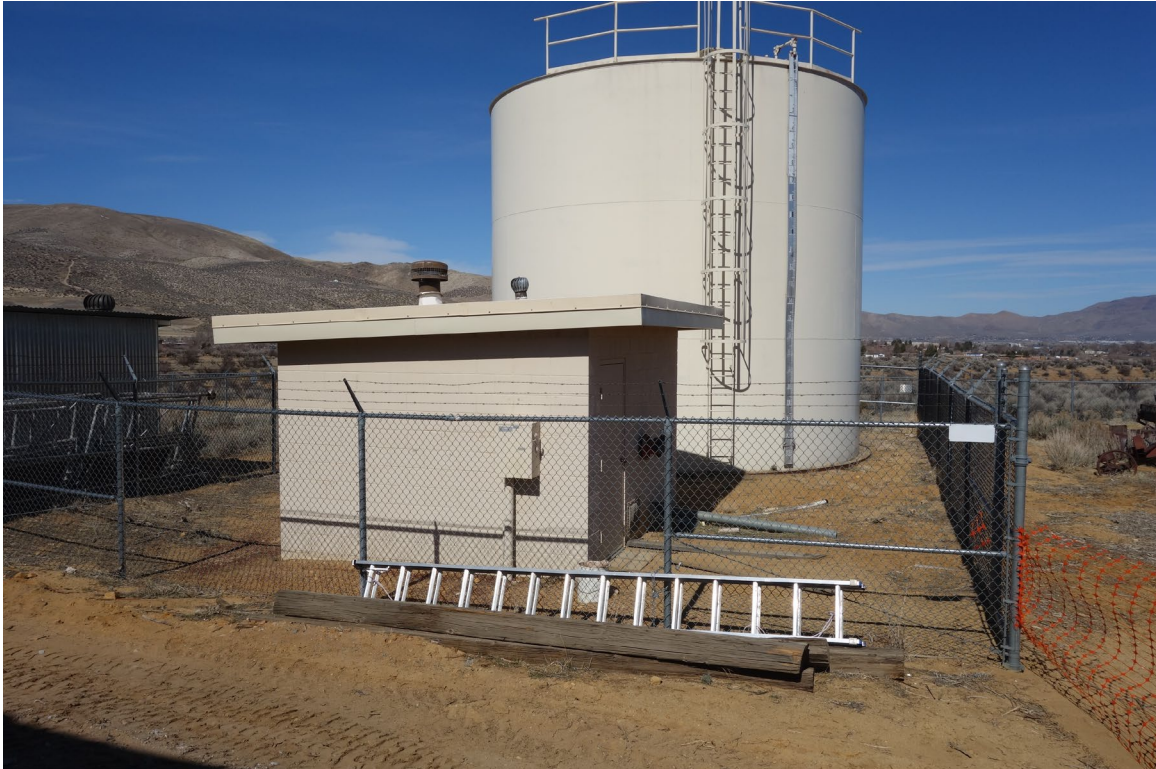
Indian Hills Water Tower – FCA Building #2563 Description: Exterior of the Water Storage Tank.
