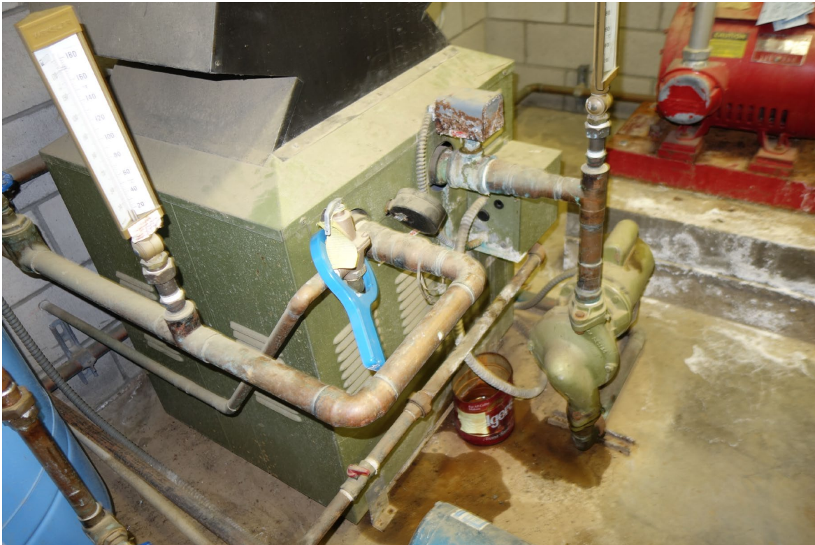
Indian Hills Pump House – FCA Building #0859 Description: Abandoned Boiler Removal Needed.
